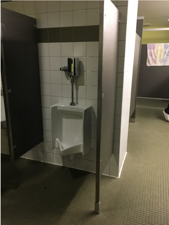
TEAM ROOM: RESTROOM
