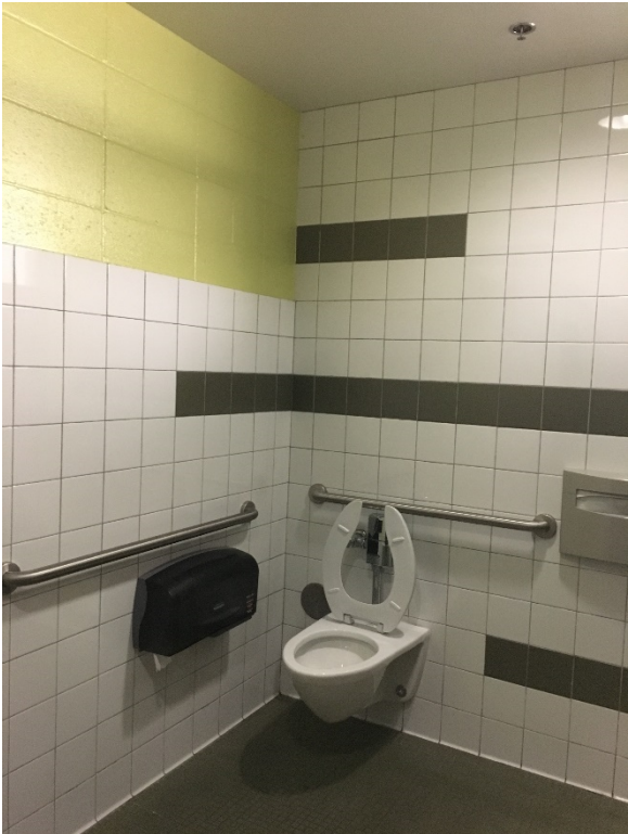
TEAM ROOM: RESTROOM
