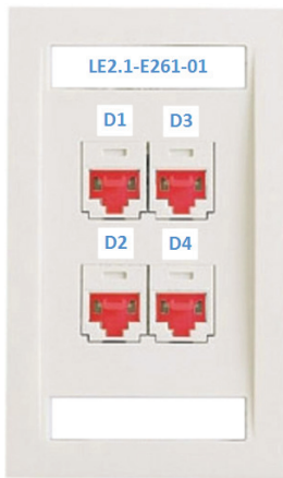
Incorrect Faceplate Labeling
