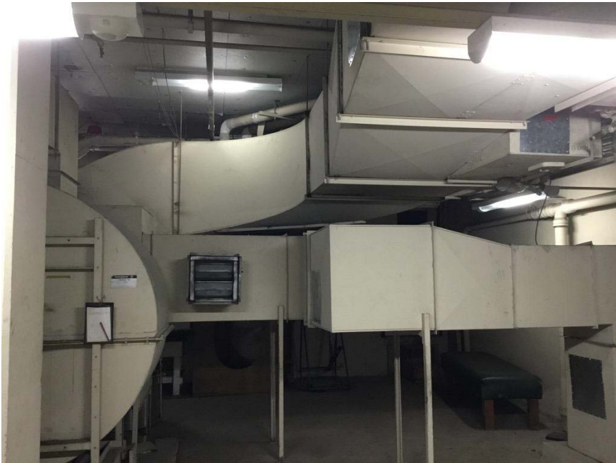
Photograph 11: View depicting the mechanical room.
