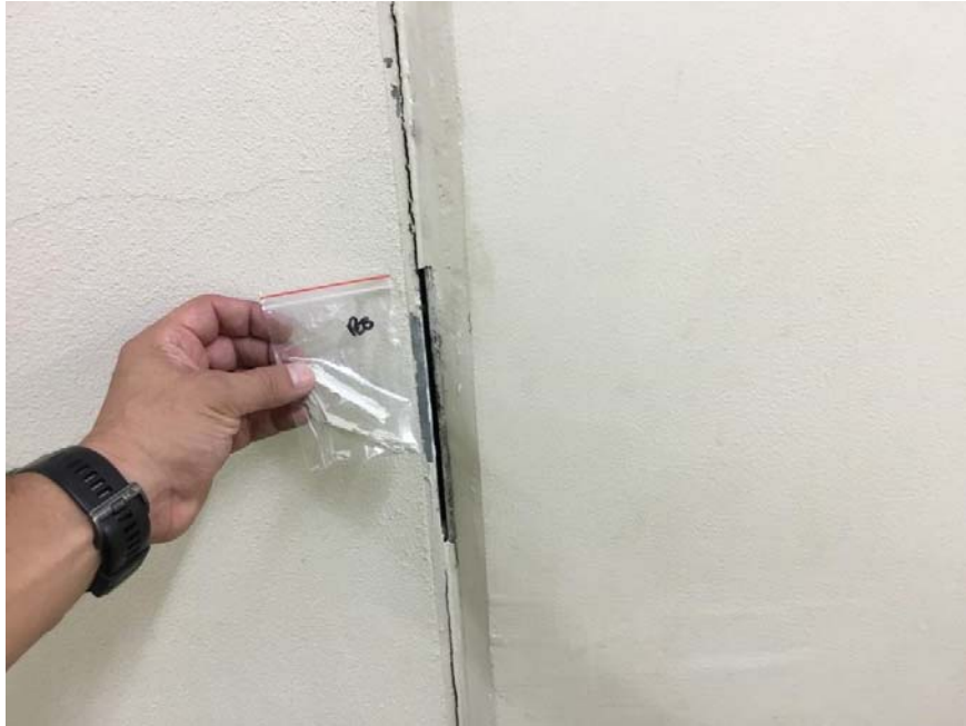
Photograph 9: View depicting the concrete caulking material located in the mechanical room hallway that contains trace amounts of PCBs.
