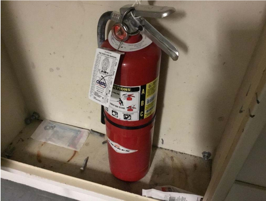
Photograph 13: View depicting a typical fire extinguisher located in the men’s locker room.
