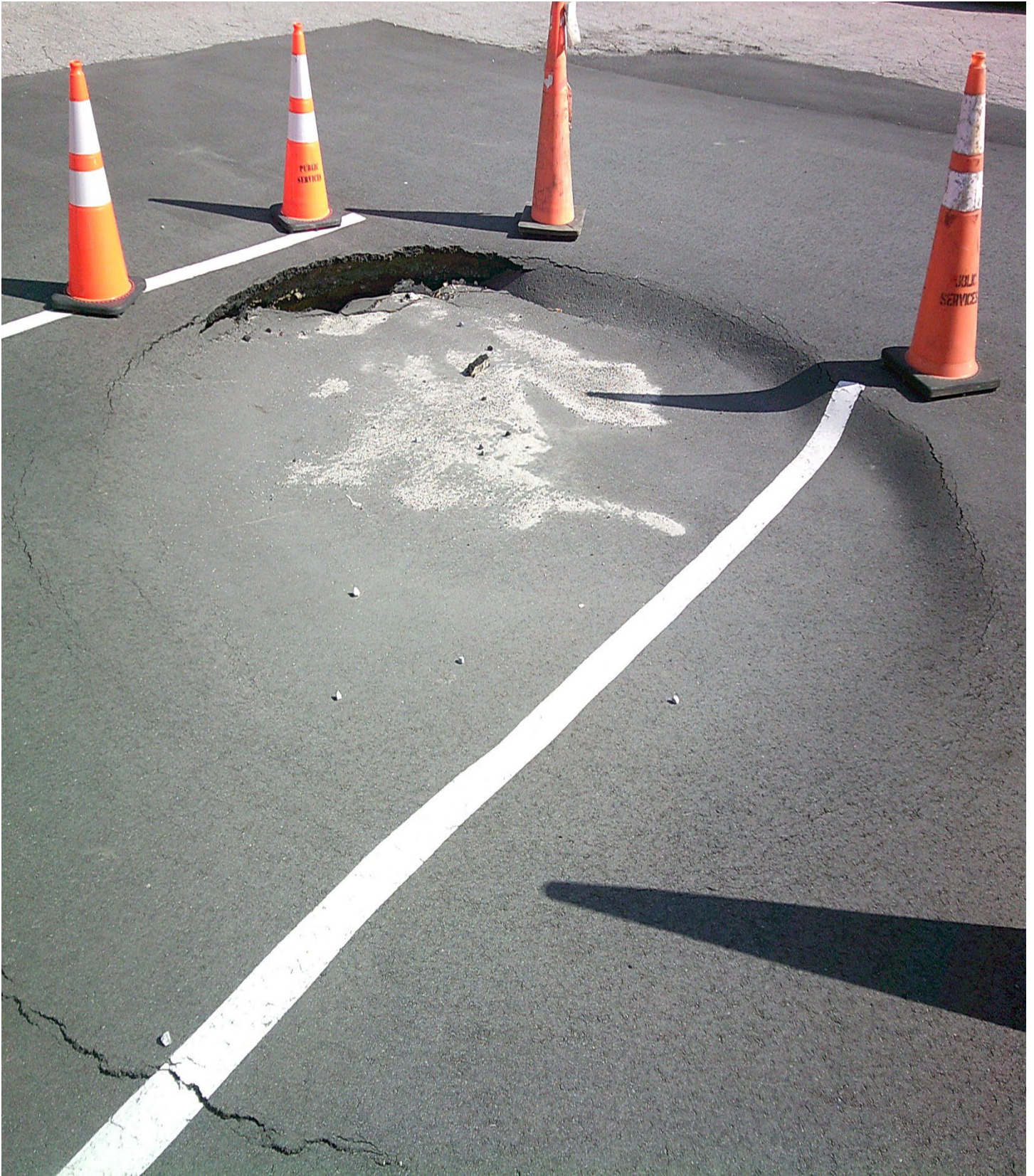
Figure 4: Image of the Sink Hole
