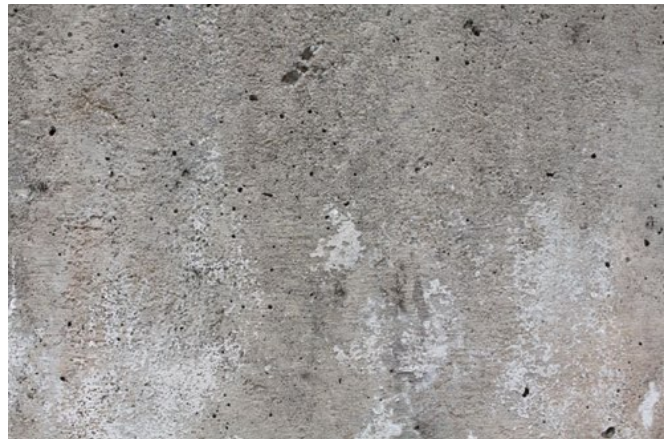
Example concrete surface showing blow holes and imperfections from form liner.
