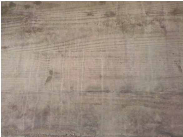
Example concrete surface showing grain from plywood form.
