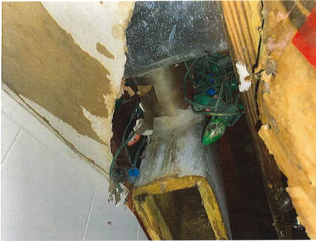
Asbestos Containing (5-6% C) Duct Mastic (Gray), Above Ceiling Office Building
