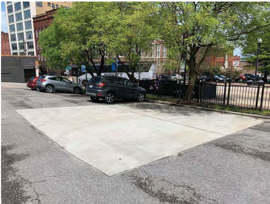
Photograph 4: Concrete-paved area along east property boundary where area of subsidence was repaired
