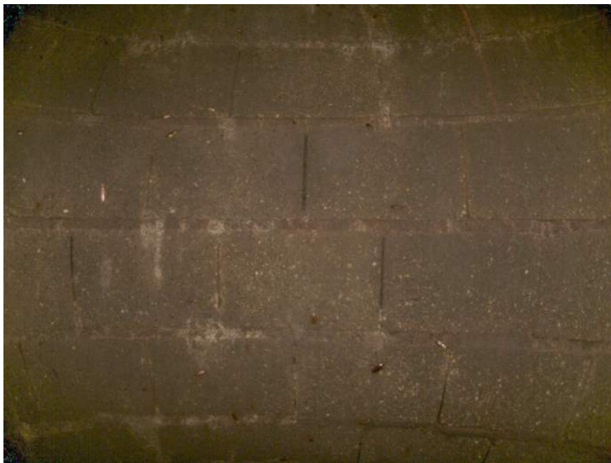
1841a_7e3e94ed-5602-4c81-88a8-bfb0bb428782_0c78dd5f-e3c7-4c72-9611-2f16527626f1_P11.jpg, 00:00:42, 9.84 Surface Damage Aggregate Visible from 12 o'clock to 12 o'clock, within 8 inch
