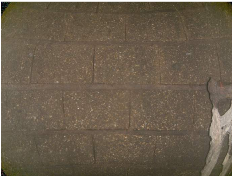
1838_4d464b94-a957-4557-a7ae-8bb14bf4d783_5c5b9007-ca65-4280-add5-f176f9132037_P11.jpg, 00:00:28, 6.15 Missing Mortar Large from 12 o'clock to 12 o'clock
