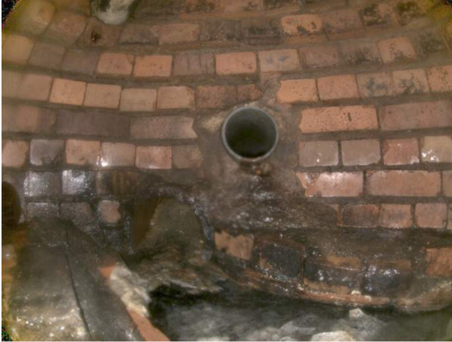
2193c_2b27c63e-1844-43c6-8c49-44849fa40c9a_db133c1a-727c-427a-9ae2-24e83ae66ad0_P11.jpg, 00:00:17, 3.42 Infiltration Weeper from 4 o'clock to 11 o'clock, within 8 inch
