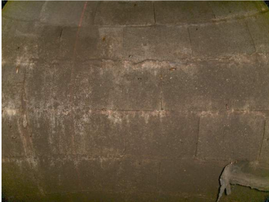
1841a_7e3e94ed-5602-4c81-88a8-bfb0bb428782_51c81039-b210-414f-a942-c3150f368998_P11.jpg, 00:00:33, 7.62 Missing Mortar Large from 12 o'clock to 12 o'clock
