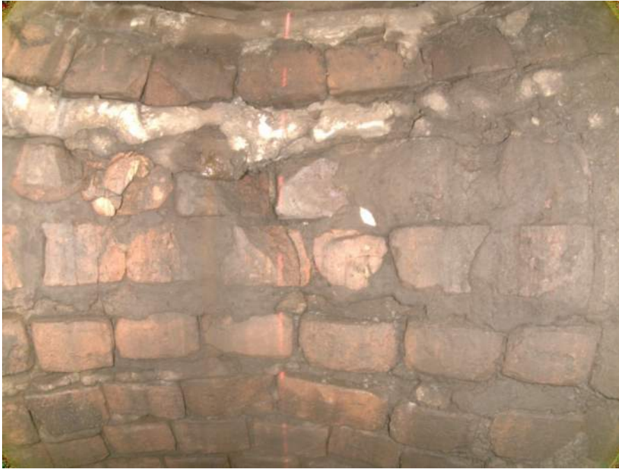
1829b_c3bb5419-4fc2-49bd-9cbb-ae8a522c6251_3b097954-56f3-4b33-9fc7-c80c508f7421_P11.jpg, 1.28 Infiltration Weeper from 6 o'clock to 7 o'clock, within 8 inch
