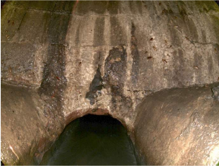
1839_f7a2e778-f07c-460d-8979-384ad1d2d1b3_f0b0d505-39c7-45cf-a092-b070cc688200_PI1.jpg, 00:00:43, 9.11 Infiltration Weeper Connection from 5 o'clock to 7 o'clock, within 8 inch
