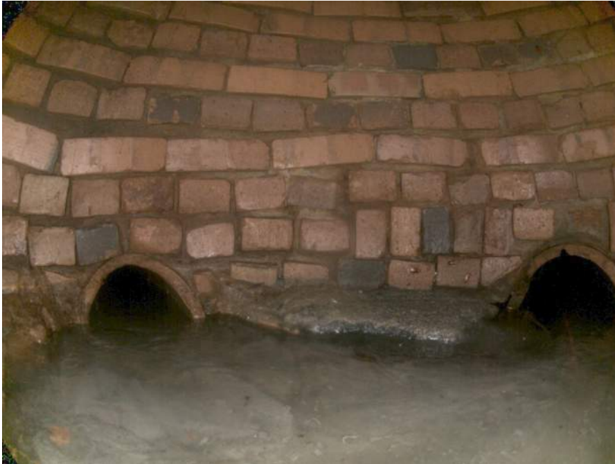
1832_5c717e28-5342-43ea-a091-aed22e190ee5_5c9301a7-40d7-4e29-bed0-567614a4fd1c_P11.jpg, 00:00:00, 7.68 Missing Mortar Medium from 12 o'clock to 12 o'clock
