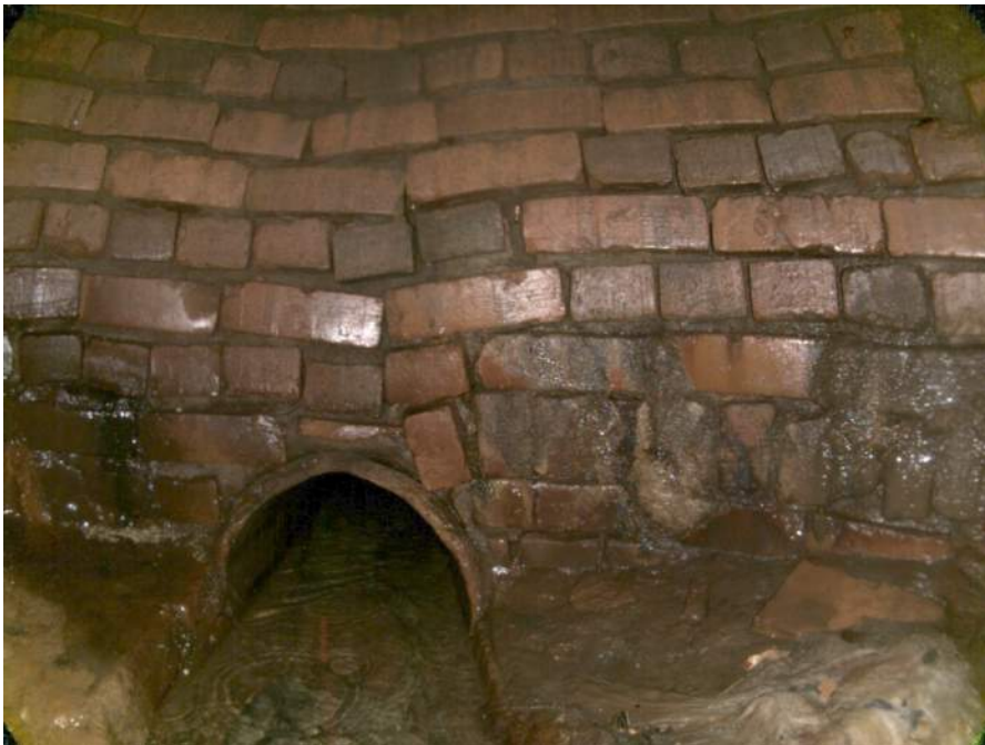
1830_f8e692ed-45a5-4111-be6d-dbb6437dd8b2_e7ceb1d1-5301-4ee2-b6a3-deb392ea1197_P11.jpg, 00:00:38, 7.93 Displaced Brick from 5 o'clock to 7 o'clock
