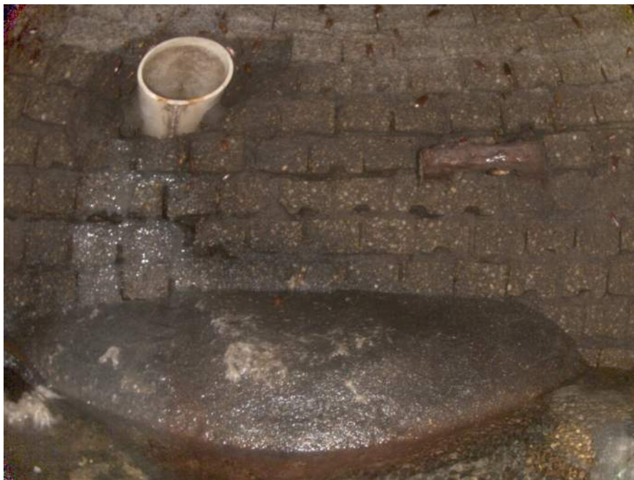
1823d_c2435bdb-6471-4a3b-8f5b-2755123d82bf_7b3163da-1179-4d08-8a3e-afb833ffb71f_P11.jpg, 00:00:15, 4.37 Deposits Settled Gravel, 15% of cross sectional area from 8 o'clock to 12 o'clock, within 8 inch
