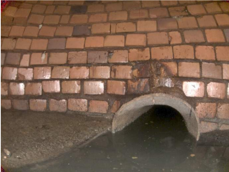
1818_a75925b2-5868-48ca-b1fe-f6e0ecc4562_e8967312-3d74-46f8-a9cd-e2c4d6f5cb14_P11.jpg, 00:00:35, 8.12 Infiltration Weeper from 5 o'clock to 7 o'clock, within 8 inch
