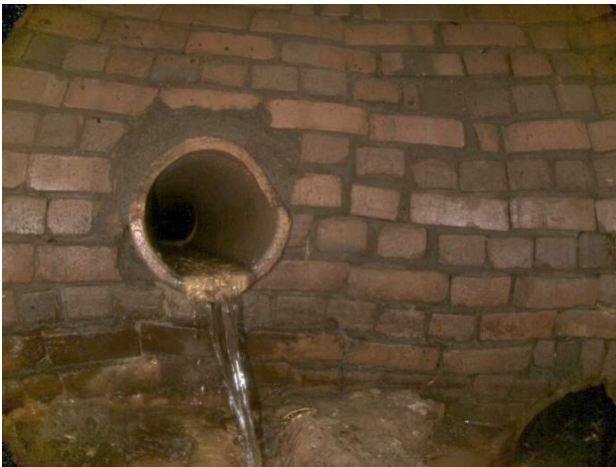
1834b_16edcb0d-7f2c-4b5a-bd27-6b0d1bf9d1bd_b33f93a0-66d3-4a68-be57-658e110c837b_P11.jpg, 00:00:29, 6.90 Missing Mortar Large from 12 o'clock to 12 o'clock
