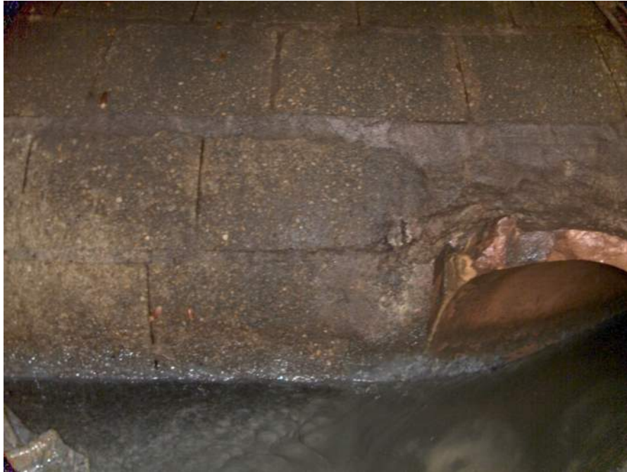
1842_98b1de5e-0e50-41ed-b476-ff581fdb636e_bb003c6b-c5eb-4aa5-a173-ba34dc52eeb9_PI1.jpg, 00:00:42, 8.72 Infiltration Weeper from 10 o'clock to 12 o'clock, within 8 inch
