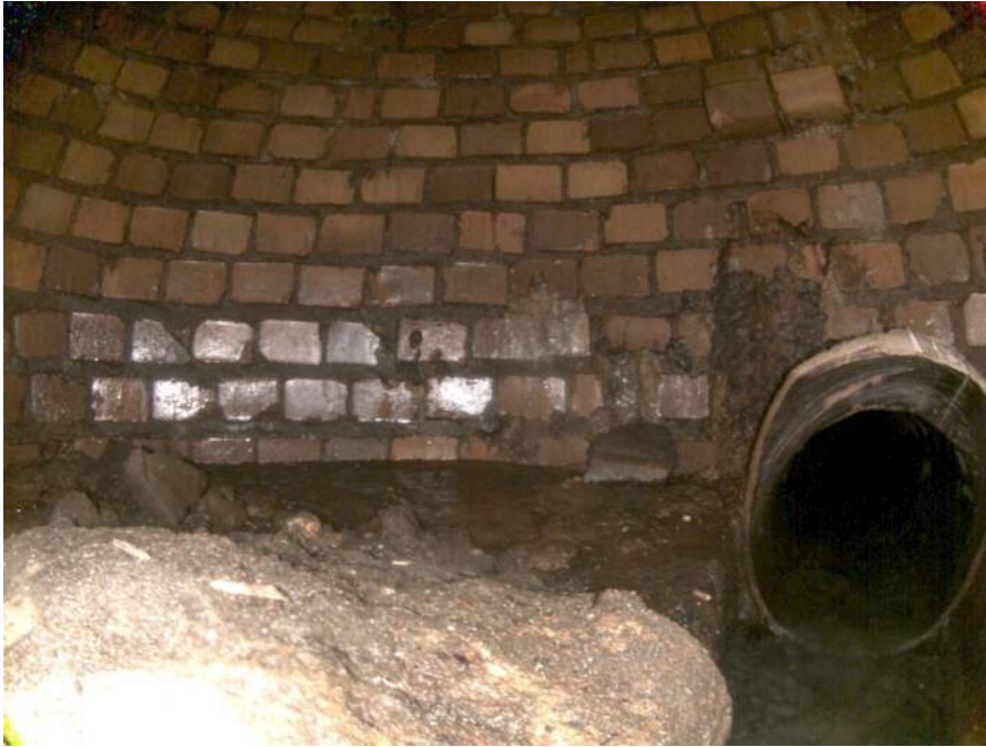
1819_3d72062a-4862-48ce-be8e-7bbe04d95bb2_bdad6f71-750a-47c5-9c9e-cf68ca13fd8e_P11.jpg, 00:00:36, 8.57 Deposits Settled Other, 35% of cross sectional area from 9 o'clock to 3 o'clock, within 8 inch
