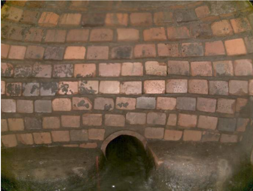
2194_1962243a-d72d-4c62-9e3a-2c87a26c1c57_382482e7-71a6-48b7-908e-3d8be0875e4c_P11.jpg, 00:00:19, 3.16 Missing Mortar Large from 12 o'clock to 12 o'clock
