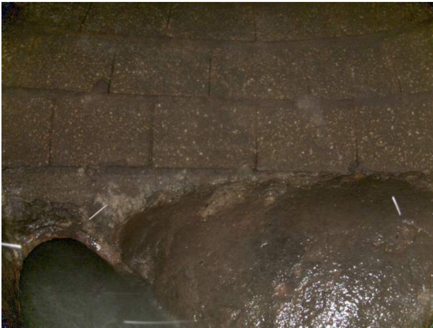
1837c_166883a2-6c9f-44dc-8d3b-993be20f6dc6_8f20deb1-cfa1-4303-84b8-4d47adbe017c_P11.jpg, 00:00:37, 8.51 Infiltration Weeper from 1 o'clock to 5 o'clock, within 8 inch
