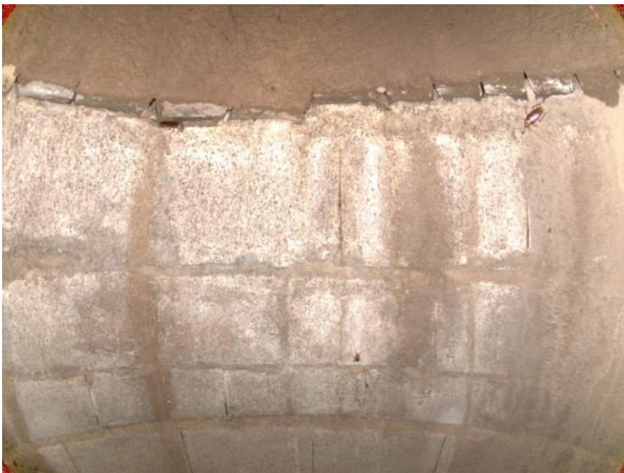
1841a_7e3e94ed-5602-4c81-88a8-bfb0bb428782_49b19cba-c025-49c9-8b0e-801e87cd9422_PL11.jpg, 00:00:13, 2.38 Missing Mortar Large from 12 o'clock to 11 o'clock, Start
