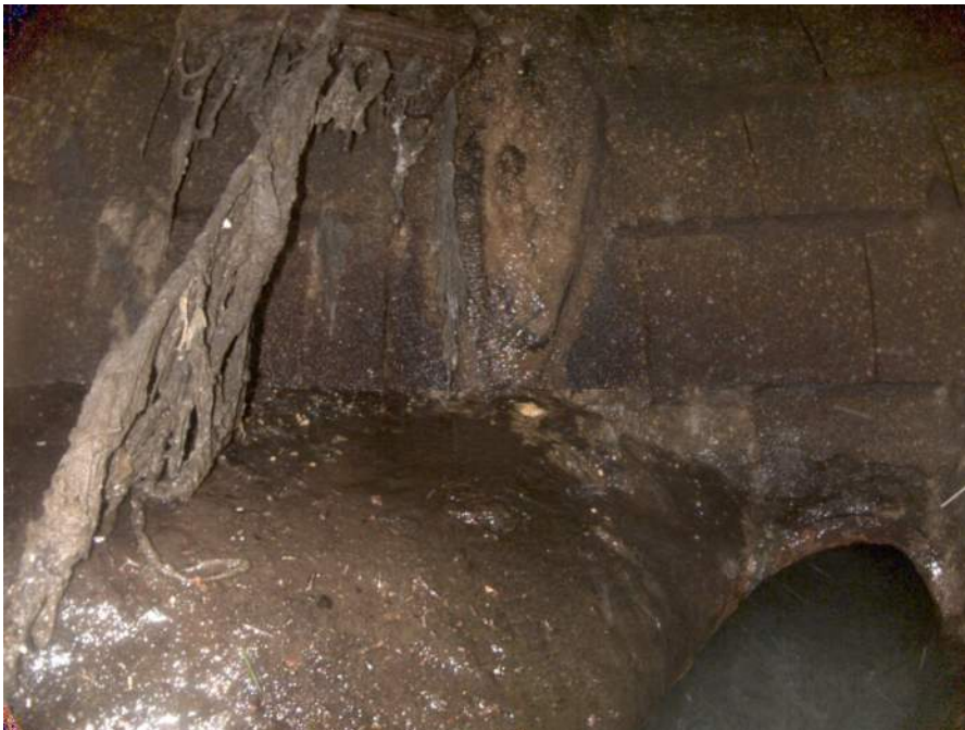
1837c_166883a2-6c9f-44dc-8d3b-993be20f6dc6_531288a5-3195-4292-88f6-c4597b920581_P11.jpg, 00:00:37, 8.90 Infiltration Weeper from 11 o'clock to 1 o'clock, within 8 inch
