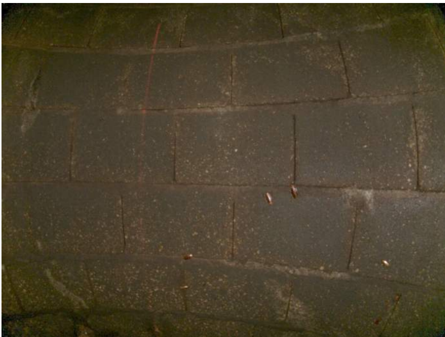
1842_98b1de5e-0e50-41ed-b476-ff581fdb636e_dcbefd8a-b7e6-401c-9a30-5acdf49e2291_PI1.jpg, 00:00:33, 6.73 Missing Mortar Large from 12 o'clock to 12 o'clock
