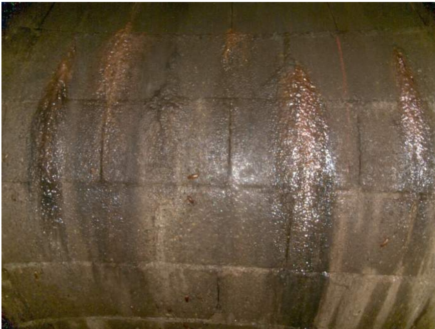
1839_f7a2e778-f07c-460d-8979-384ad1d2d1b3_28c88a54-ab87-4373-9285-fc74b2411704_PI1.jpg, 00:00:33, 6.76 Missing Mortar Large from 12 o'clock to 12 o'clock
