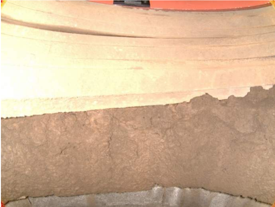
1841a_7e3e94ed-5602-4c81-88a8-bfb0bb428782_5ec9646d-4da9-4be7-a8c7-3f5e4dbdd8f5_PL11.jpg, 00:00:08, 1.01 Missing Mortar Small from 1 o'clock to 6 o'clock
