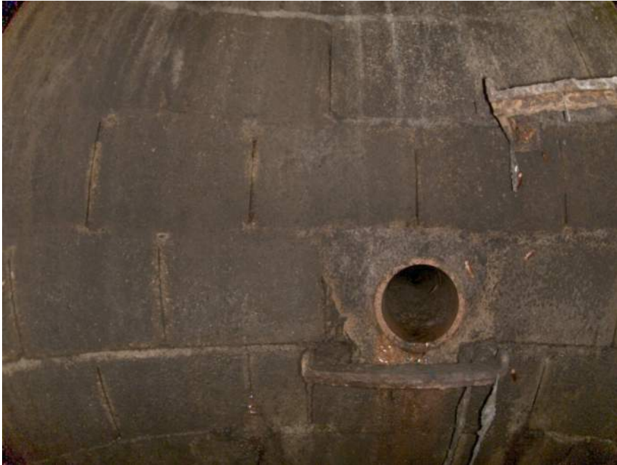
1839_f7a2e778-f07c-460d-8979-384ad1d2d1b3_26e11d77-b5b6-47cb-ba13-ce6b8078be20_P11.jpg, 00:00:22, 4.10 Deposits Attached Ragging, 5% of cross sectional area from 8 o'clock to 12 o'clock, within 8 inch
