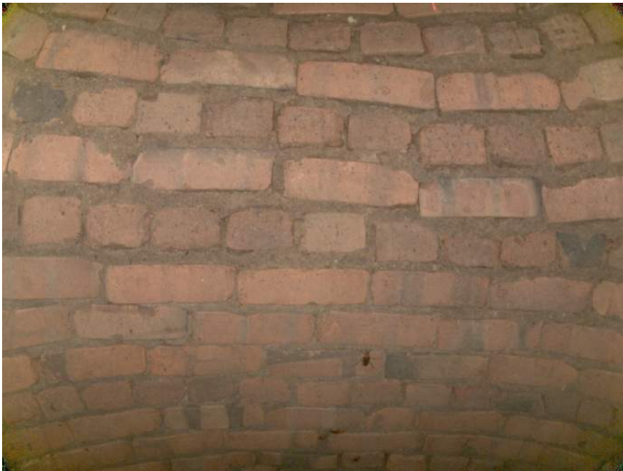
1834b_16edcb0d-7f2c-4b5a-bd27-6b0d1bf9d1bd_858fbed5-5e08-48eb-856e-6c910e6eeb07_P11.jpg, 00:00:18, 4.00 Missing Mortar Large from 12 o'clock to 12 o'clock
