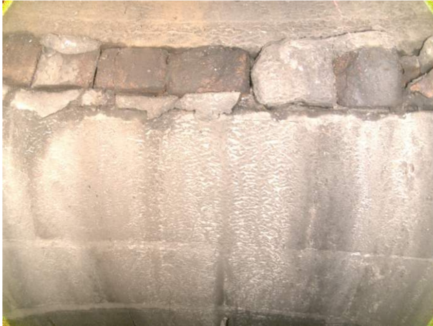
1837c_166883a2-6c9f-44dc-8d3b-993be20f6dc6_657e633f-e4e6-4faa-a090-0da65f01be06_P11.jpg, 00:00:09, 1.12 Infiltration Stain from 12 o'clock to 12 o'clock, within 8 inch
