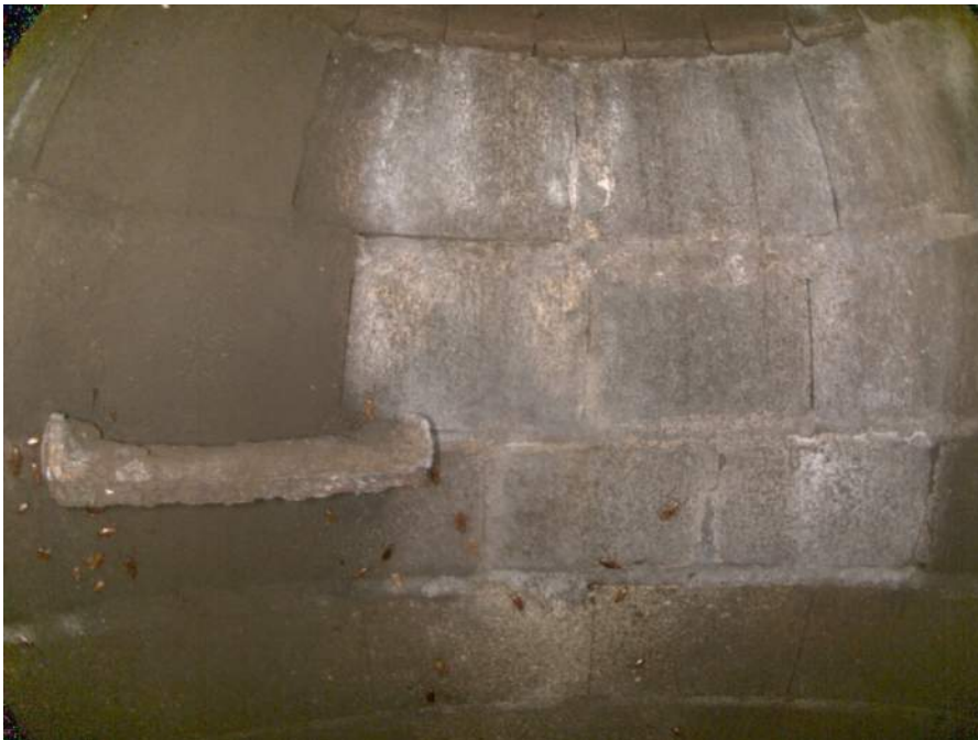
1840b_b7eec4bd-8b4a-4779-9657-5106bc04b13d_ebc59ab5-135d-41b7-a25a-f94a7cc157d3_P11.jpg, , 3.05 Infiltration Stain from 9 o'clock to 2 o'clock, within 8 inch
