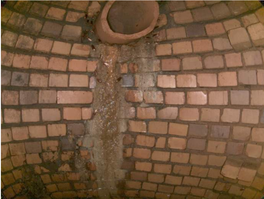
1818_a75925b2-5868-48ca-b1fe-f6e00ecc4562_5ad39124-75a8-4790-880a-2cad4d512614_P11.jpg, 00:00:27, 6.17 Infiltration Dripper from 12 o'clock to 2 o'clock, within 8 inch
