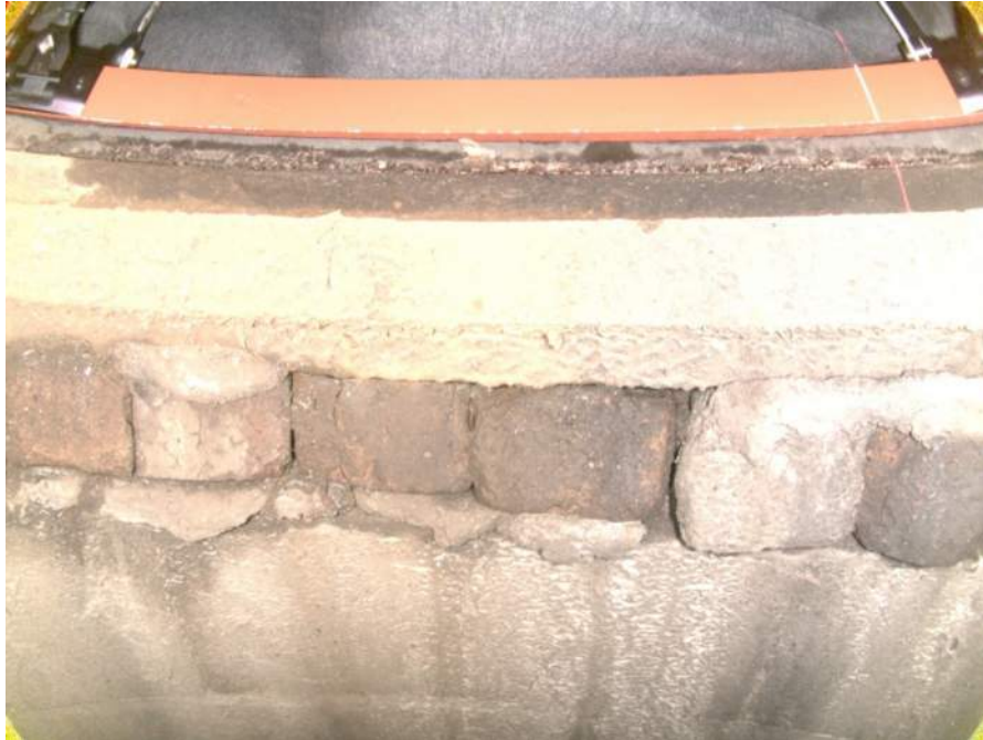
1837c_166883a2-6c9f-44dc-8d3b-993be20f6dc6_49d81684-3099-4e55-92f5-afd22f980810_P11.jpg, 00:00:07, 0.58 Missing Mortar Large from 12 o'clock to 12 o'clock
