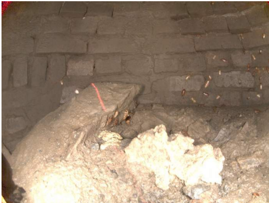
1821_b79fd861-dd10-4846-a6c3-82d3d499c9c7_0bc5d1de-e242-4391-b787-4bef6b28f7b0_PI1.jpg, 00:00:17, 3.83 Obstruction Construction Debris, 35% of cross sectional area from 12 o'clock to 12 o'clock
