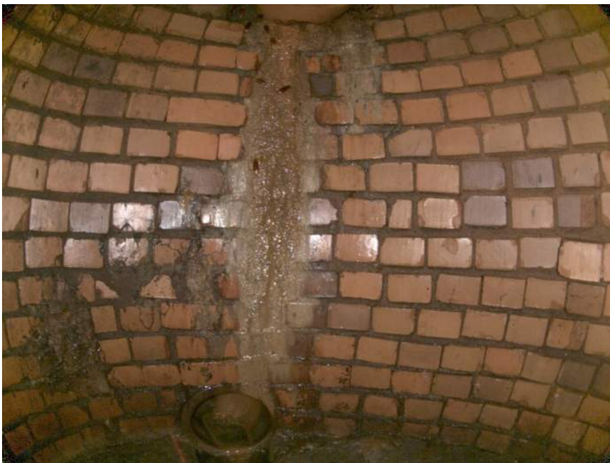
1818_a75925b2-5868-48ca-b1fe-f6e00ecc4562_dd159dc7-5399-49fc-888f-b48a01663db8_P11.jpg, 00:00:31, 7.17 Missing Mortar Large from 12 o'clock to 12 o'clock
