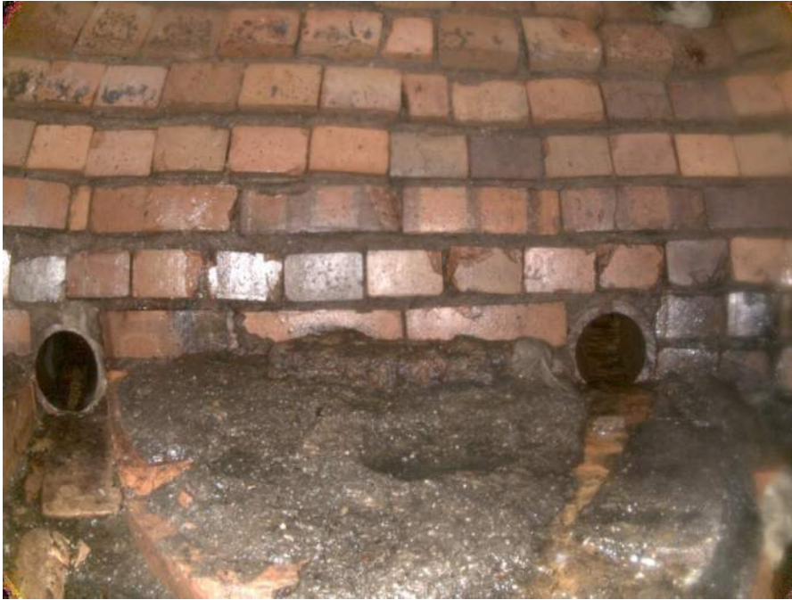
2193c_2b27c63e-1844-43c6-8c49-44849fa40c9a_6167233f-25d9-4a6c-8135-a91386f86965_P11.jpg, 00:00:17, 3.80 Deposits Attached Grease, 5% of cross sectional area from 5 o'clock to 7 o'clock, within 8 inch
