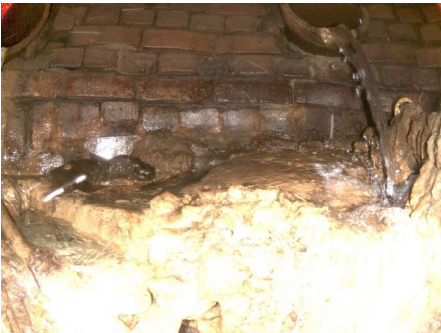
1834b_16edcb0d-7f2c-4b5a-bd27-6b0d1bf9d1bd_e218bb93-14c1-4f86-9c8f-5284944152be_P11.jpg, 00:00:34, 8.00 Obstruction Construction Debris, 30% of cross sectional area from 10 o'clock to 5 o'clock
