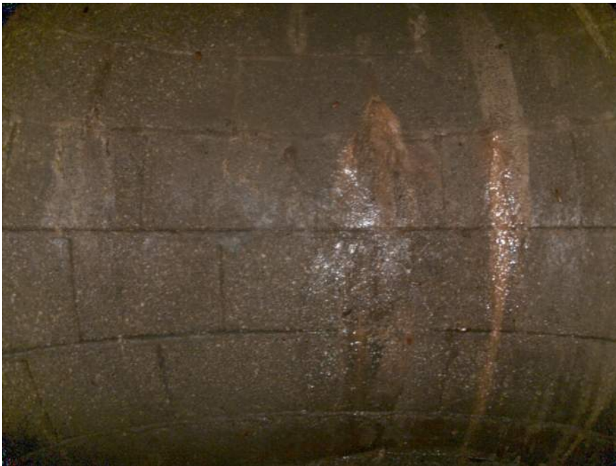
1840b_b7eec4bd-8b4a-4779-9657-5106bc04b13d_f2959d06-e2b7-4c56-8149-9d52cb0888f3_P11.jpg, 00:00:37, 8.74 Infiltration Weeper from 1 o'clock to 4 o'clock, within 8 inch
