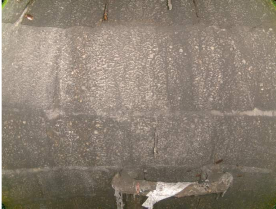
1838_4d464b94-a957-4557-a7ae-8bb14bf4d783_e264c322-c1cf-4ac7-a7cc-1ded439b5dae_P11.jpg, 00:00:15, 2.72 Missing Mortar Large from 12 o'clock to 12 o'clock
