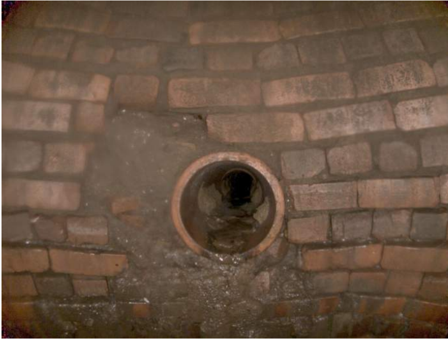
1830_f8e692ed-45a5-4111-be6d-dbb6437dd8b2_de081dc9-a855-40d9-ab49-9ba9a0eef9e8_P11.jpg, 00:00:32, 6.65 Hole Soil Visible from 8 o'clock to 10 o'clock, within 8 inch
