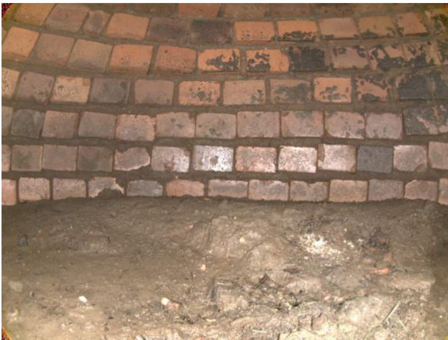
2194_1962243a-d72d-4c62-9e3a-2c87a26c1c57_80c86366-c9e9-43ae-8397-d26630ffeced_P11.jpg, 00:00:20, 3.69 Deposits Settled Gravel, 30% of cross sectional area from 9 o'clock to 2 o'clock, within 8 inch
