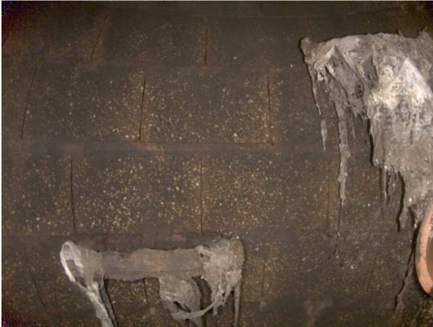
1837c_166883a2-6c9f-44dc-8d3b-993be20f6dc6_9705dbdb-6ee7-4b05-98c9-4de012303572_P11.jpg, 00:00:23, 5.04 Deposits Attached Ragging, 5% of cross sectional area from 7 o'clock to 10 o'clock, within 8 inch
