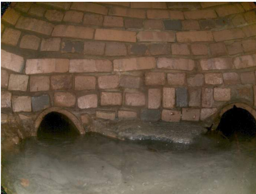
1832_5c717e28-5342-43ea-a091-aed22e190ee5_6c1efc1e-0984-40af-82c8-62d31a60d6ca_P11.jpg, 00:00:00, 7.15 Missing Mortar Large from 12 o'clock to 12 o'clock
