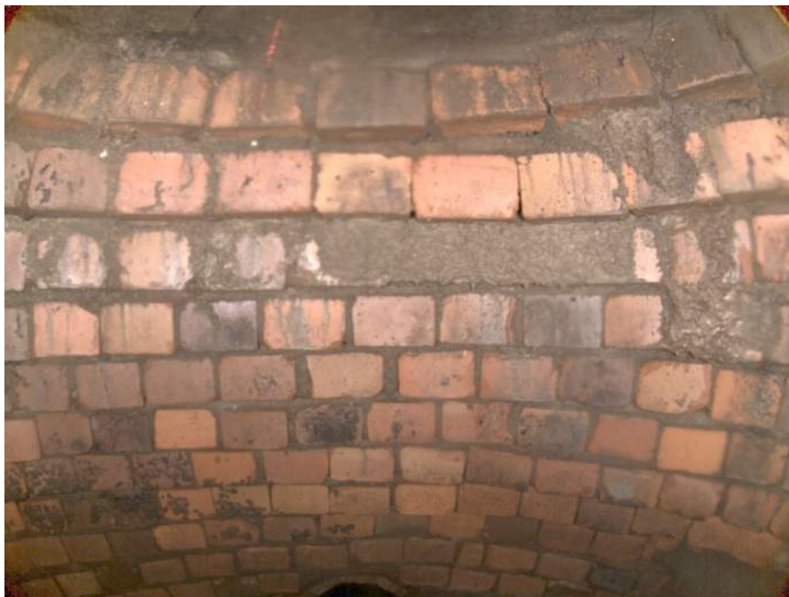
2194_1962243a-d72d-4c62-9e3a-2c87a26c1c57_f68e1b1f-3d93-4c0c-8e24-01f9fd97e403_P11.jpg, 00:00:15, 1.99 Missing Mortar Large from 12 o'clock to 12 o'clock
