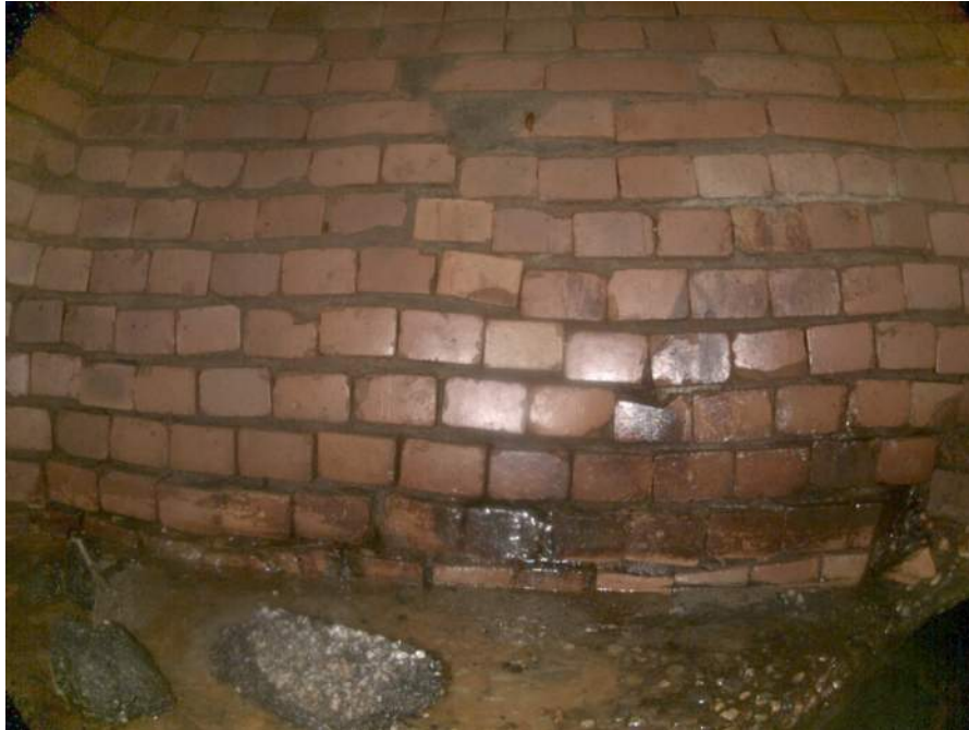
1831_511dce6f-34cf-4134-8589-97e8cd9b2803_68fc3d96-c177-4386-b216-8c69251a096f_P11.jpg, 00:00:30, 6.18 Infiltration Weeper from 1 o'clock to 9 o'clock, within 8 inch
