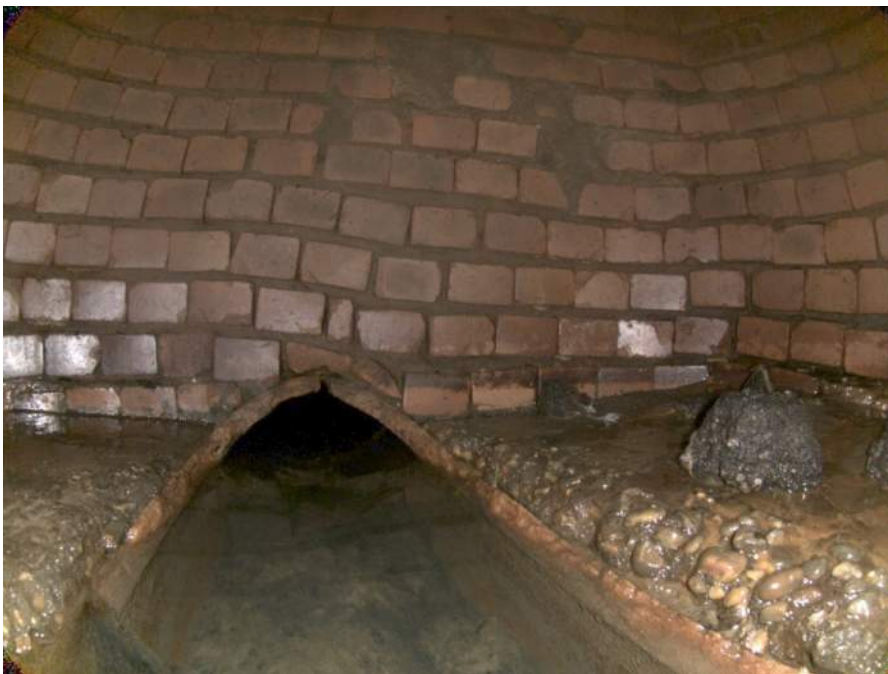
1831_511dce6f-34cf-4134-8589-97e8cd9b2803_26edafcf-9755-414d-ac9d-c19aa6e5a345_PI1.jpg, 00:00:33, 7.29 Surface Damage Aggregate Projecting from 11 o'clock to 2 o'clock, within 8 inch, Start
