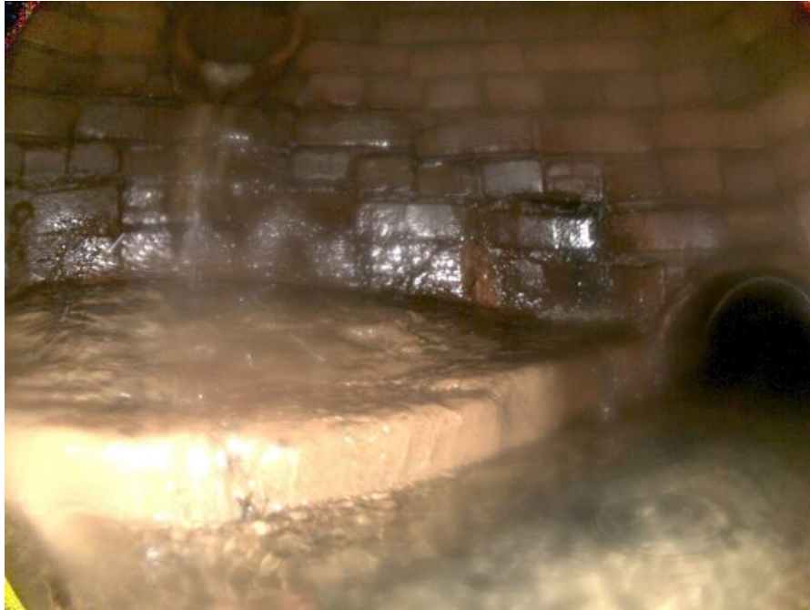
1830_f8e692ed-45a5-4111-be6d-dbb6437dd8b2_0017aeda-f63f-406e-b9a0-11021f9f5edf_PI1.jpg, 00:00:40, 8.26 Missing Mortar Large from 12 o'clock to 2 o'clock
