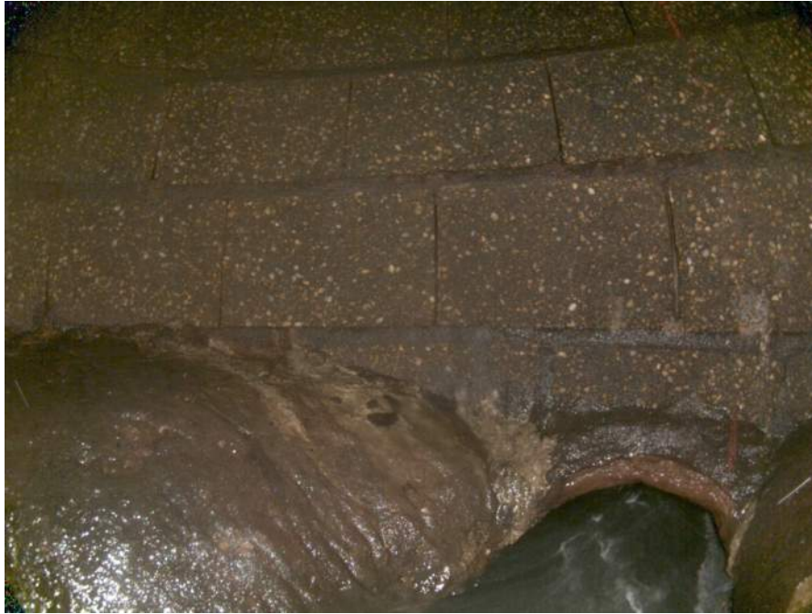
1837c_166883a2-6c9f-44dc-8d3b-993be20f6dc6_eae99878-23a6-4d1a-bde4-6169661a4df4_P11.jpg, 00:00:37, 8.92 Infiltration Weeper from 5 o'clock to 7 o'clock, within 8 inch
