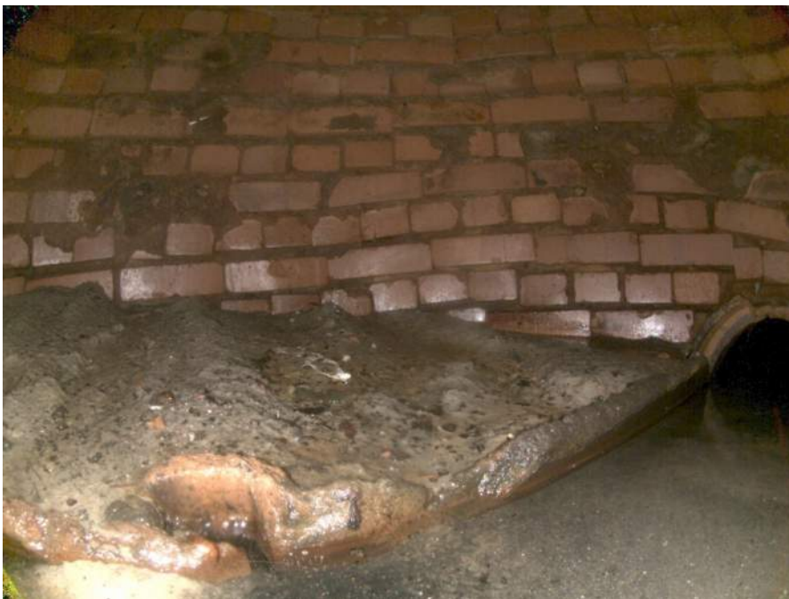
1833a_415896af-f5e7-4861-970c-902a07ead962_67f78bf4-e94b-4f03-8b46-ec002a1f34f9_P11.jpg, 00:00:32, 7.50 Deposits Settled Fine, 45% of cross sectional area from 12 o'clock to 12 o'clock, within 8 inch
