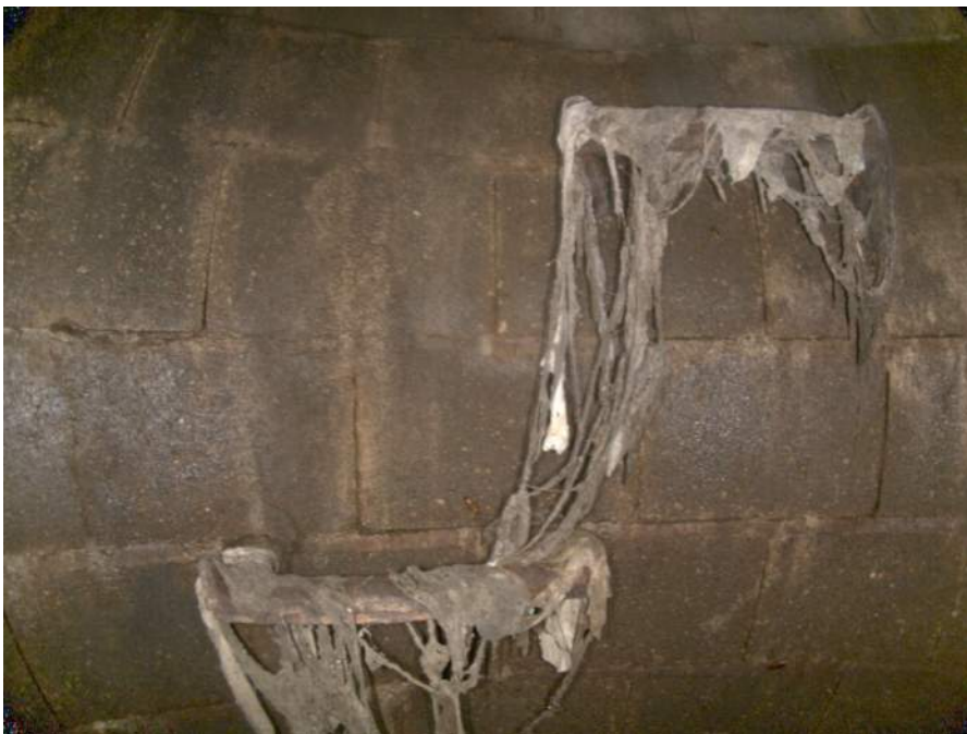
1842_98b1de5e-0e50-41ed-b476-ff581fdb636e_59d47be1-5aec-4a1d-aa9f-42075eb1f695_PI1.jpg, , 5.45 Deposits Attached Ragging, 5% of cross sectional area from 11 o'clock to 2 o'clock, within 8 inch
