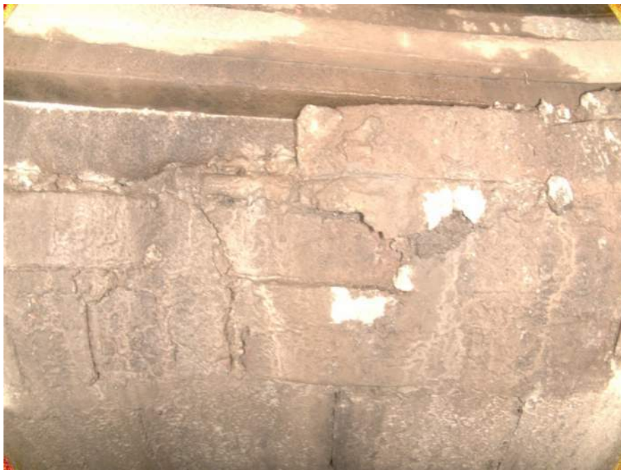
1839_f7a2e778-f07c-460d-8979-384ad1d2d1b3_f10eed2a-ba9a-477d-b689-5f09c7740fe1_PI1.jpg, , 0.99 Missing Mortar Large from 12 o'clock to 12 o'clock
