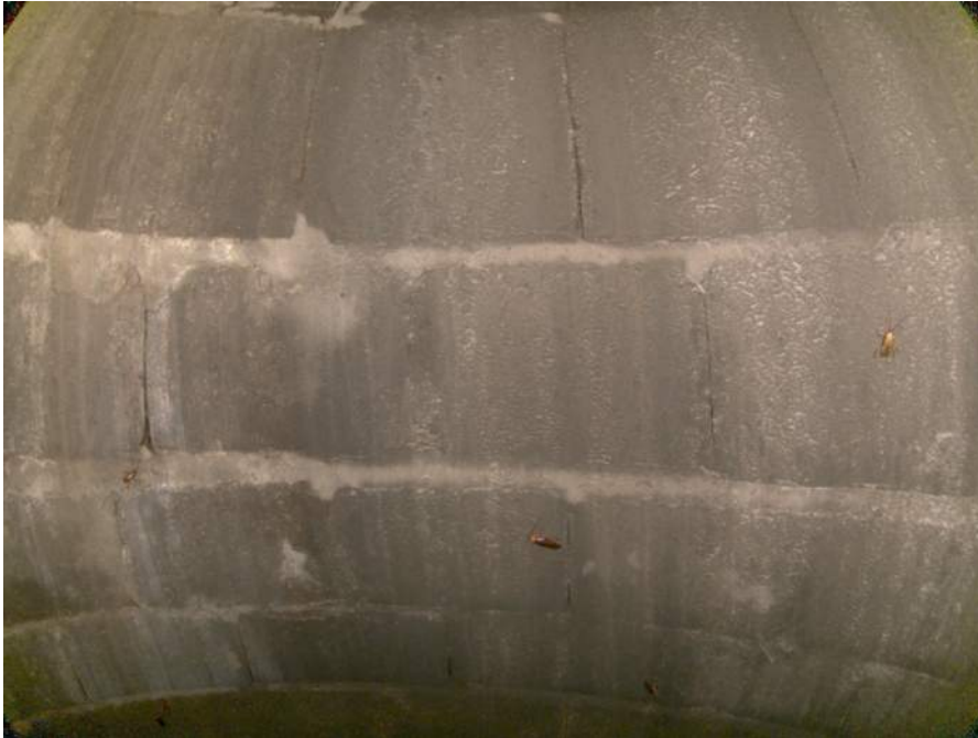
1842_98b1de5e-0e50-41ed-b476-ff581fdb636e_6920a2a8-262a-48f1-bd0b-801a4acf77ef_PI1.jpg, 00:00:18, 2.64 Missing Mortar Large from 12 o'clock to 12 o'clock
