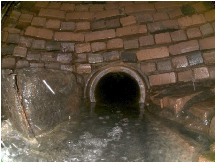
1829b_c3bb5419-4fc2-49bd-9cbb-ae8a522c6251_fafdea7a-ceca-49f8-a0fe-aca9e9443519_P11.jpg, 00:00:43, 10.53 Infiltration Dropper from 12 o'clock to 12 o'clock, within 8 inch
