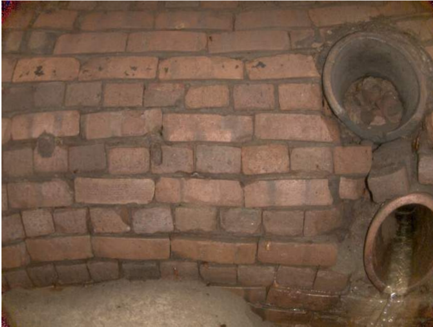
1834b_16edcb0d-7f2c-4b5a-bd27-6b0d1bf9d1bd_28df1de4-7227-40c4-98d3-59bc5e7280d2_P11.jpg, 00:00:27, 6.46 Displaced Brick from 11 o'clock to 1 o'clock
