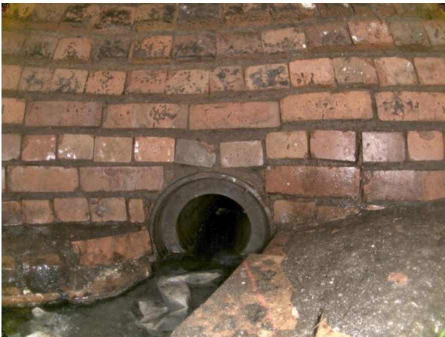
2193c_2b27c63e-1844-43c6-8c49-44849fa40c9a_40c119e6-e6b7-45ce-9ad4-8e93fa226faa_P11.jpg, 00:00:17, 3.25 Missing Mortar Large from 12 o'clock to 12 o'clock
