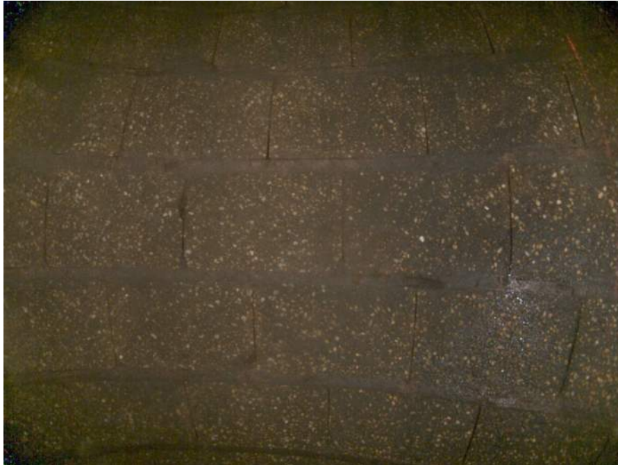
1837c_166883a2-6c9f-44dc-8d3b-993be20f6dc6_17940cd5-8d60-4c09-a955-64962a677a23_P11.jpg, 00:00:27, 5.97 Missing Mortar Large from 12 o'clock to 12 o'clock
