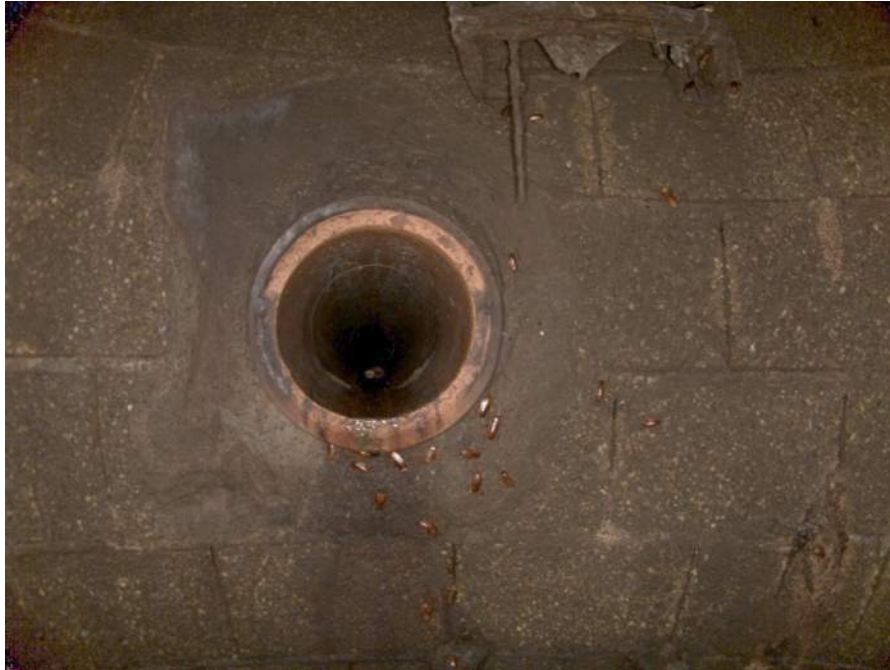
1840b_b7eec4bd-8b4a-4779-9657-5106bc04b13d_35529e95-0a62-48f8-98e8-335a84118c73_P11.jpg, 00:00:31, 7.26 Deposits Attached Ragging, 5% of cross sectional area from 9 o'clock to 12 o'clock, within 8 inch
