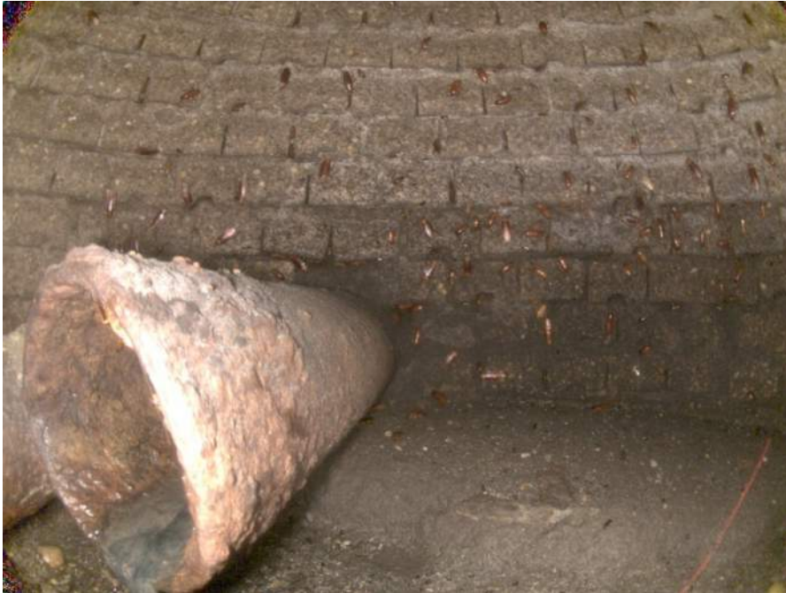
1823d_c2435bdb-6471-4a3b-8f5b-2755123d82bf_4fbed3c0-fe61-4052-b7b0-54b3f722a6e9_P11.jpg, 00:00:14, 3.50 Missing Mortar Large from 12 o'clock to 12 o'clock
