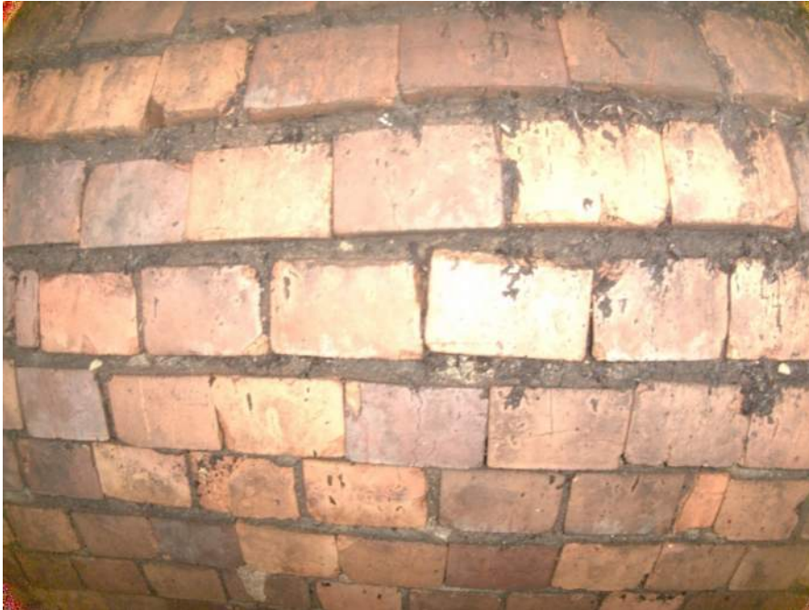
1819_3d72062a-4862-48ce-be8e-7bbe04d95bb2_032d7f95-1b7c-47a9-8899-107e5eae3b48_P11.jpg, 00:00:18, 3.65 Missing Mortar Large from 12 o'clock to 12 o'clock
