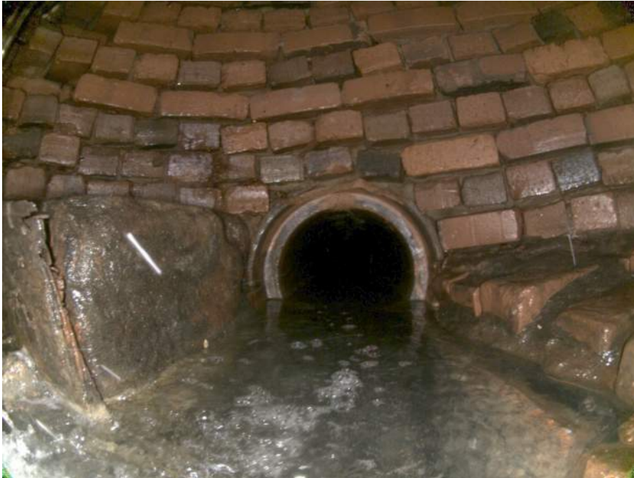
1829b_c3bb5419-4fc2-49bd-9cbb-ae8a522c6251_5dac7274-bd42-468c-9cd3-1184b31077e1_P11.jpg, 00:00:43, 10.48 Missing Mortar Large from 12 o'clock to 12 o'clock
