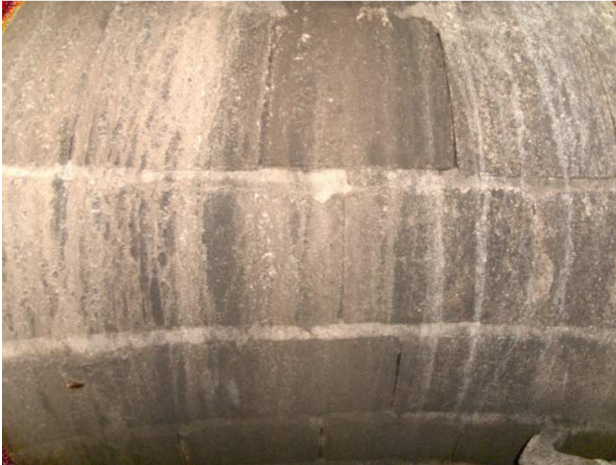
1839_f7a2e778-f07c-460d-8979-384ad1d2d1b3_ee7ac1aa-28e5-461c-bbd2-05e6ce6ef2a0_PI1.jpg, 00:00:15, 2.33 Infiltration Stain from 12 o'clock to 12 o'clock, within 8 inch
