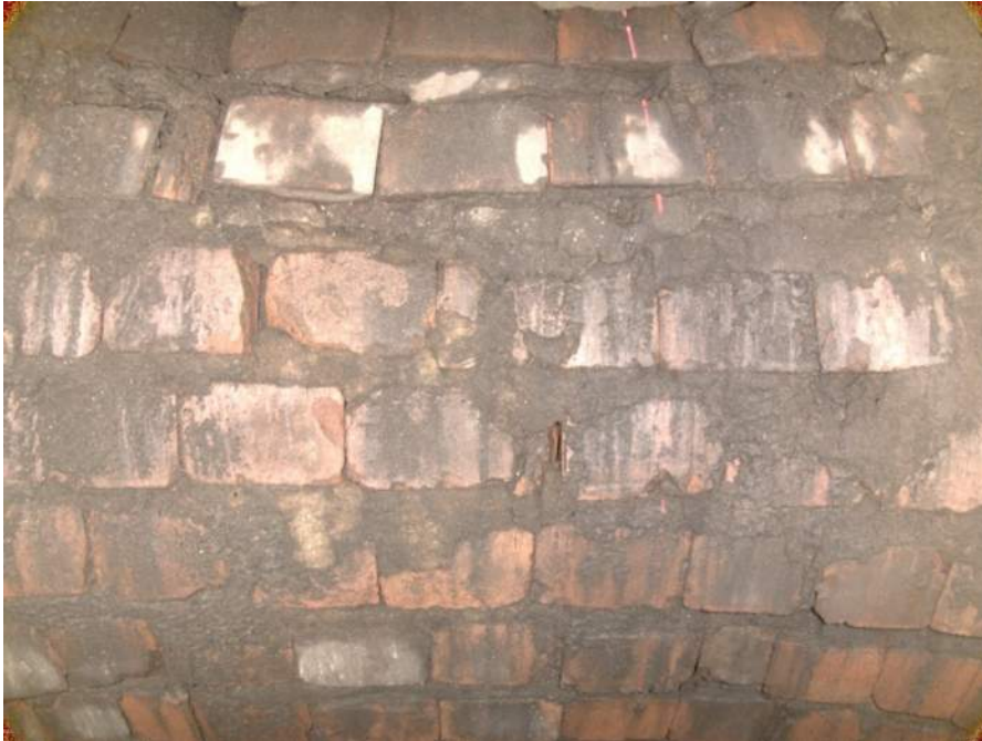
1831_511dce6f-34cf-4134-8589-97e8cd9b2803_08a2a119-0b33-4ac0-aeaf-df97445384cd_PI1.jpg, , 1.49 Missing Mortar Large from 12 o'clock to 12 o'clock
