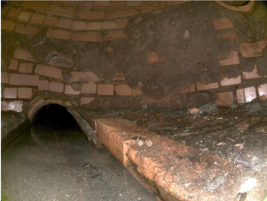
1833a_415896af-f5e7-4861-970c-902a07ead962_38c4850f-5e37-4e65-942c-3ee5629b147e_P11.jpg, 00:00:32, 7.40 Missing Mortar Large from 6 o'clock to 10 o'clock
