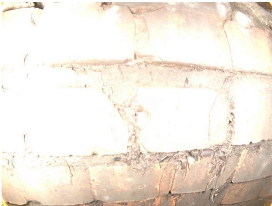
1819_3d72062a-4862-48ce-be8e-7bbe04d95bb2_603a522c-9262-4b30-a481-701e95f23165_P11.jpg, , 1.93 Infiltration Stain from 12 o'clock to 12 o'clock, within 8 inch
