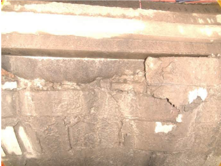
1839_f7a2e778-f07c-460d-8979-384ad1d2d1b3_31e68735-8741-46f8-a0f5-72a580d3aa28_PI1.jpg, 00:00:09, 0.84 Missing Brick from 3 o'clock to 6 o'clock
