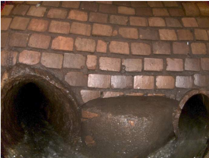
1819_3d72062a-4862-48ce-be8e-7bbe04d95bb2_f70a0414-0ff6-4f34-b025-c17650aa6690_P11.jpg, 00:00:36, 8.64 Missing Mortar Small from 3 o'clock to 9 o'clock
