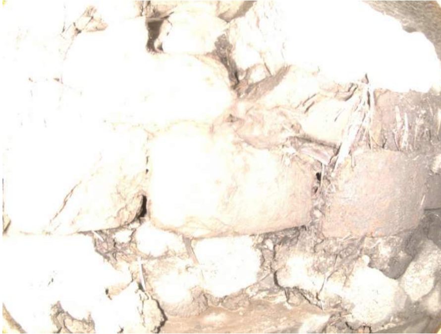
1819_3d72062a-4862-48ce-be8e-7bbe04d95bb2_4dd14b71-64fa-4846-b986-3e011a3effe3_P11.jpg, 00:00:09, 1.12 Missing Mortar Large from 12 o'clock to 12 o'clock
