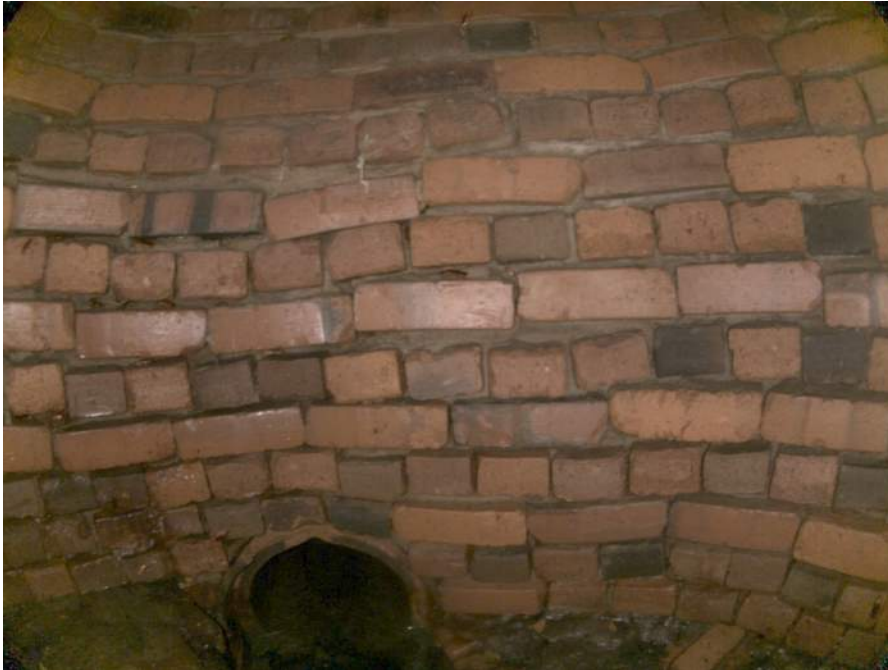
1829b_c3bb5419-4fc2-49bd-9cbb-ae8a522c6251_9e8d4b03-b9ec-4381-9e05-22afe383fce8_P11.jpg, 00:00:37, 8.63 Missing Mortar Large from 12 o'clock to 12 o'clock
