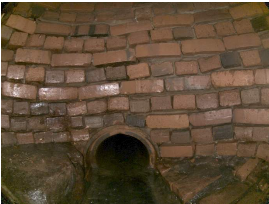
1829b_c3bb5419-4fc2-49bd-9cbb-ae8a522c6251_e8cafd26-0278-49d6-ae87-3f0214f81d3b_P11.jpg, 00:00:40, 9.39 Infiltration Weeper from 12 o'clock to 12 o'clock, within 8 inch
