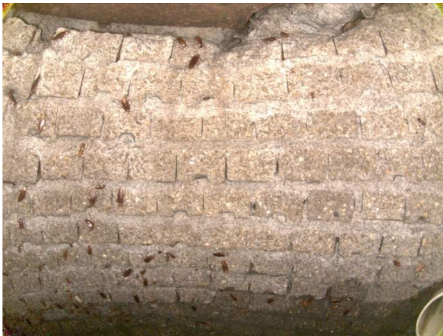
1823d_c2435bdb-6471-4a3b-8f5b-2755123d82bf_3c920d25-da83-4924-ac81-5fffd8014f1a_P11.jpg, 00:00:10, 1.87 Missing Mortar Large from 12 o'clock to 12 o'clock
