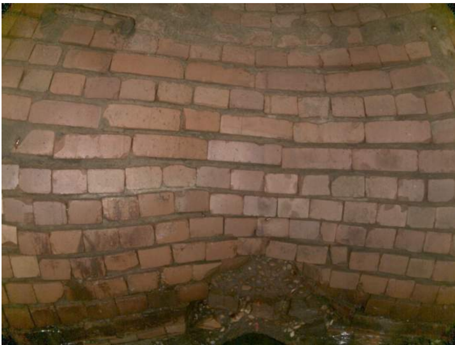
1831_511dce6f-34cf-4134-8589-97e8cd9b2803_367c9464-e72c-4588-83a0-4bdce23a220f_P11.jpg, 00:00:27, 5.49 Missing Mortar Large from 12 o'clock to 12 o'clock
