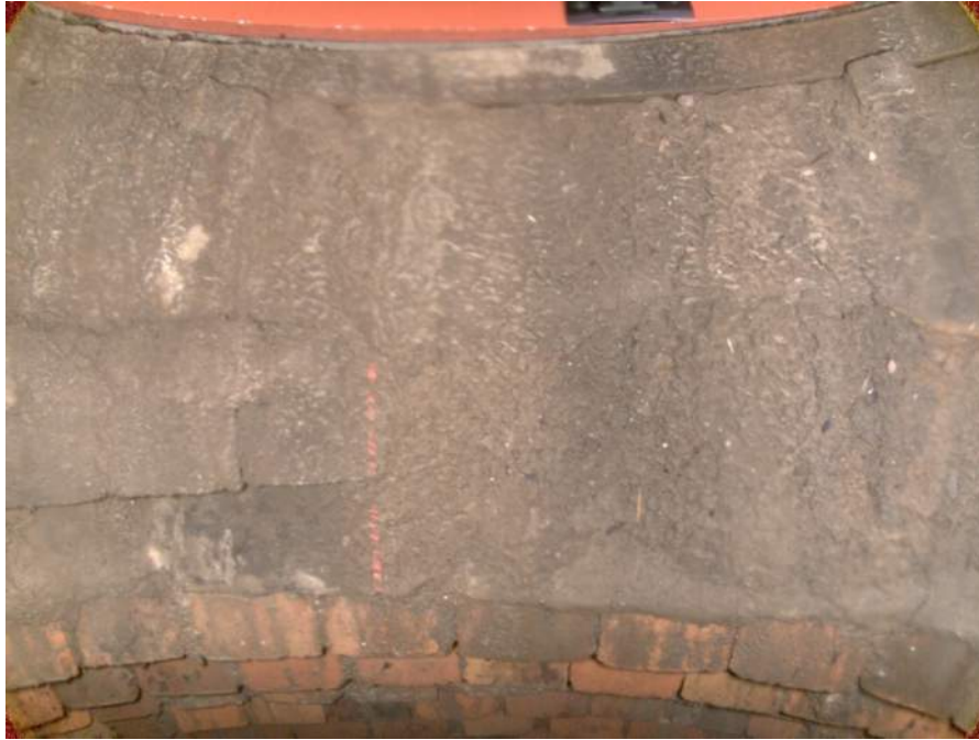
2194_1962243a-d72d-4c62-9e3a-2c87a26c1c57_aeb8bf8d-f294-49aa-a231-debc66a1da36_P11.jpg, , 0.73 Missing Mortar Medium from 12 o'clock to 12 o'clock
