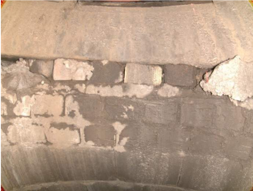
1842_98b1de5e-0e50-41ed-b476-ff581fdb636e_6e4dd29f-ca9b-4492-8423-80415962fdbb_PI1.jpg, 00:00:10, 1.00 Missing Mortar Large from 12 o'clock to 12 o'clock
