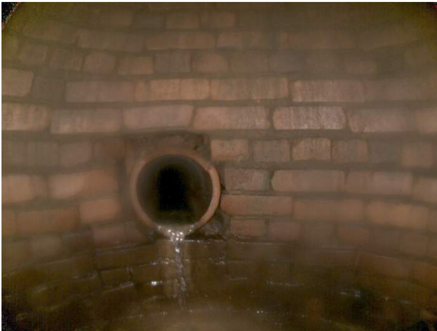
1830_f8e692ed-45a5-4111-be6d-dbb6437dd8b2_0cb77971-2dac-4139-a4e2-6617e6a83616_P11.jpg, 00:00:32, 6.76 Missing Mortar Medium from 2 o'clock to 4 o'clock
