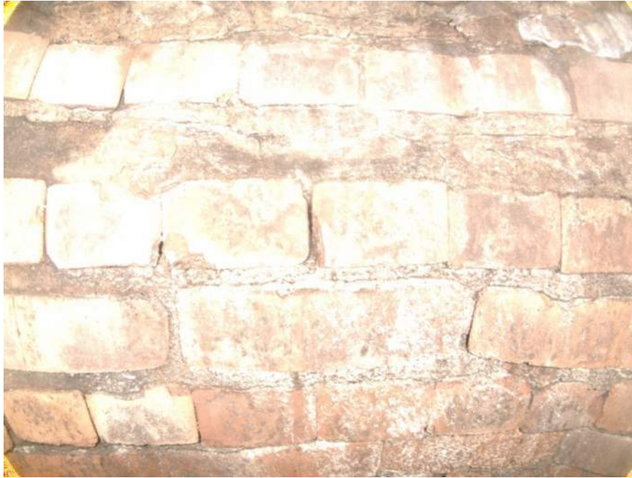
1833a_415896af-f5e7-4861-970c-902a07ead962_e490ae15-1014-4918-bd9c-91c581413cf2_P11.jpg, 1.65 Missing Mortar Large from 4 o'clock to 3 o'clock
