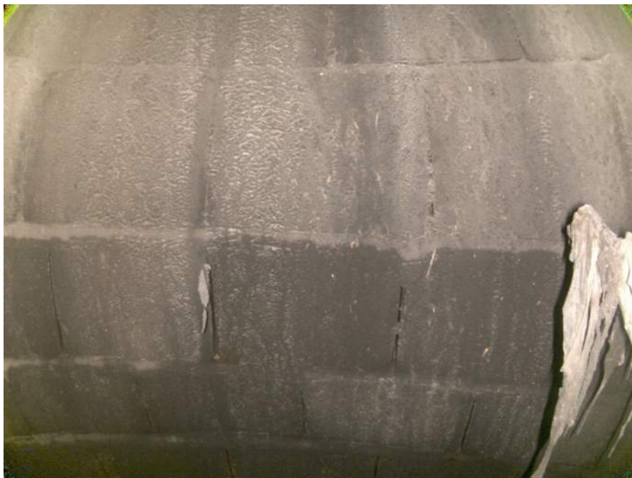
1837c_166883a2-6c9f-44dc-8d3b-993be20f6dc6_1649f046-1a82-498d-82e2-e1f4de576c6f_P11.jpg, 00:00:13, 2.11 Missing Mortar Large from 12 o'clock to 12 o'clock
