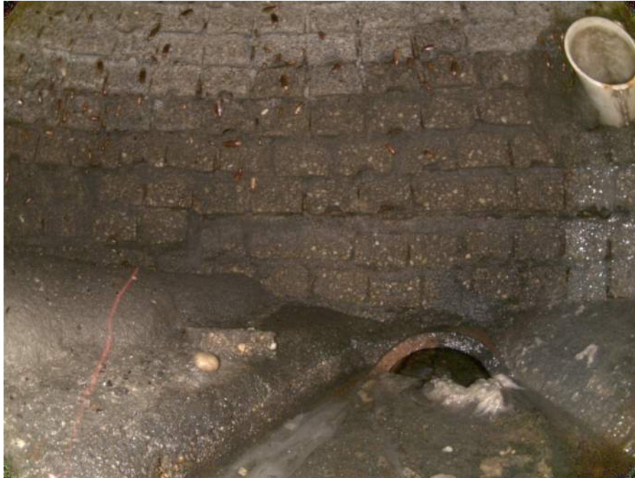
1823d_c2435bdb-6471-4a3b-8f5b-2755123d82bf_b0f872e0-40b7-4b28-929d-b62788bbfa20_P11.jpg, 00:00:15, 4.37 Infiltration Weeper from 6 o'clock to 7 o'clock, within 8 inch
