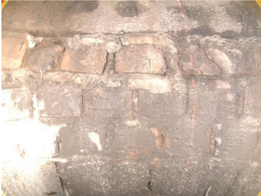
1838_4d464b94-a957-4557-a7ae-8bb14bf4d783_cce063f1-45ad-4048-bcad-c59e8cfe279b_P11.jpg, 00:00:08, 0.96 Missing Mortar Large from 12 o'clock to 12 o'clock
