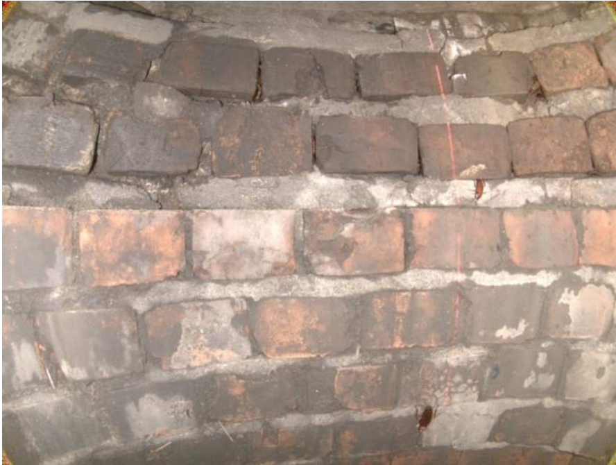
1818_a75925b2-5868-48ca-b1fe-f6e00ecc4562_2fa619db-9017-4731-8de7-af26d82f40cc_P11.jpg, 1.76 Missing Mortar Large from 12 o'clock to 12 o'clock
