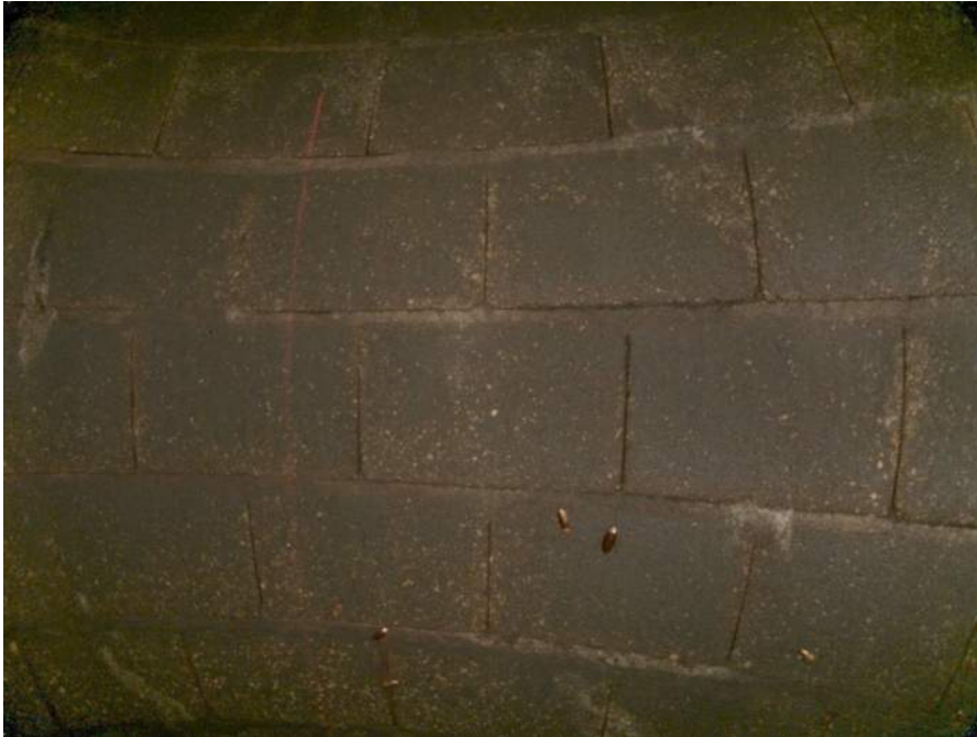
1842_98b1de5e-0e50-41ed-b476-ff581fdb636e_ec832979-62f8-4c91-8da5-8ac031d99ae4_PI1.jpg, 00:00:32, 6.40 Surface Damage Aggregate Visible from 12 o'clock to 12 o'clock, within 8 inch
