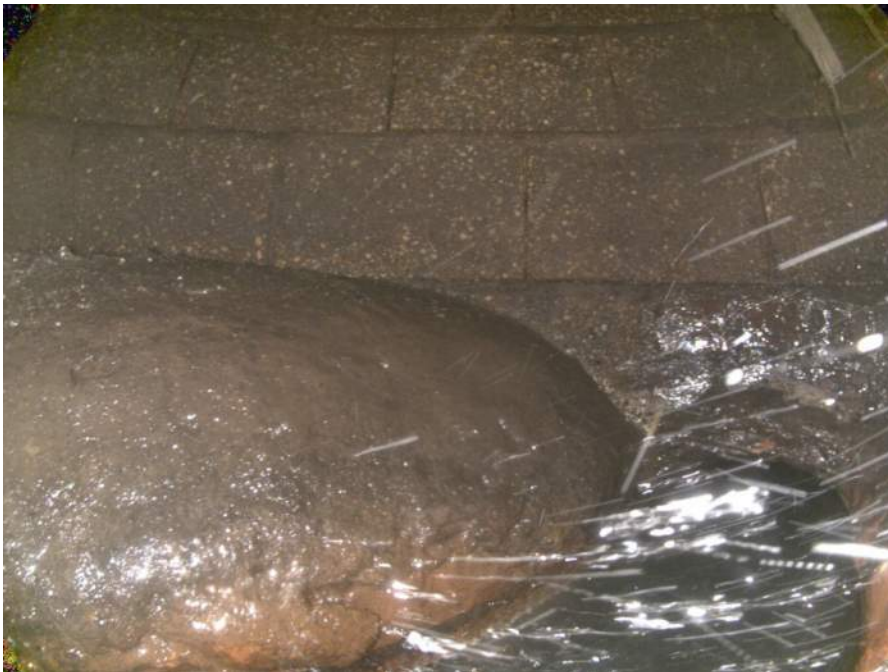
1838_4d464b94-a957-4557-a7ae-8bb14bf4d783_bcf02ece-7deb-4f88-be2a-457d033fda34_PI1.jpg, 00:00:38, 8.39 Infiltration Weeper from 5 o'clock to 7 o'clock, within 8 inch
