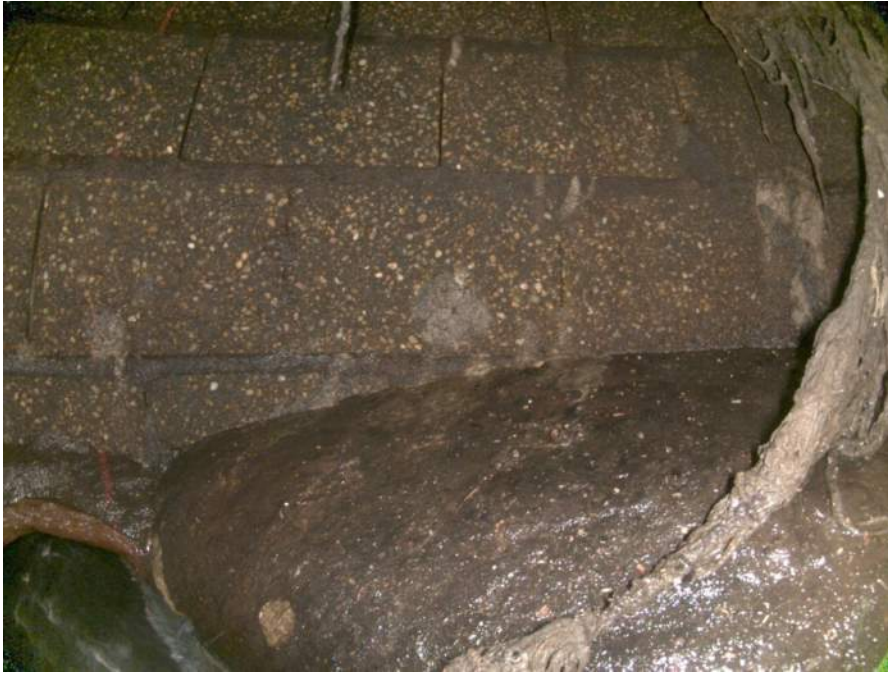
1837c_166883a2-6c9f-44dc-8d3b-993be20f6dc6_fe294033-28b6-44f4-8a38-8d327567a80b_P11.jpg, 00:00:37, 8.60 Infiltration Weeper from 7 o'clock to 10 o'clock, within 8 inch
