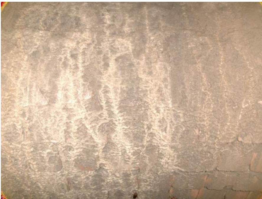
1831_511dce6f-34cf-4134-8589-97e8cd9b2803_88dfd25-526c-4368-a44f-9a542564fddd_PI1.jpg, 00:00:12, 1.54 Infiltration Stain from 7 o'clock to 2 o'clock, within 8 inch
