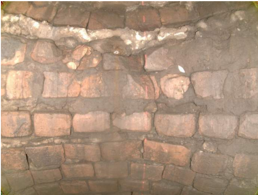
1829b_c3bb5419-4fc2-49bd-9cbb-ae8a522c6251_e2247d21-da48-437d-b0c9-70c0777bef81_P11.jpg, 00:00:10, 1.51 Missing Mortar Large from 12 o'clock to 12 o'clock
