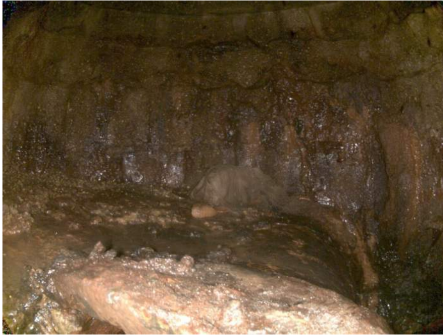
1835c_f2d6f72e-14ab-43ef-906b-8e360bc88926_591172c5-468d-4e0c-a783-9c27bbd0c414_P11.jpg, 00:00:31, 7.01 Deposits Attached Ragging, 5% of cross sectional area from 2 o'clock to 6 o'clock, within 8 inch
