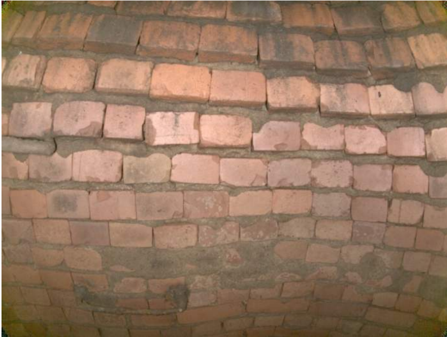
1831_511dce6f-34cf-4134-8589-97e8cd9b2803_25daea92-acd2-4201-a301-2eaaa0f1d117_P11.jpg, 00:00:18, 3.24 Missing Mortar Large from 12 o'clock to 12 o'clock
