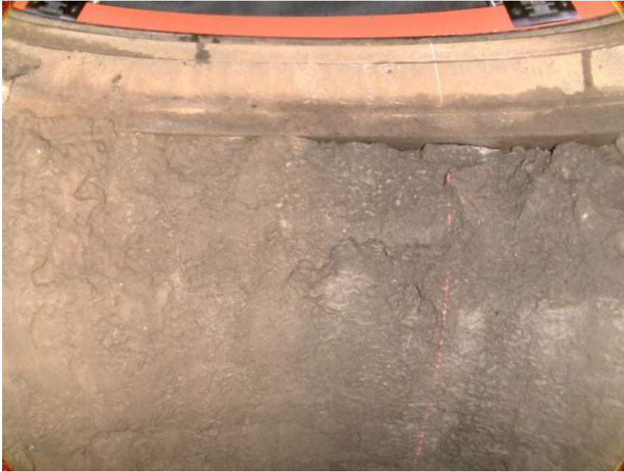
1830_f8e692ed-45a5-4111-be6d-dbb6437dd8b2_978e29b1-d29c-43a2-9208-b804c66c84c3_P11.jpg, 00:00:07, 0.67 Missing Mortar Medium from 12 o'clock to 12 o'clock
