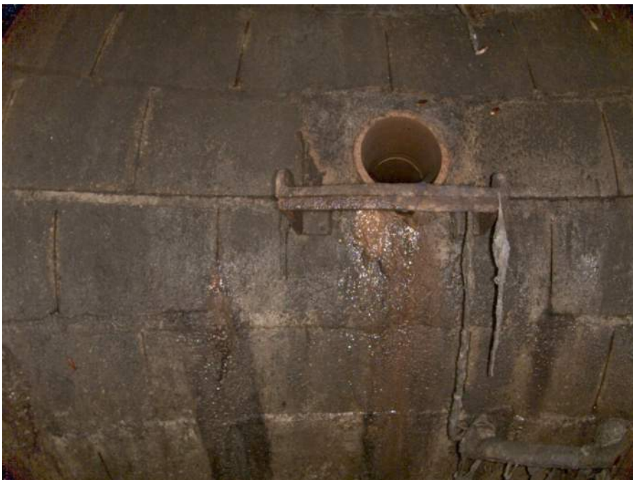
1839_f7a2e778-f07c-460d-8979-384ad1d2d1b3_02e3030d-803b-4789-b031-fbff11776bf2_P11.jpg, 00:00:26, 5.08 Infiltration Weeper Connection from 9 o'clock to 11 o'clock, within 8 inch
