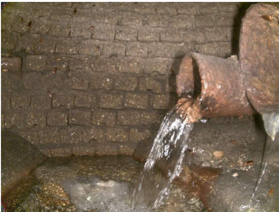
1823d_c2435bdb-6471-4a3b-8f5b-2755123d82bf_13f7f9e5-b29d-4219-b01c-6b84ab9916f3_P11.jpg, 00:00:15, 4.04 Infiltration Weeper from 11 o'clock to 1 o'clock, within 8 inch
