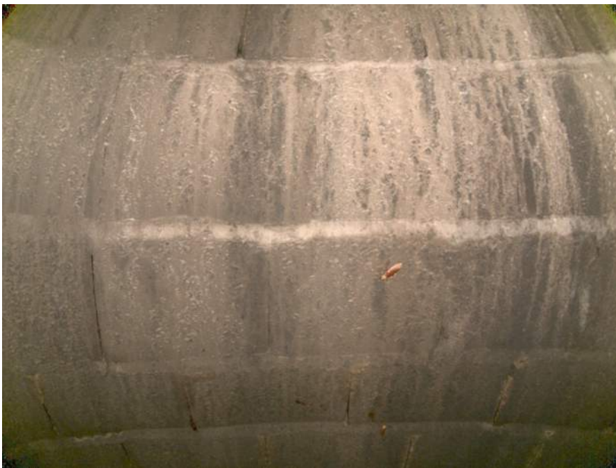
1839_f7a2e778-f07c-460d-8979-384ad1d2d1b3_2ceee7b3-5cb1-48fb-b1bd-03d0ef3fc47e_PI1.jpg, 00:00:17, 2.77 Missing Mortar Large from 12 o'clock to 12 o'clock
