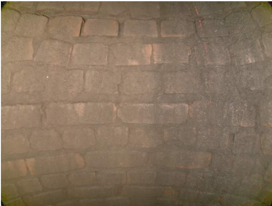
1830_f8e692ed-45a5-4111-be6d-dbb6437dd8b2_f26ac0c9-3f10-4b31-9cd6-9eb7d445b966_P11.jpg, 00:00:17, 3.09 Infiltration Stain from 4 o'clock to 9 o'clock, within 8 inch
