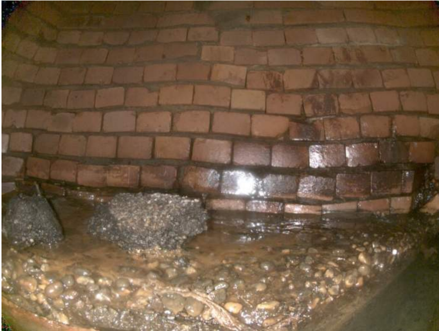
1831_511dce6f-34cf-4134-8589-97e8cd9b2803_f6d5ccc0-e1d8-4e3e-8fe5-b6471e9965fe_PI1.jpg, 00:00:33, 7.05 Obstruction Construction Debris, 5% of cross sectional area from 1 o'clock to 4 o'clock
