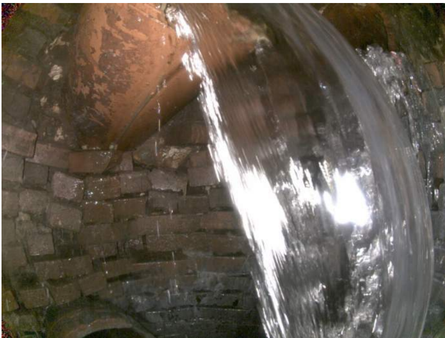
1828b_5154b3dc-7153-4625-bad4-be8d5b792f69_a9eef5b8-2357-475d-a879-3b8cd9676573_P11.jpg, 00:00:39, 8.18 Displaced Brick from 8 o'clock to 11 o'clock
