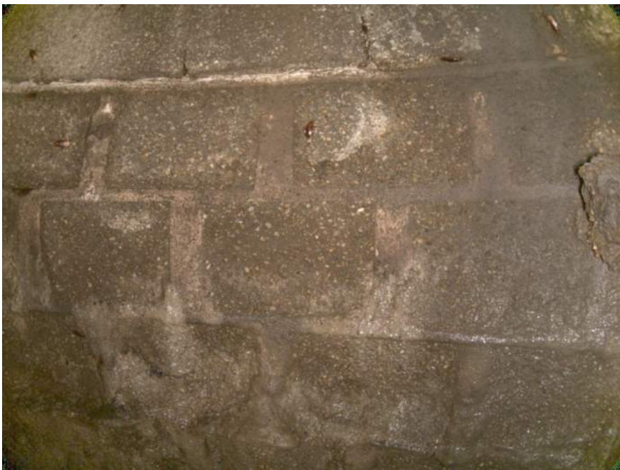
1835c_f2d6f72e-14ab-43ef-906b-8e360bc88926_e8a7c4a0-bf72-4c2e-9871-44d321ec9f86_PI1.jpg, 00:00:21, 4.27 Surface Damage Aggregate Visible from 12 o'clock to 12 o'clock, within 8 inch
