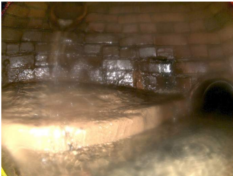
1830_f8e692ed-45a5-4111-be6d-dbb6437dd8b2_3adc60c1-ed59-466f-9d64-e0d2b984441e_PI1.jpg, 00:00:40, 8.48 Obstruction Construction Debris, 35% of cross sectional area from 1 o'clock to 10 o'clock
