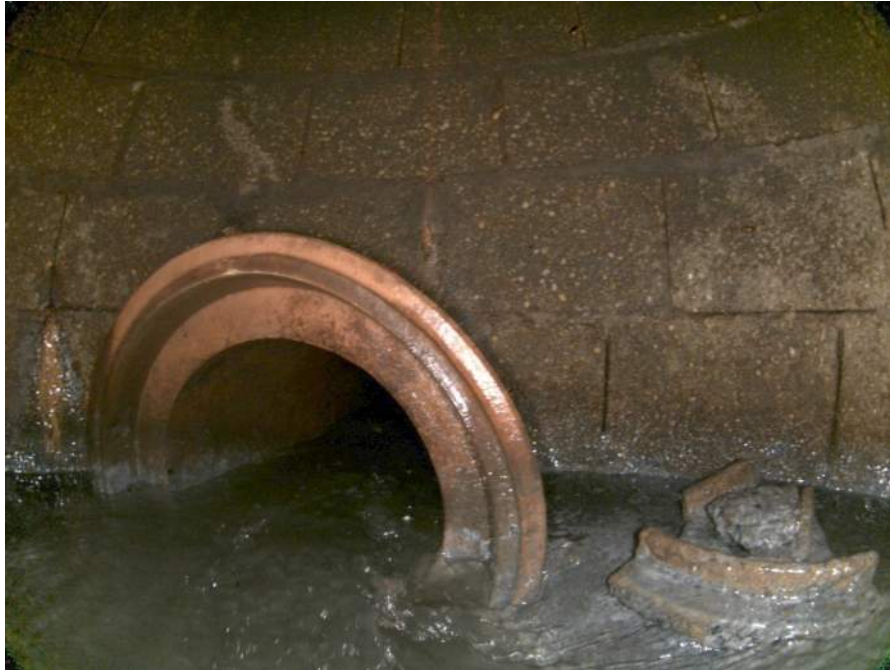
1842_98b1de5e-0e50-41ed-b476-ff581fdb636e_da26af56-9524-4d1f-8dc6-a1a065c0e713_P11.jpg, 00:00:43, 9.47 Obstruction Construction Debris, 5% of cross sectional area from 7 o'clock to 9 o'clock
