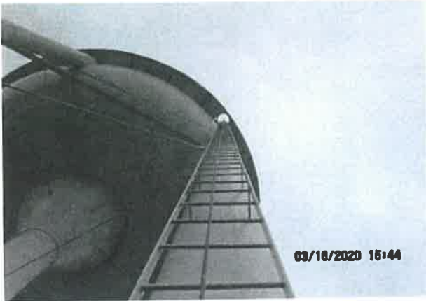
Safety climb cable
