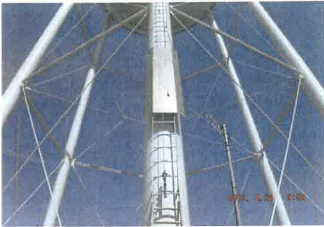
Ladder equipped with safety climb
