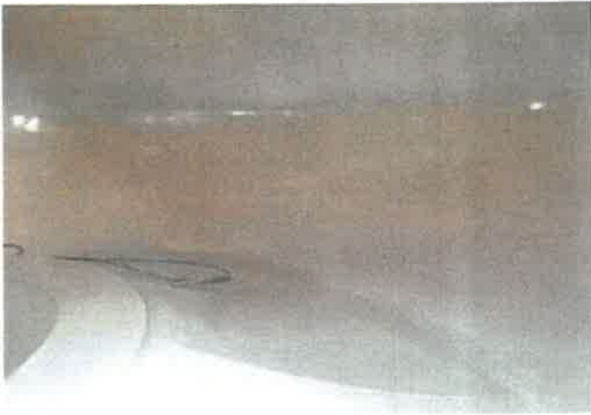
Interior After Washout
