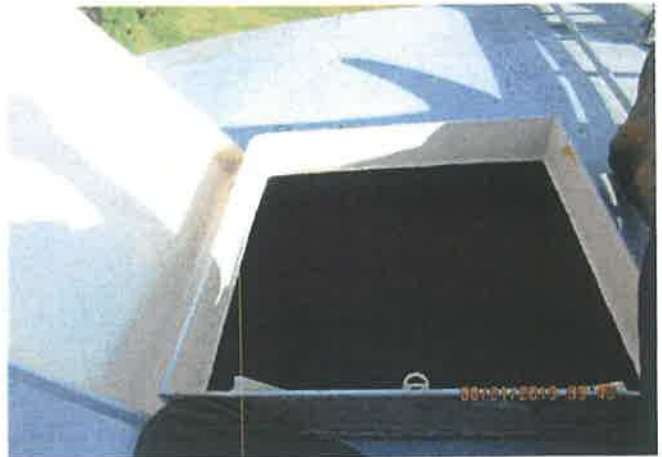
Wet Interior Roof Access Hatch Open
