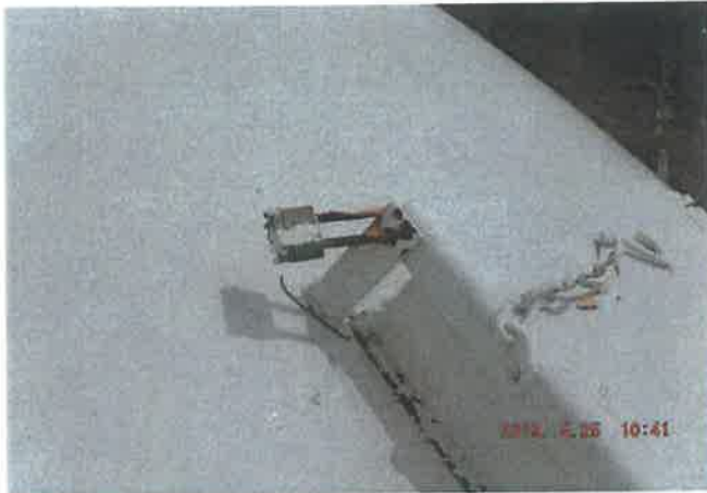
Roof access hatch locked
