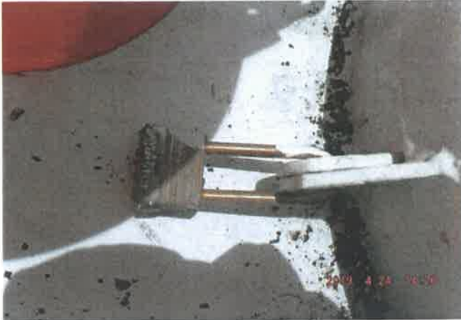
Roof access hatch locked
