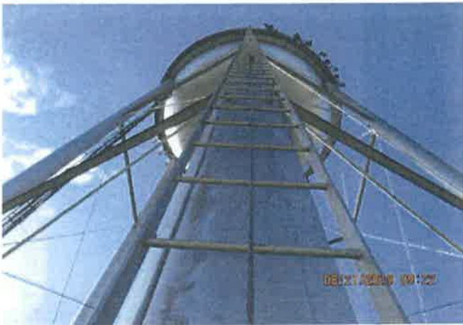
Cable Safety Climb On Access Ladder
