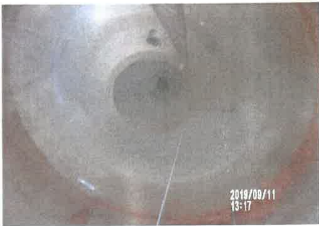
Interior After Washout
