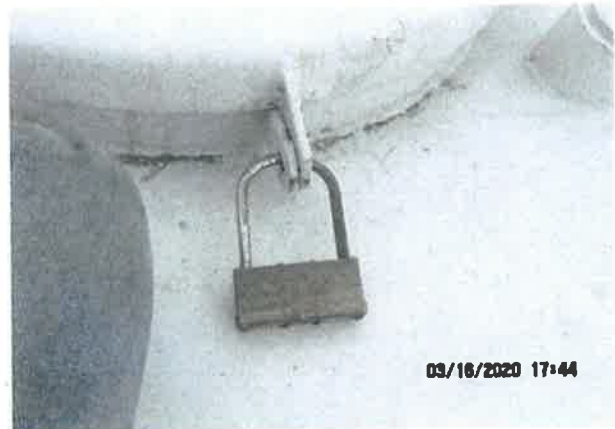
Roof access hatch locked
