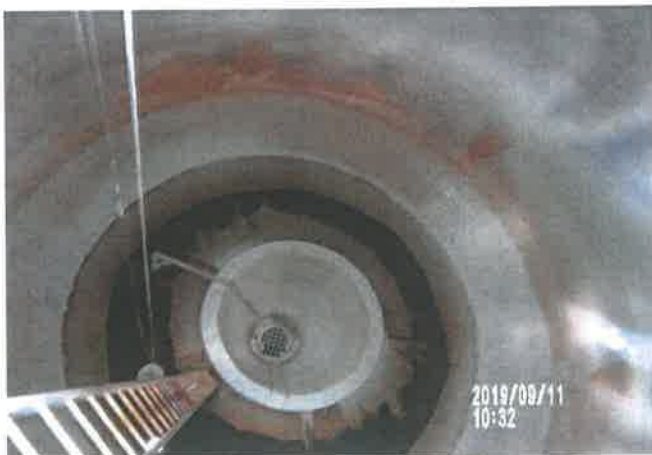
Interior Access Ladder with Minor Deficiencies
