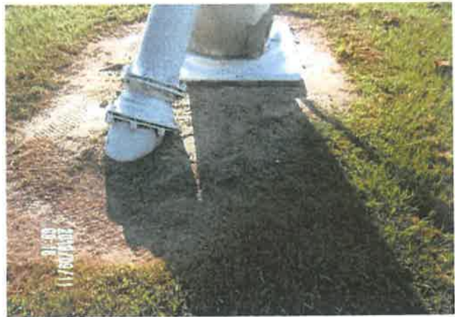
Overflow Pipe Termination
