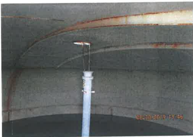
Interior Roof with Deficiencies
