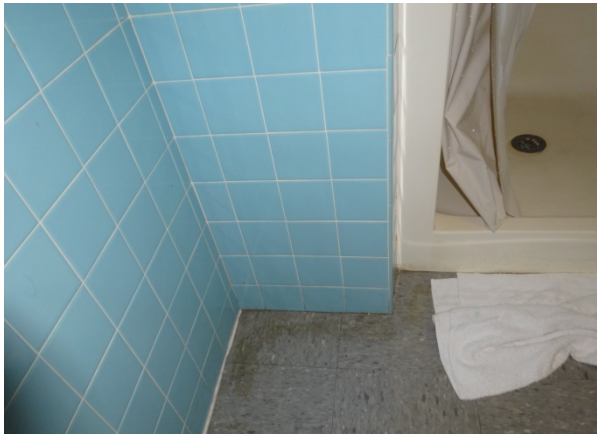
Photo 21 Bathroom – moisture damage to floor tile
