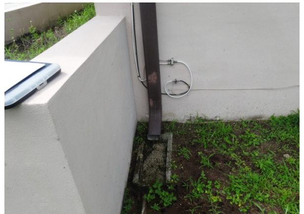
Photo 6 Downspout with minor washout and not effectively diverting water away
