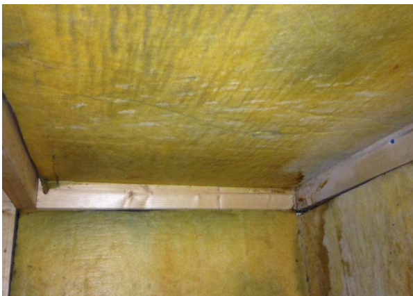
Photo 35 Stains on Fiberglass insulation of AHU
