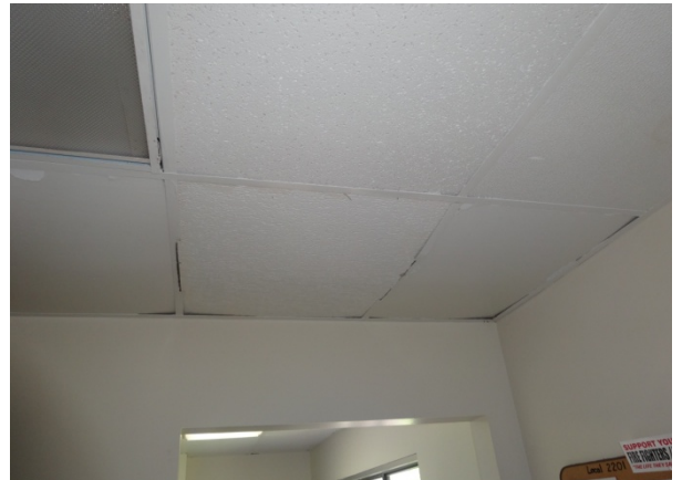
Photo 16 In front of entry to kitchen – example of painted ceiling tiles previously stained
