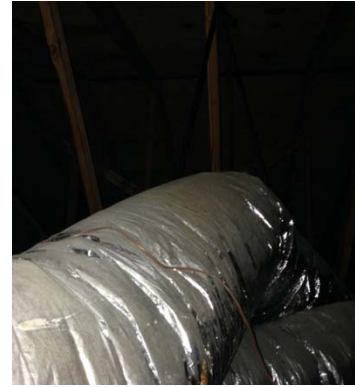
Photo 38 Dust on flexible fiberglass ducts above ceiling tiles
