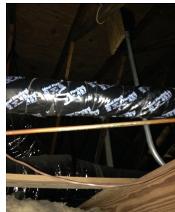
Photo 36 Wet insulation on condensate line, above ceiling tiles in Ready room
