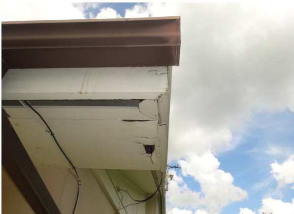
Photo 5 Deteriorated fascia and soffit
