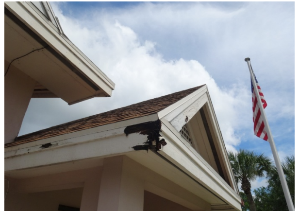
Photo 4 Deteriorated fascia above entry door
