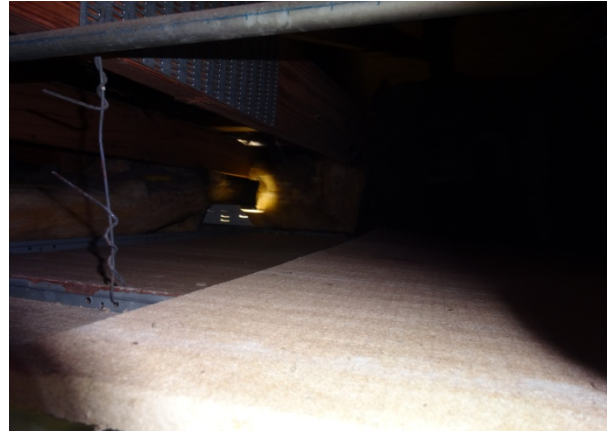
Photo 26 Above ready room – insulation moved out of place
