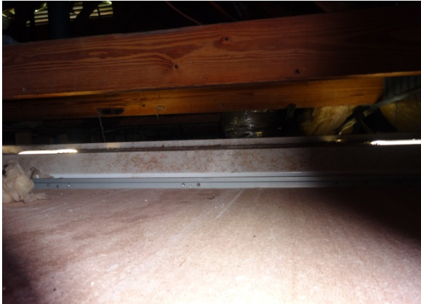
Photo 25 Above ready room – rust on light fixture
