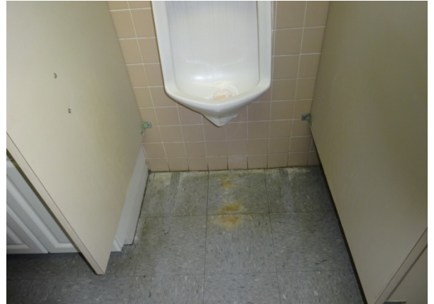
Photo 14 Moisture damage at vinyl floor tiles
