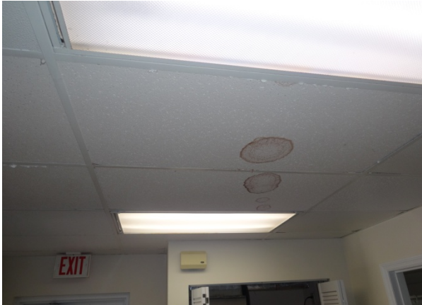
Photo 13 Stained ceiling tile in front of A/C closet – moisture dripping from coolant line in attic
