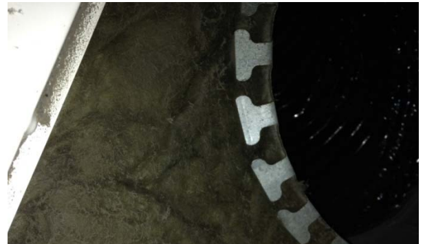
Photo 40 Dust at A/C return in Bunk area
