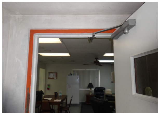
Photo 12 Door from apparatus bay into office area – no weather-stripping
