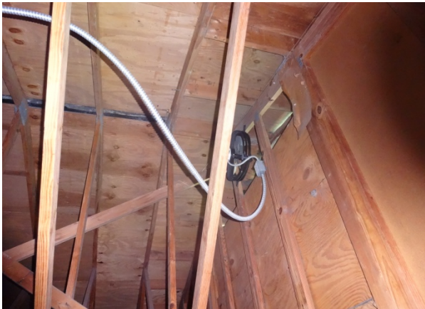
Photo 27 Attic exhaust fan – appears to be non-operational
