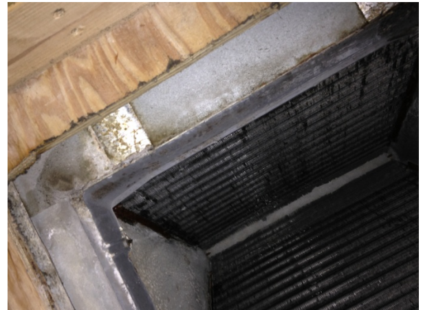
Photo 34 S.V.M at coils of AHU in Ready room
