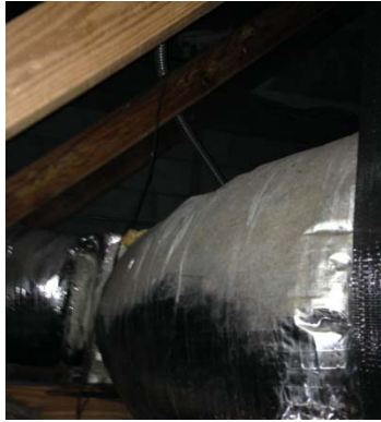
Photo 37 Dust on flexible fiberglass ducts above ceiling tiles
