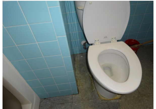
Photo 22 Bathroom – moisture damage to floor tile
