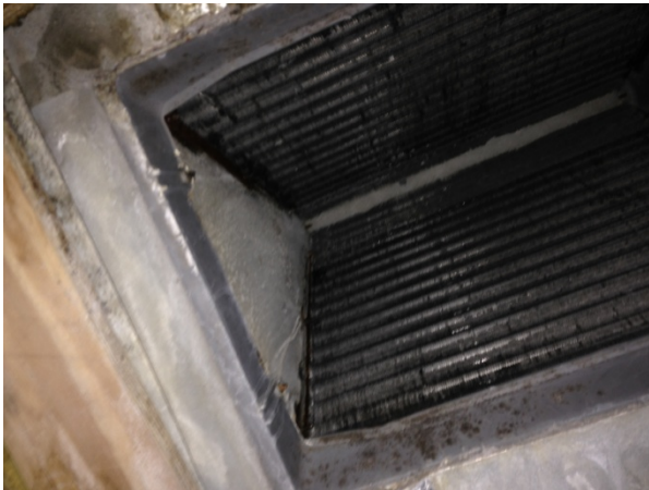
Photo 33 SVM at coils of AHU in Ready room
