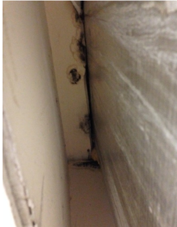
Photo 31 Suspect Visible Mold (SVM) on ceiling of A/C closet
