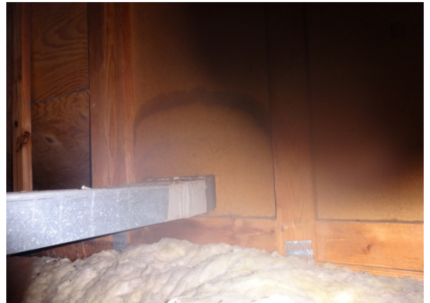
Photo 28 Moisture stain on exterior wall sheathing in attic at vent
