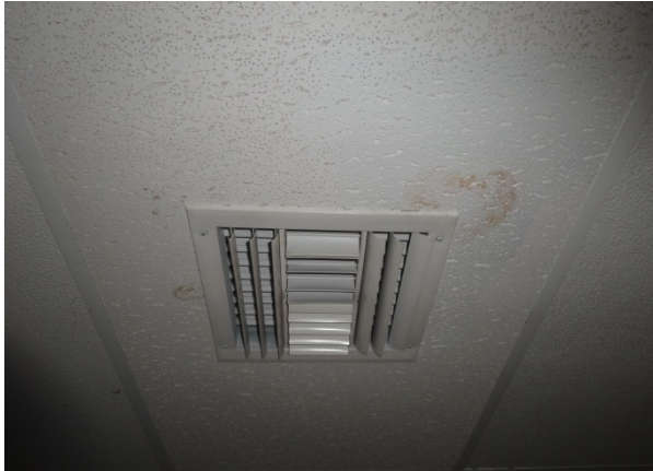
Photo 19 Stained ceiling tile and SVM on diffuser in ready room
