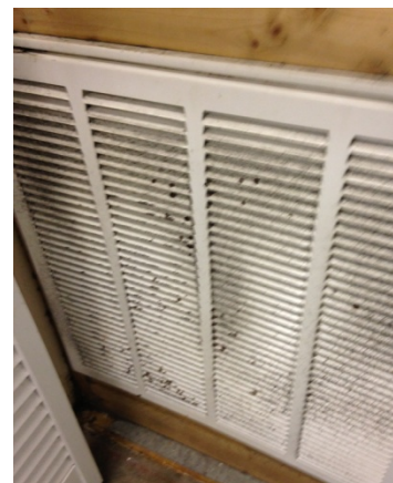
Photo 30 Vent of A/C in Ready room
