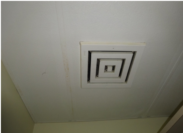
Photo 15 Vent fan in men's bathroom, exhausts into attic – SVM, rust on ceiling grid
