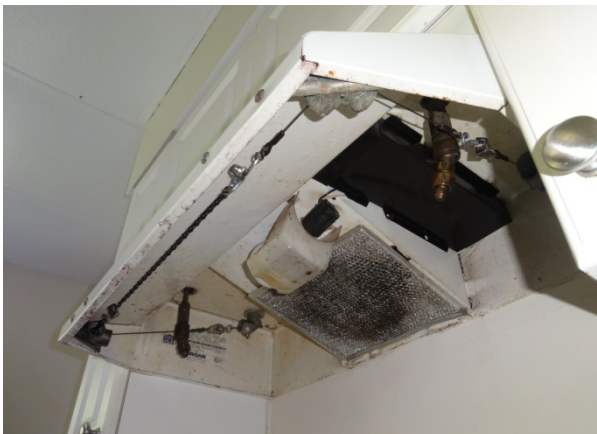
Photo 17 Underside of stove vent hood – needs cleaning and SVM
