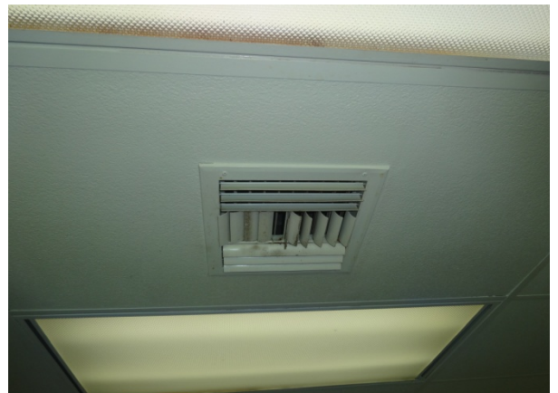
Photo 18 Diffuser in kitchen - SVM
