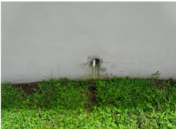
Photo 9 Condensate drain from icemaker – no p-trap and moisture is not directed away from building
