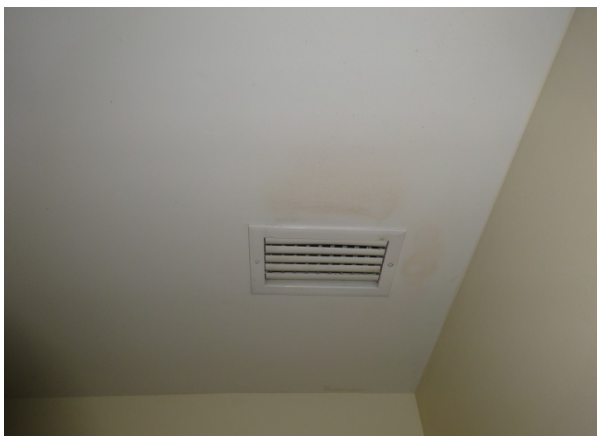
Photo 23 Bathroom, stains on ceiling (SVM) and diffuser has been painted
