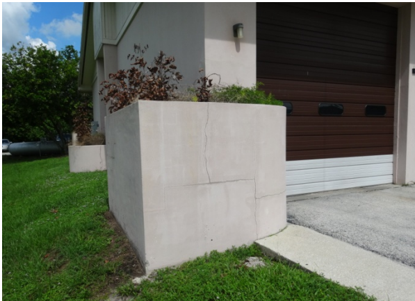
Photo 3 Typical cracks in planter walls
