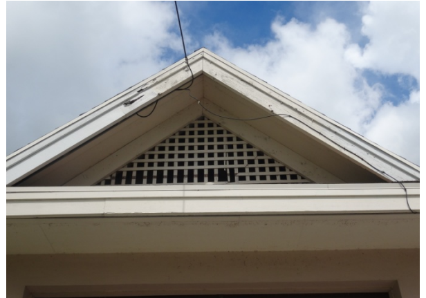
Photo 2 Damaged lattice above entry door
