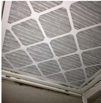
Photo 39 Visible signs of SVM on A/C return in Bunk area
