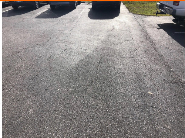
Image 2 – Low to Medium Sev. Block Cracking
