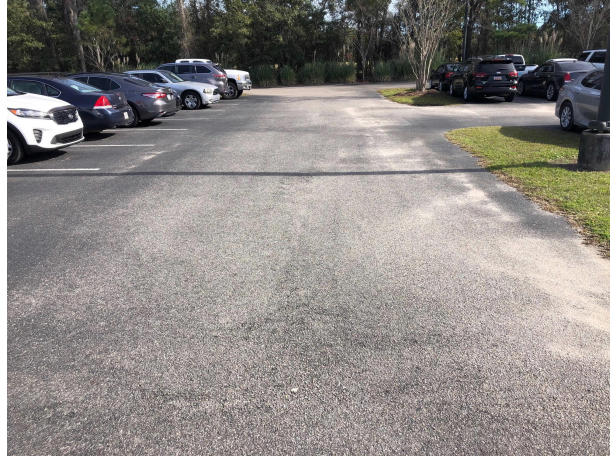
Image 4 - Fair Pavement Conditions
