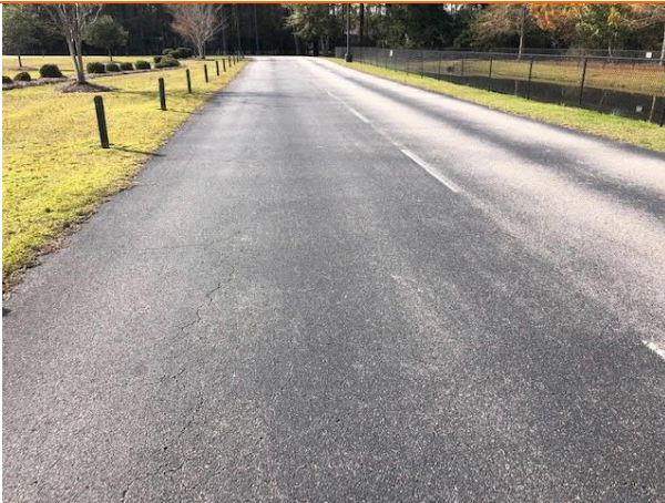
Image 1 - Low Sev. Block Cracking
