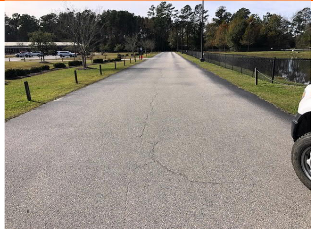
Image 10 - Low Sev. Longitudinal Cracking
