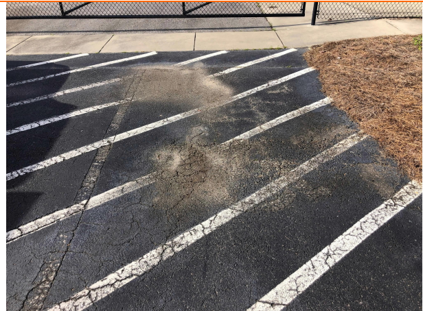
Image 8 - Med. Sev. Alligator Cracking
