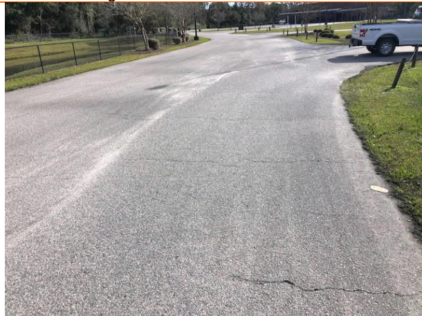
Image 6 - Low Sev. Edge Cracking
