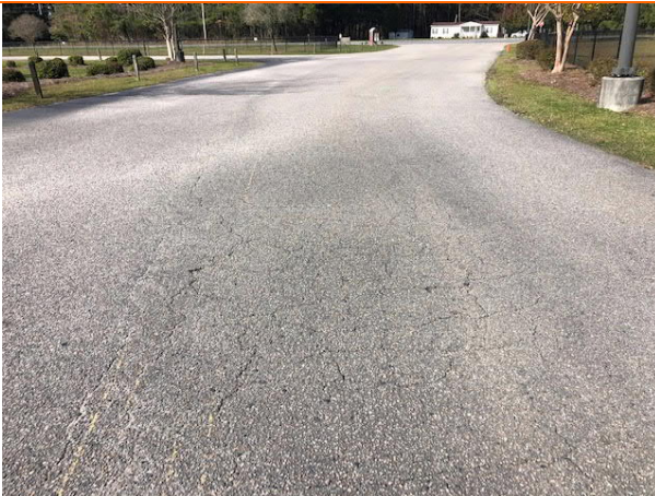
Image 7 - Low Sev. Alligator Cracking
