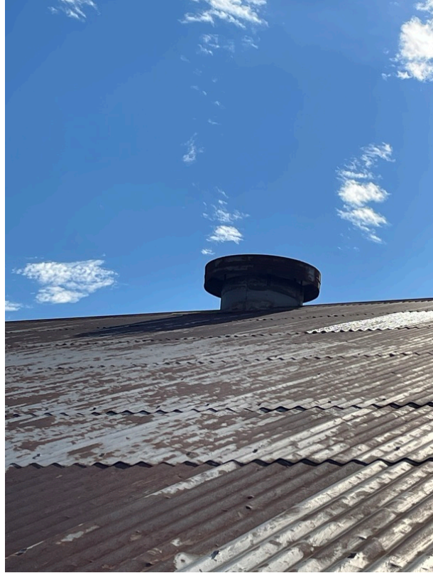
View of the assumed asbestos-containing Roof Penetration Materials (HA 4-4)
