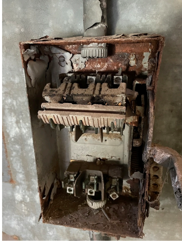
View of the assumed asbestos-containing Cementitious Electrical Breaker Bars (HA 2-4)
