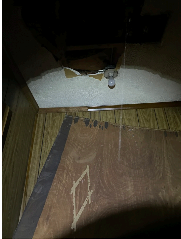
View of the asbestos-containing White Ceiling Texture over Wallboard (HA 3-3)
