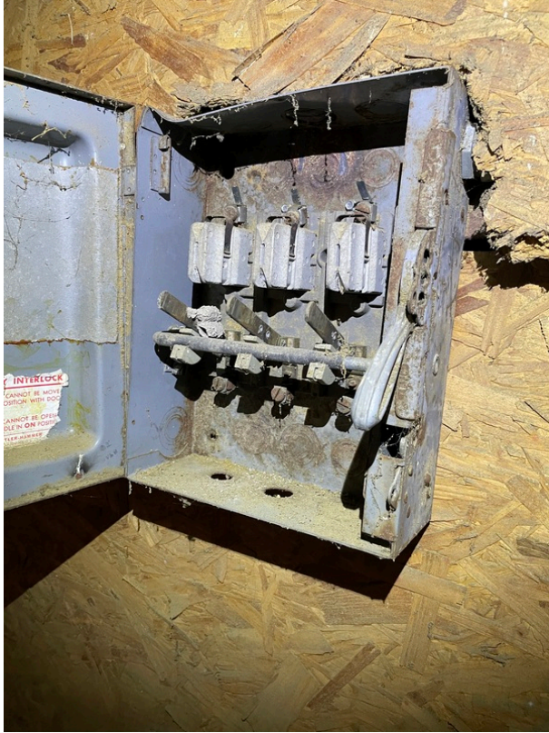
View of the assumed asbestos-containing Cementitious Electrical Breaker Bars (HA 4-3)
