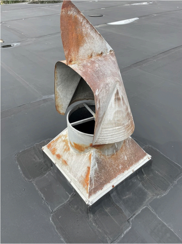
General view of the asbestos-containing Silver Penetration Paint on a roof penetration (HA 3-10)
