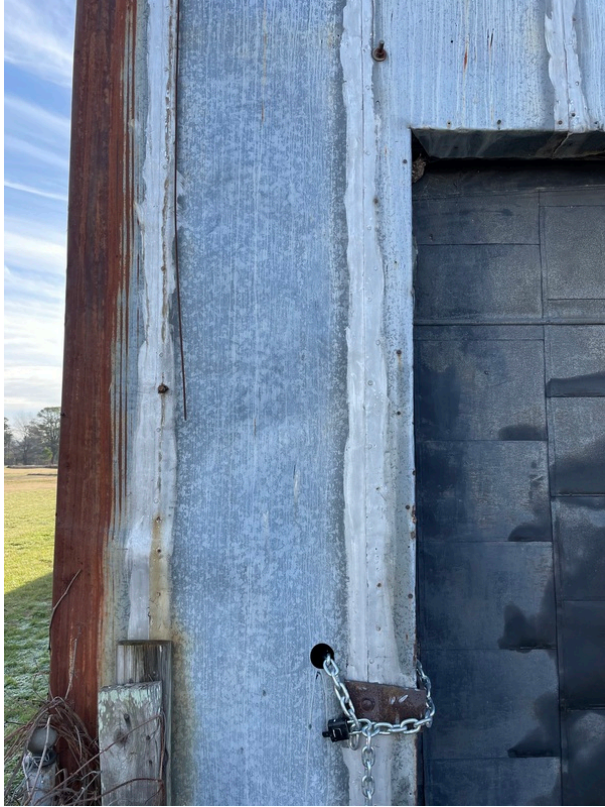
View of the asbestos-containing Silver Paint on Metal (HA 3-4)
