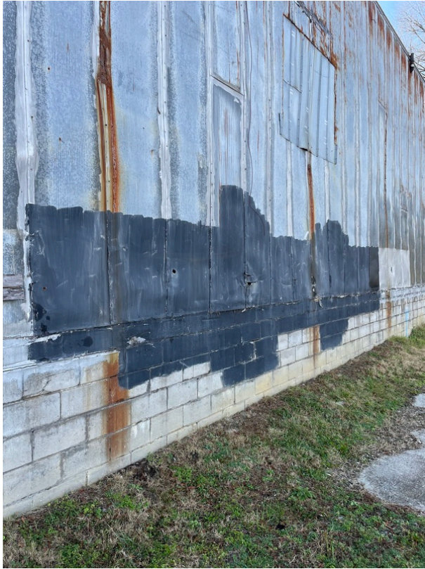
View of the asbestos-containing Grey/ Silver/Black Exterior CMU/Metal Surfacing (HA 3-8)
