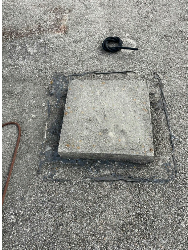
View of the asbestos-containing Black/Gray Penetration Tar (HA 1-4)
