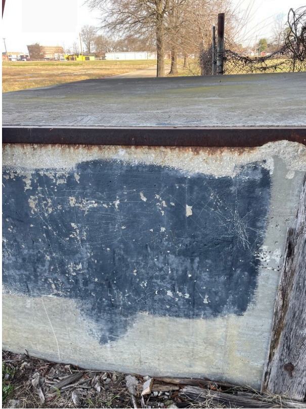
View of the asbestos-containing Beige/ Silver/Black Waterproofing (HA 3-6)
