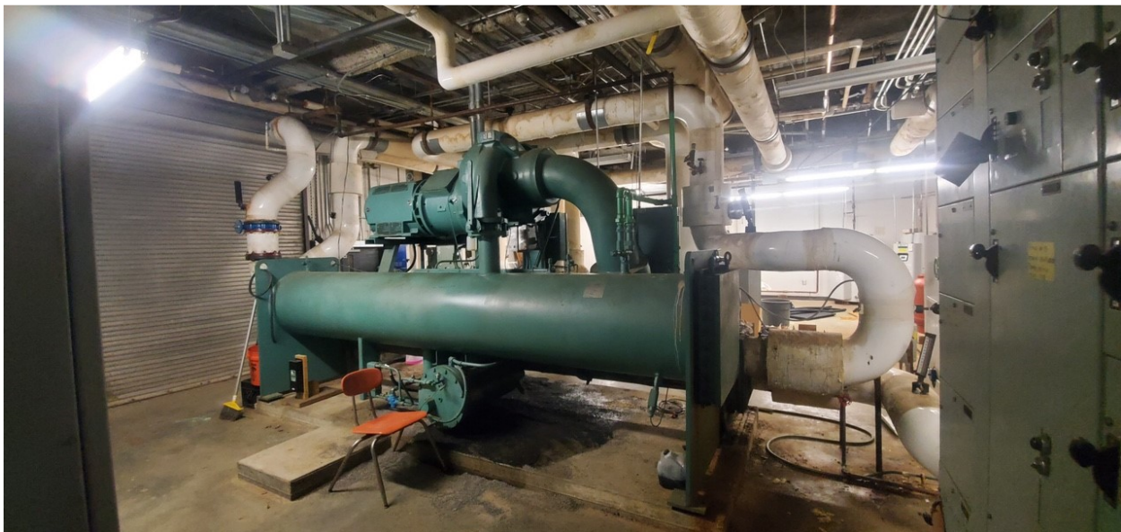
Different view of chiller. Note service door where chiller will be accessed for removal.
