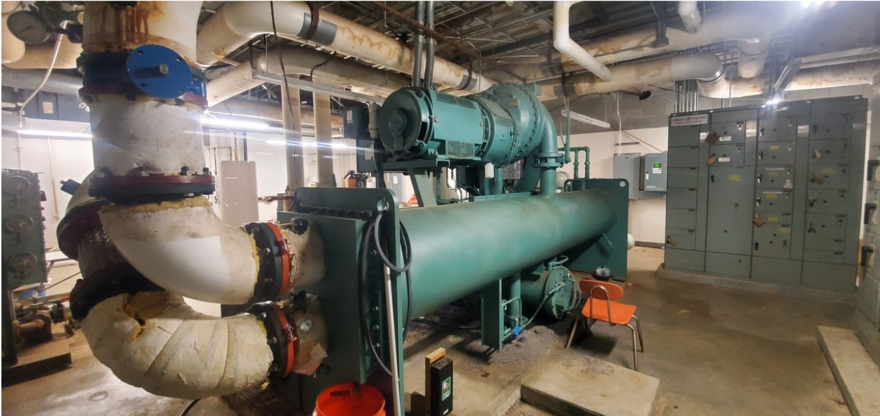
Piping connections Service Door End of Chiller
