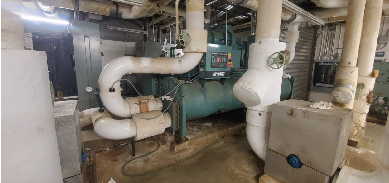
Piping connections – End of Chiller opposite the Service Door
