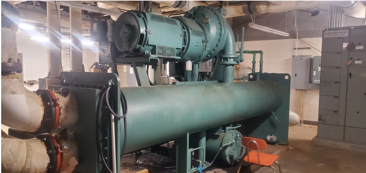
Existing chiller to be removed. Chiller is a York YKCCCCG4-CMD model.
