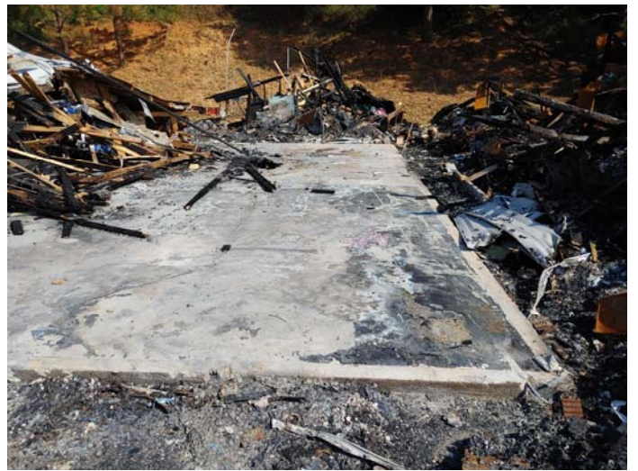
Photo 4 – Typical view of the burned remains of the house collapsed into a debris pile
