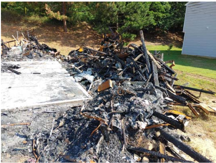
Photo 3 – Typical view of the burned remains of the house collapsed into a debris pile
