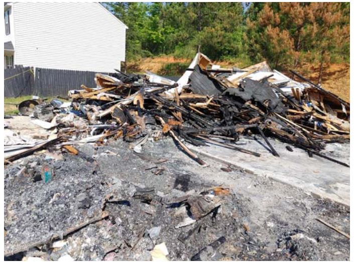
Photo 2 – Typical view of the burned remains of the house collapsed into a debris pile
