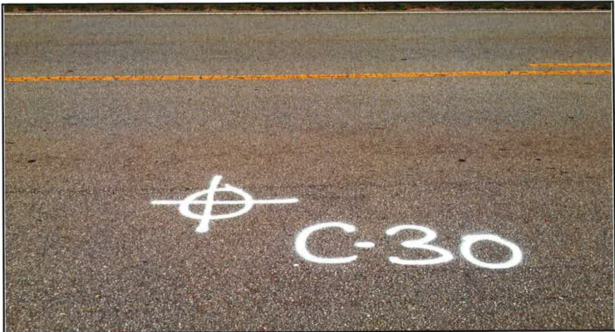
Photo 59: Minor alligator cracking, minor rutting and some weathering.
