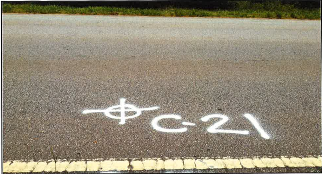
Photo 41: Rutting and weathering.
