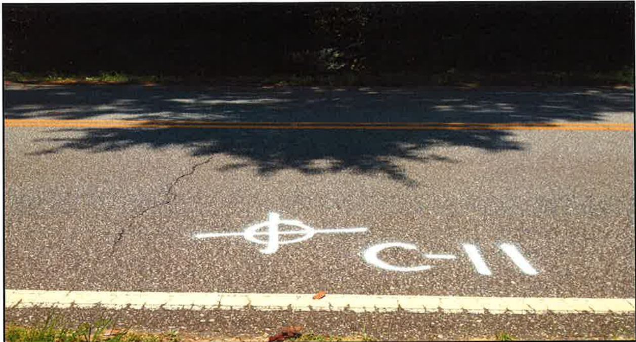
Photo 21: Transverse cracking and weathering.
