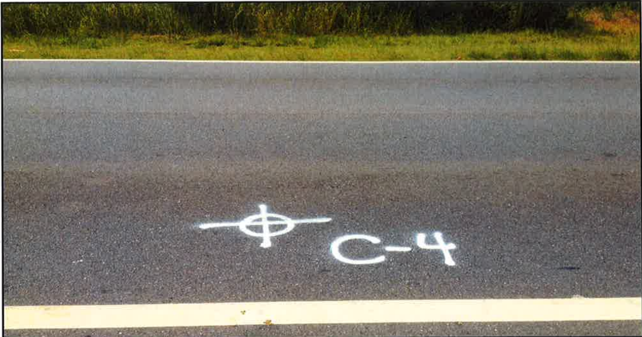
Photo 7: Pavement section looked good in the vicinity of core C-4 . Recently resurfaced.
