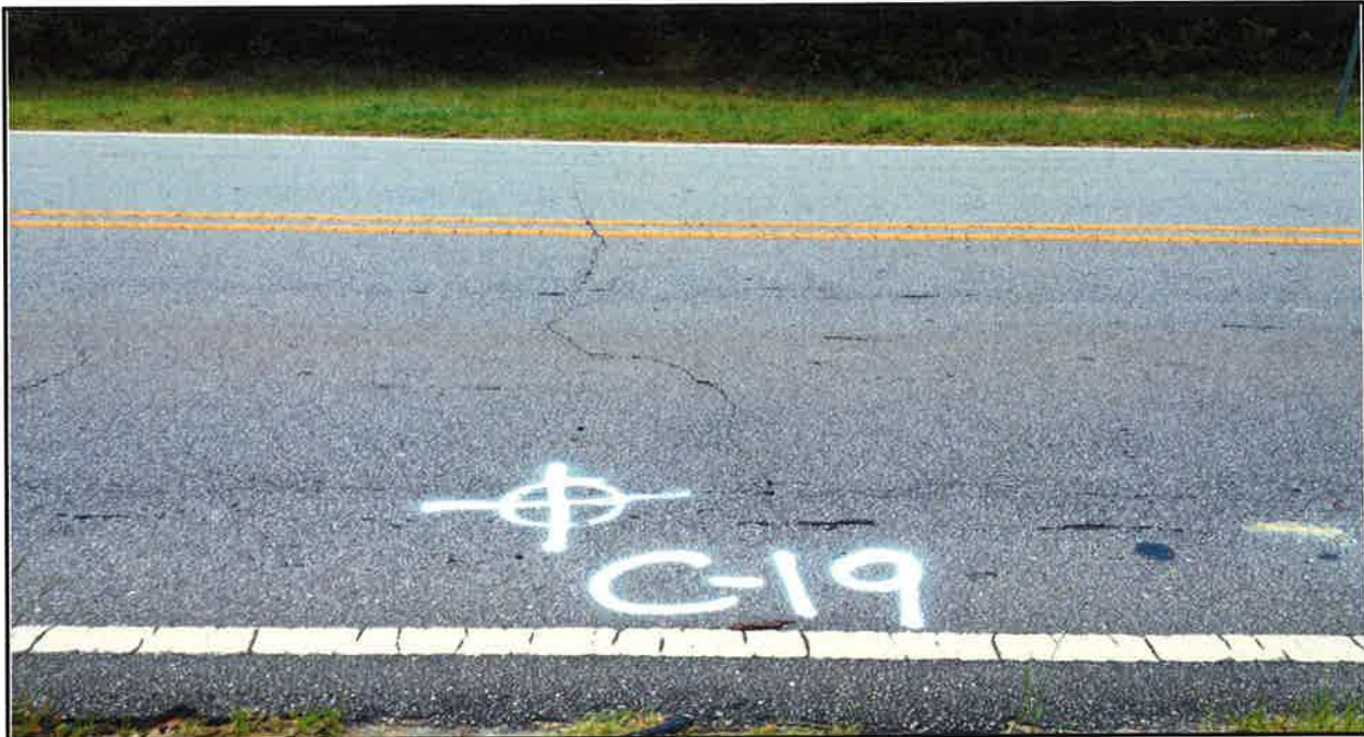
Photo 37: Block cracking, alligator cracking, rutting in wheel paths, weathering and raveling.
