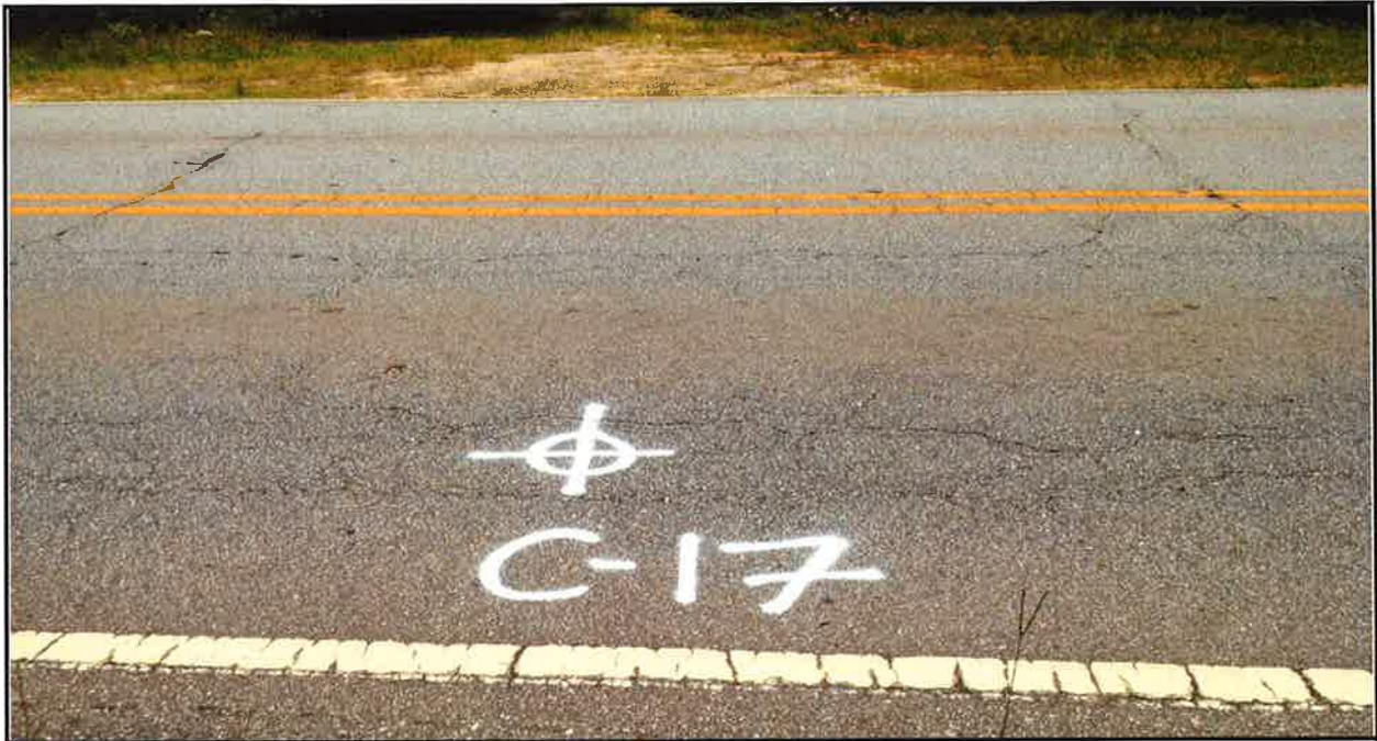
Photo 33 : Block cracking, longitudinal and transverse cracking, and rutting in wheel paths.
