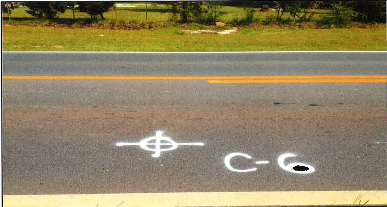
Photo 11: Pavement section looked good in the vicinity of core C-6 . Recently resurfaced.
