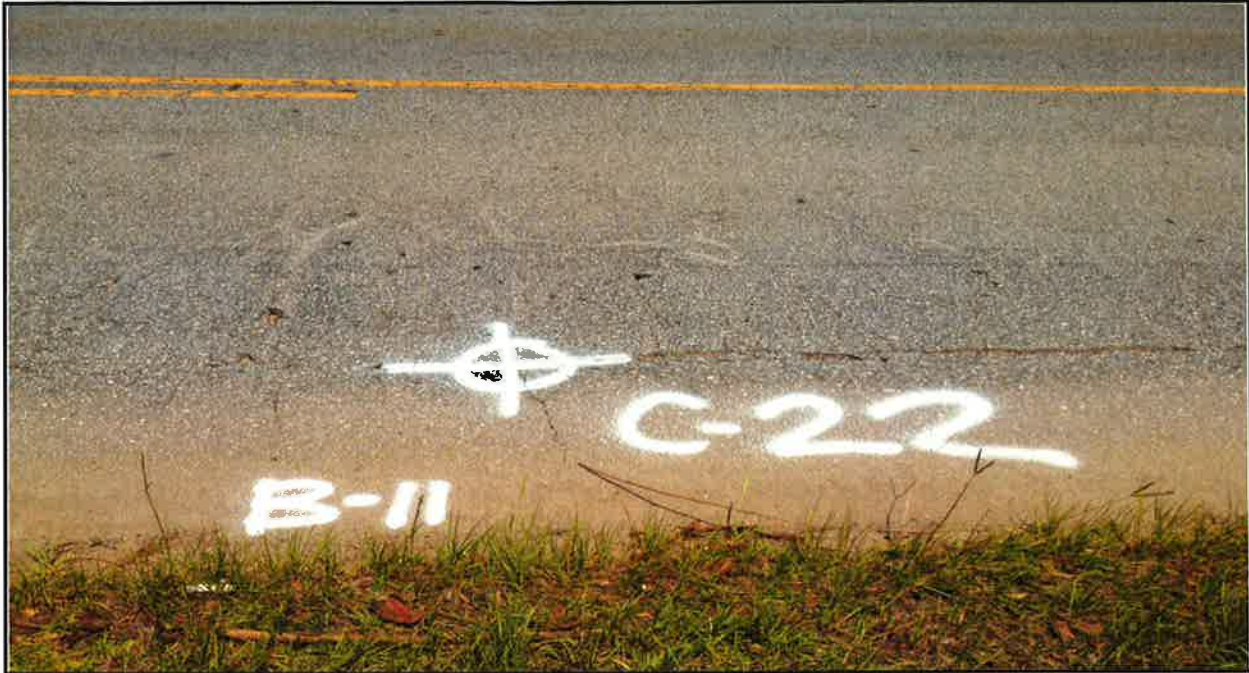
Photo 43: Alligator cracking, rutting, weathering, pumping of soil fines.
