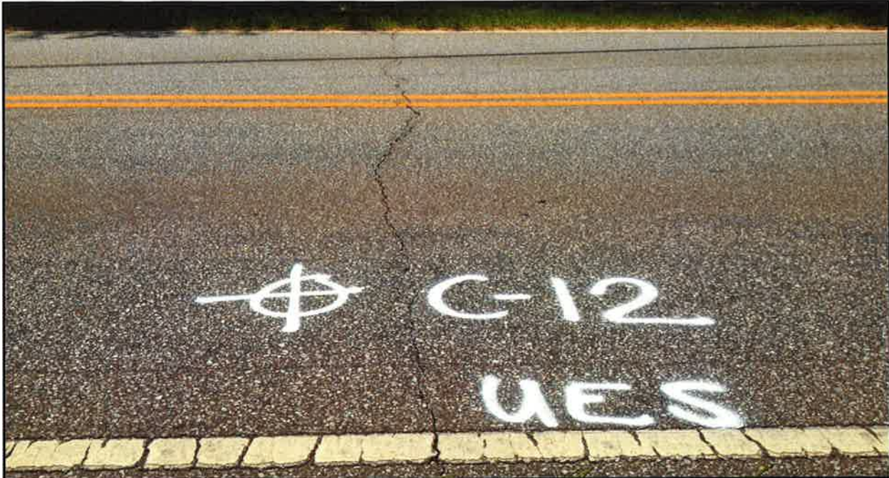
Photo 23: Transverse cracking, weathering and raveling.
