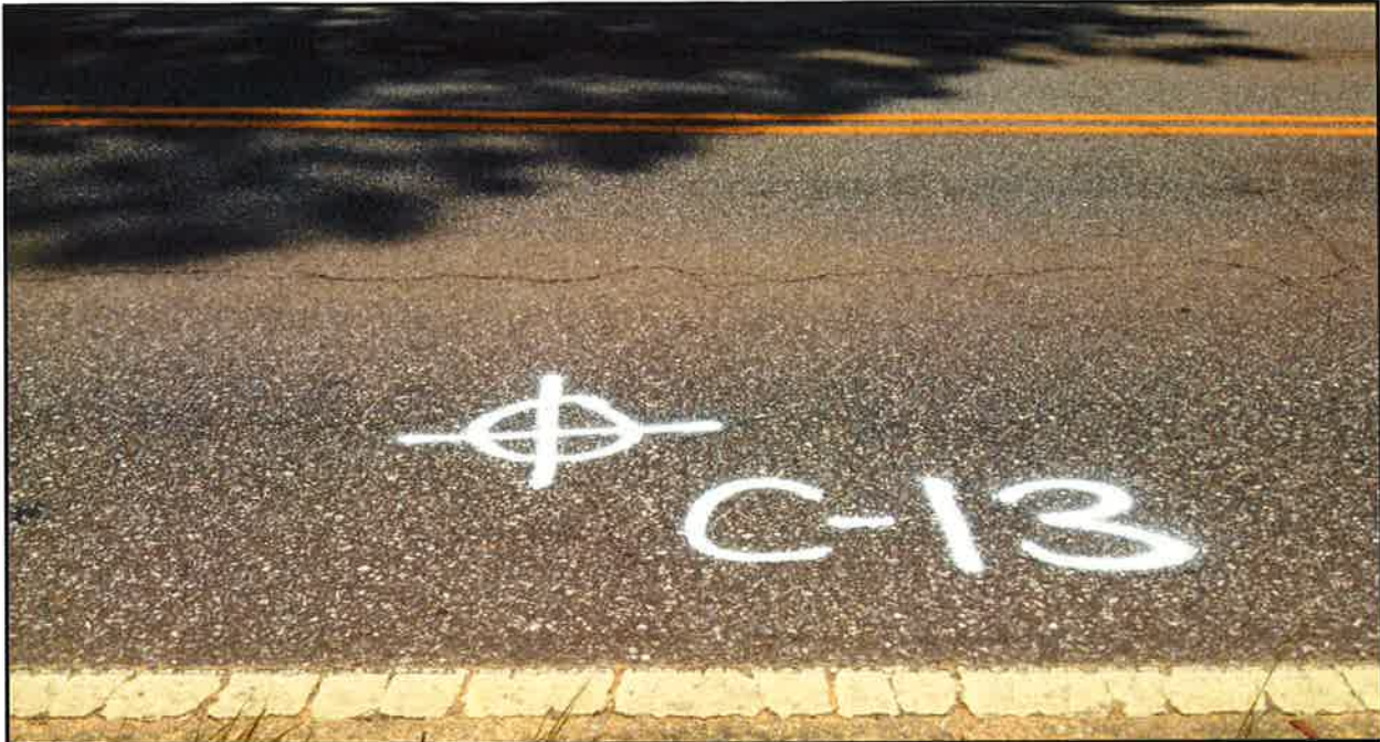
Photo 25: Longitudinal cracking, rutting in wheel paths, weathering and raveling.
