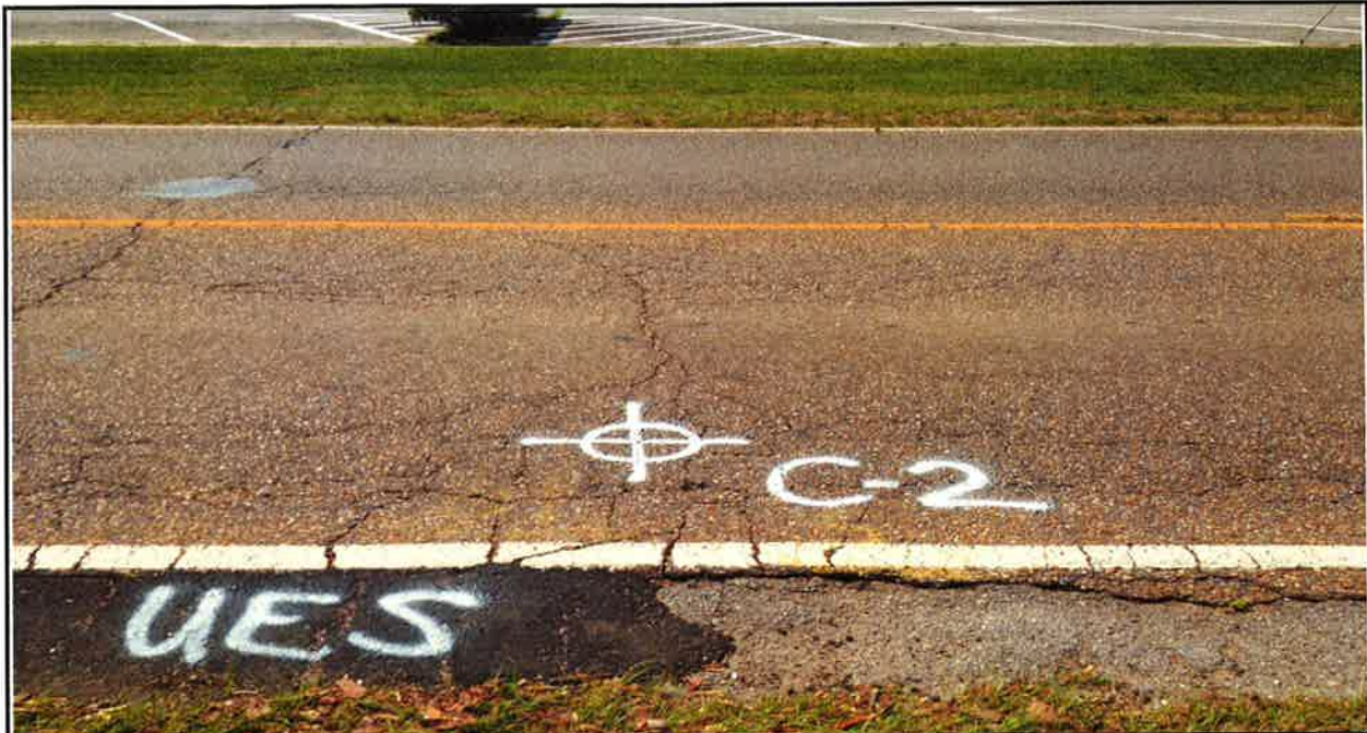
Photo 3: Patching, transverse cracking, alligator cracking, rutting in wheel paths, and weathering.
