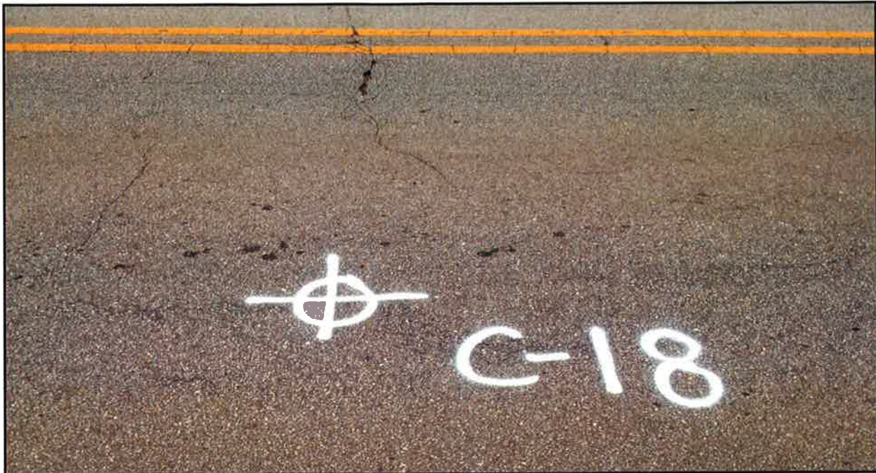
Photo 35: Alligator cracking, block cracking, weathering and raveling.
