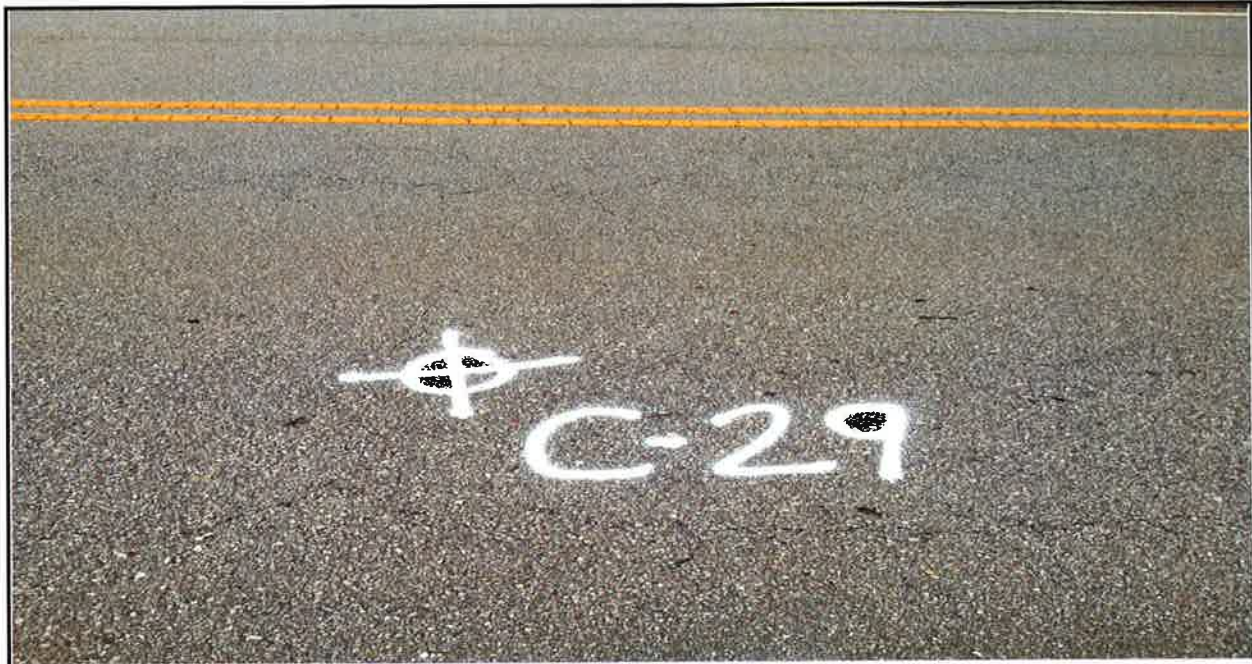
Photo 57: Minor alligator cracking, minor rutting and some weathering.
