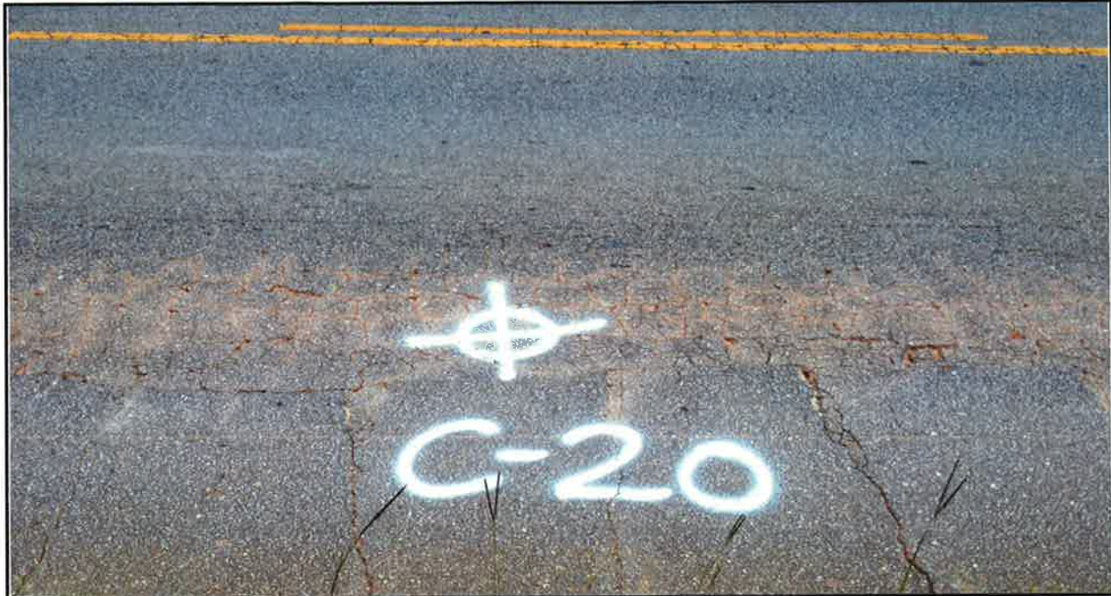
Photo 39: Alligator cracking, rutting in wheel pathes, block cracking and pumping of soil fines.
