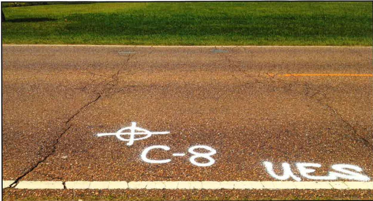
Photo 15: Block cracking, alligator cracking, and rutting in wheel paths.
