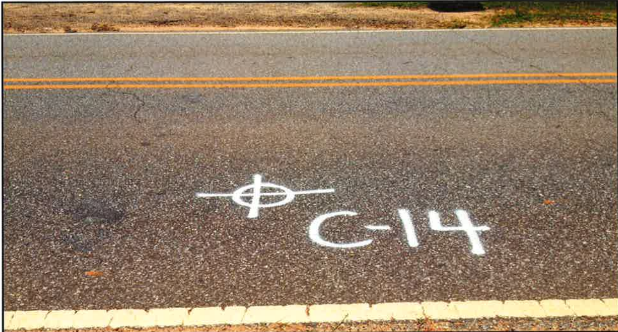
Photo 27: Transverse cracking, weathering and raveling.
