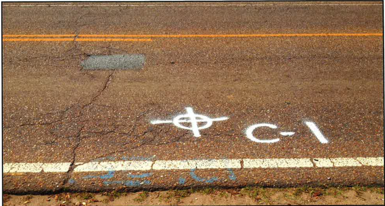
Photo 1: Patching, rutting in wheel paths, alligator cracking and weathering.
