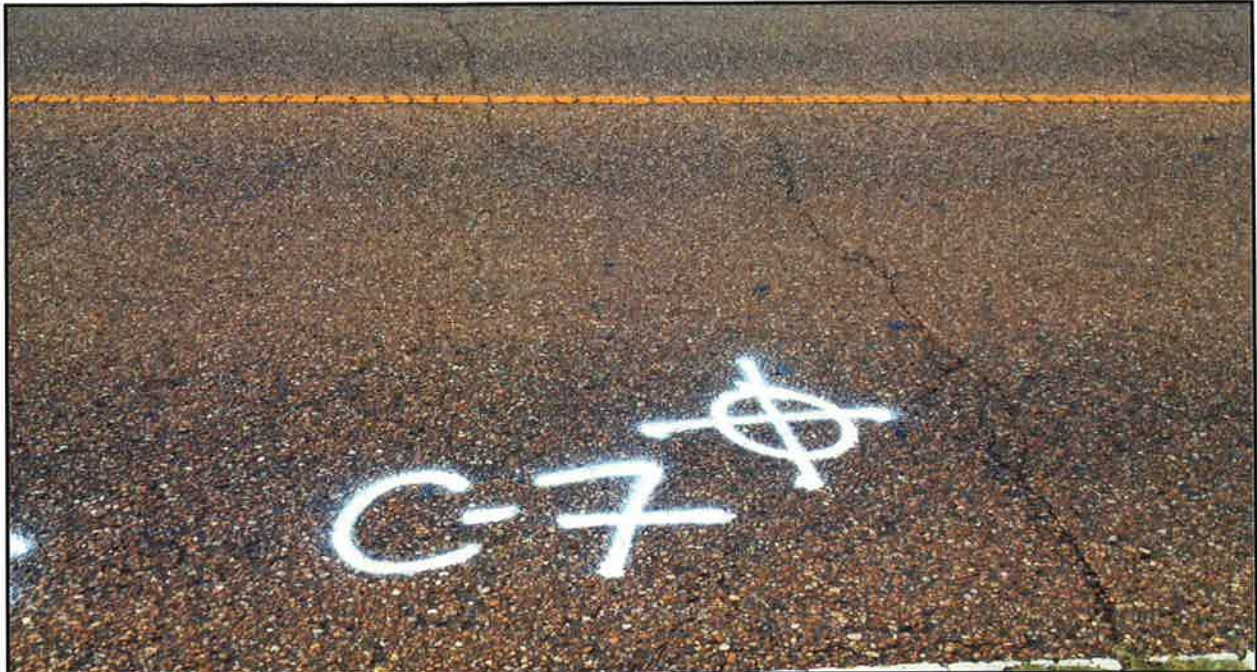
Photo 13: Block cracking and weathering.
