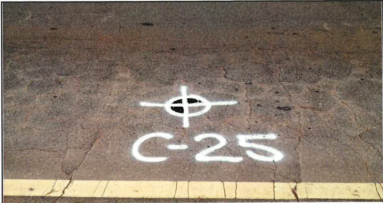
Photo 49: Alligator cracking, rutting, weathering, pumping of soil fines.
