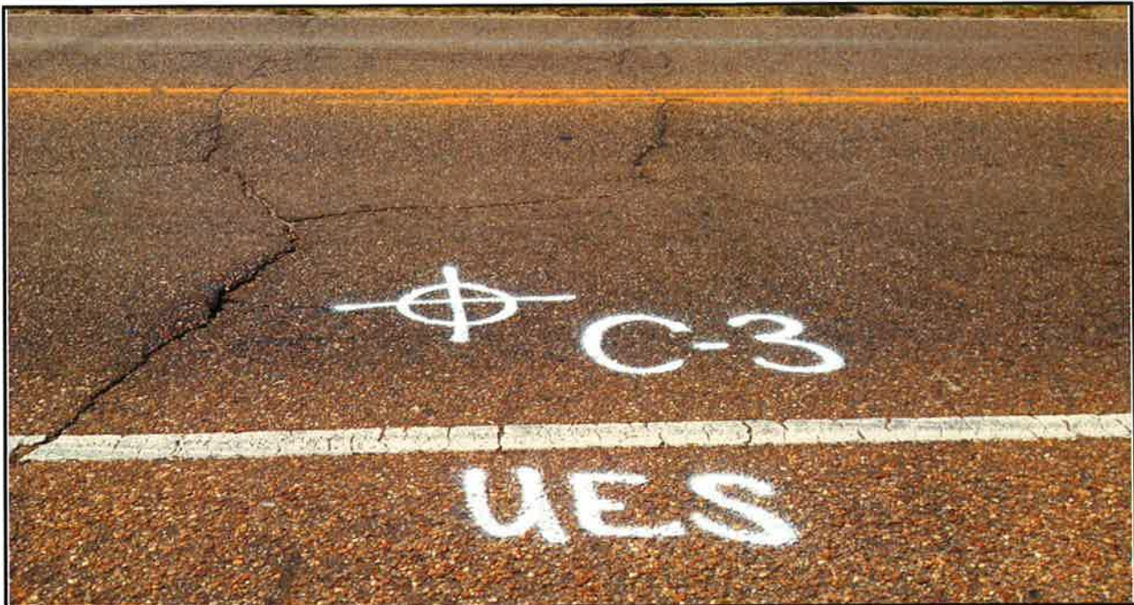
Photo 5: Block cracking, longitudinal and transverse cracking, rutting in wheel paths and weathering.
