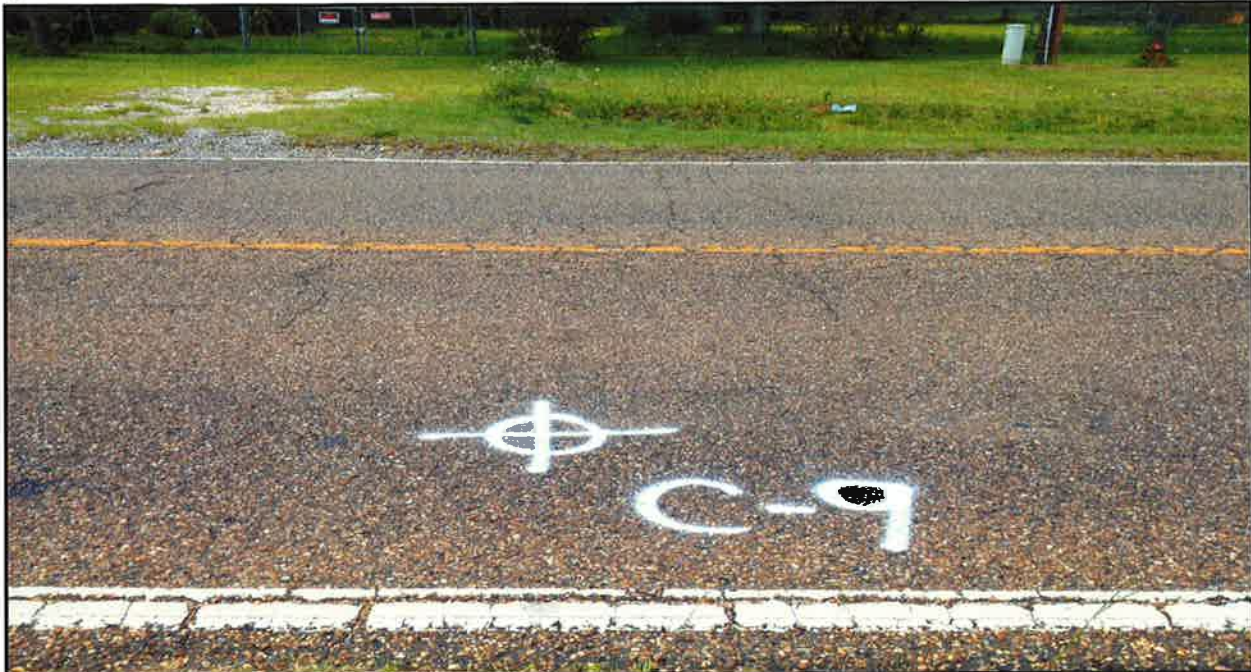
Photo 17: Block cracking, alligator cracking, rutting in wheel paths, and weathering.
