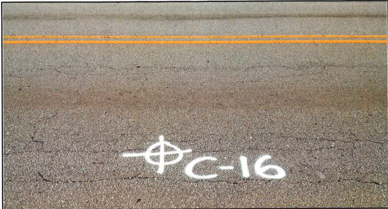
Photo 31: Block cracking, alligator cracking, rutting in wheel paths, and weathering.
