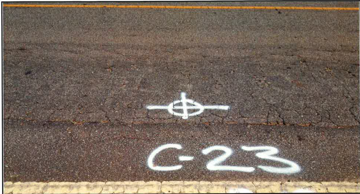
Photo 45: Alligator cracking, rutting, weathering, pumping of soil fines.
