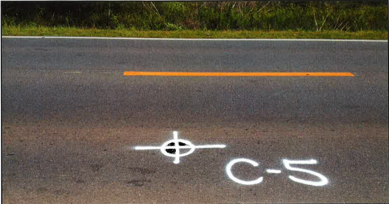
Photo 9: Pavement section looked good in the vicinity of core C-5 . Recently resurfaced.
