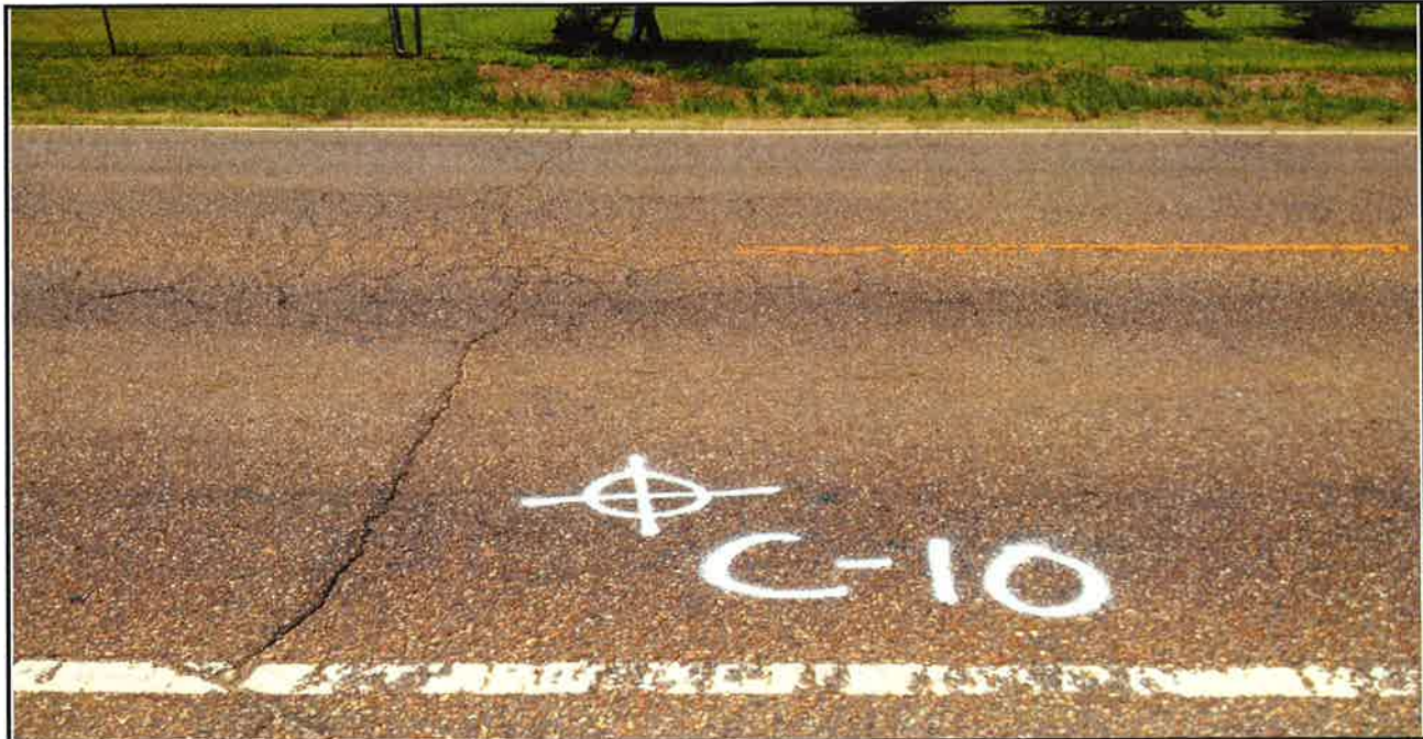
Photo 19: Block cracking, transverse cracking, minor rutting in wheel paths, and weathering.
