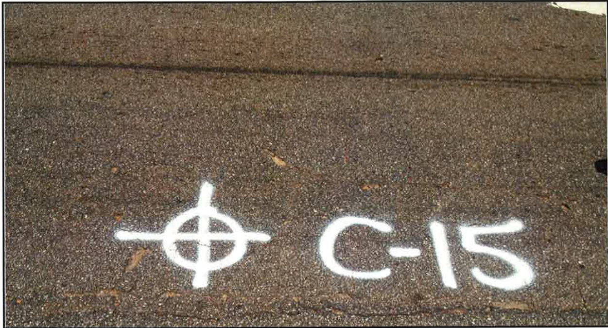
Photo 29: Alligator cracking, longitudinal cracking, rutting in wheel paths, and weathering and raveling.
