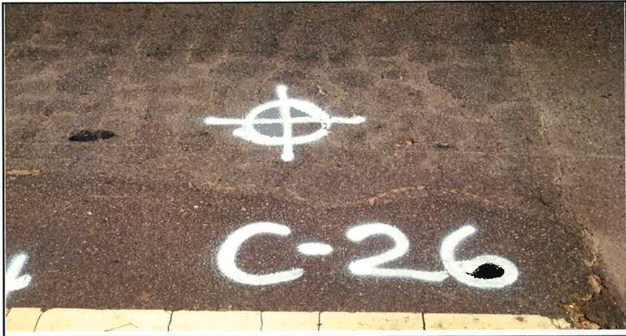
Photo 51: Alligator cracking, rutting, weathering, pumping of soil fines.
