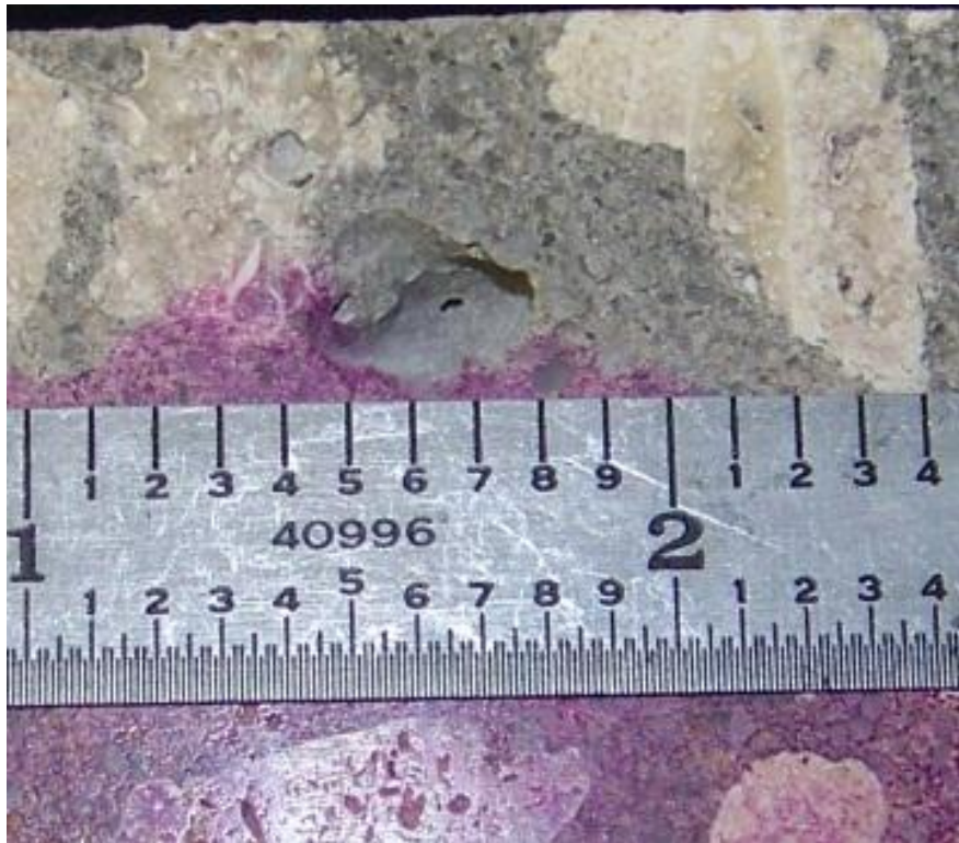
Photo 8 – Sample 3A – large entrapped air void
