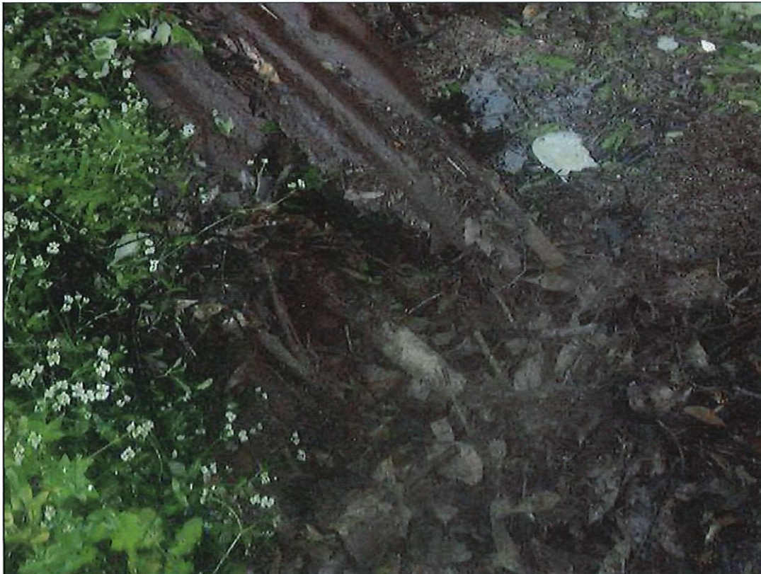
SECTION LOSS LINE 2, FROM SOUTH END BACK 2.0' (PAR)
