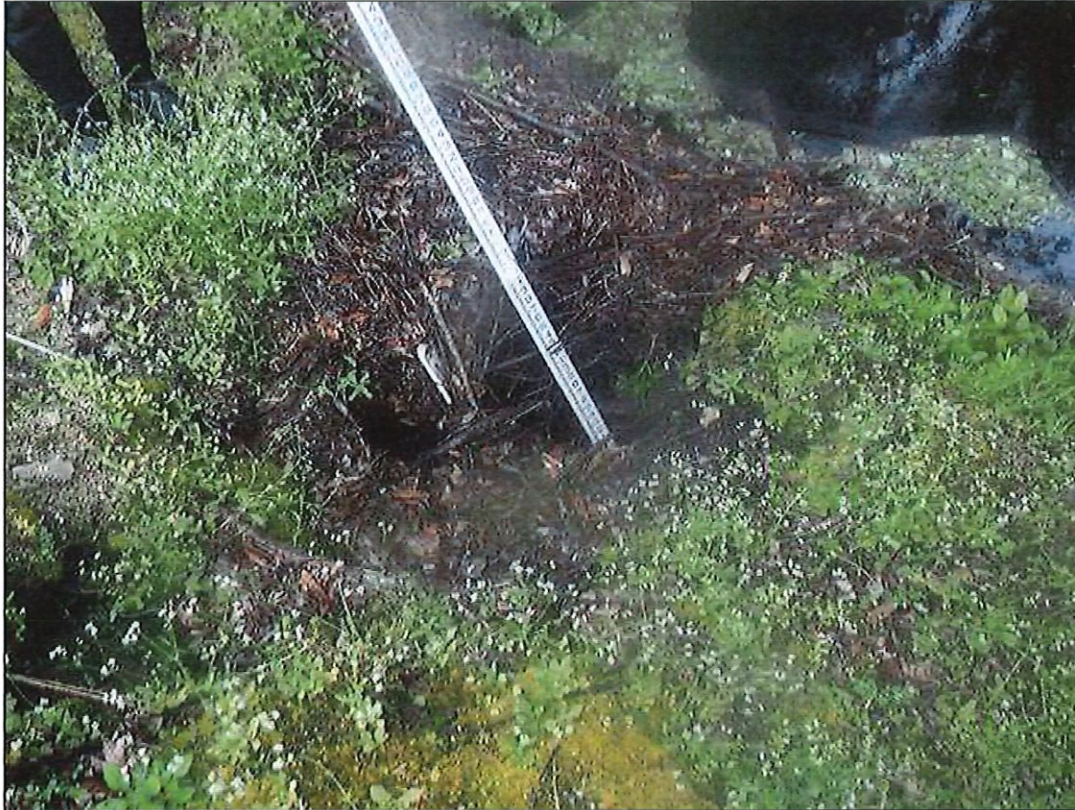
LINE 3, SOUTH END COLLAPSED FROM THE END BACK 6.0' (PAR)
