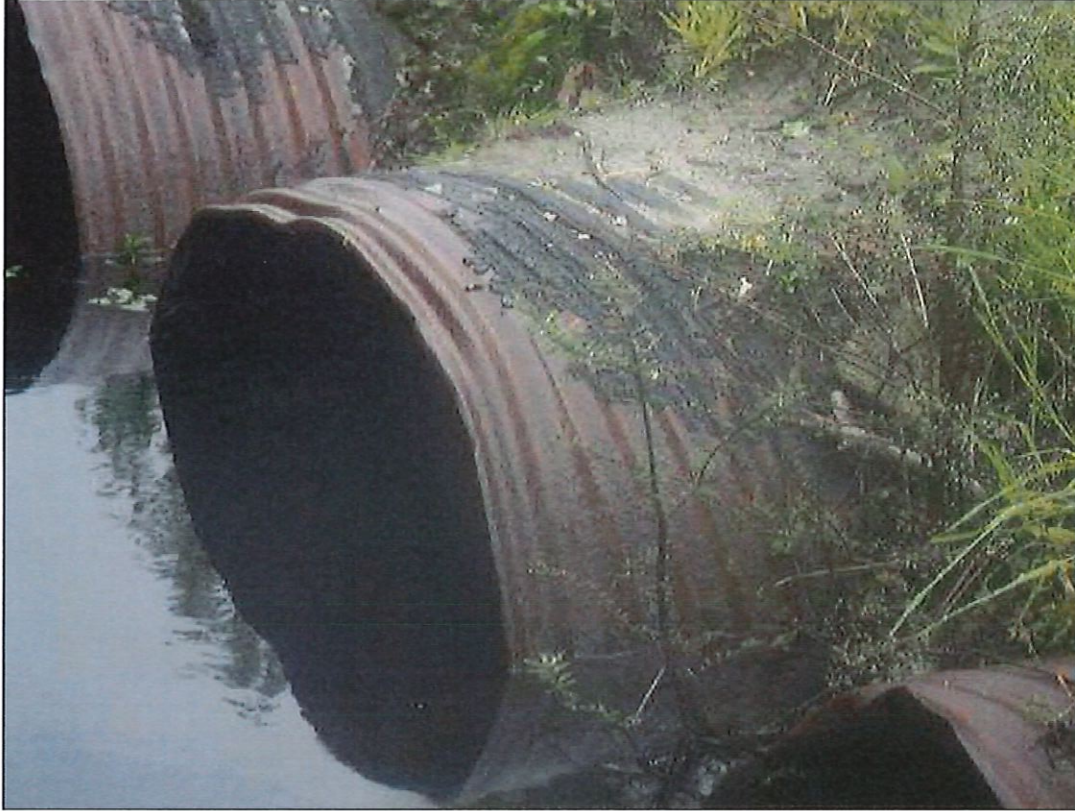
RUST AT EXPOSED PIPE ENDS
