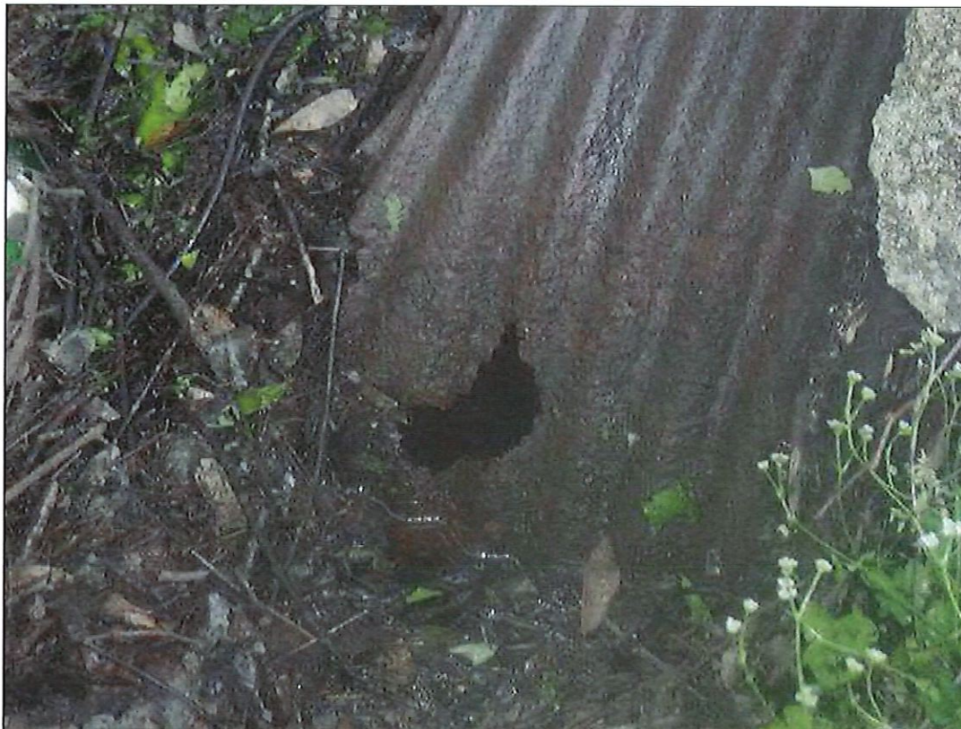
SECTION LOSS LINE 1, FROM SOUTH END BACK 1.0' (PAR)
