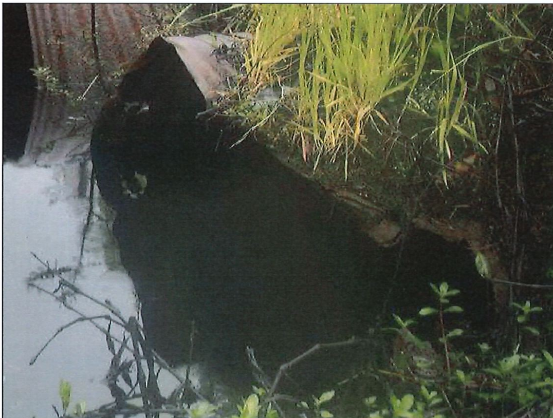
SECTION LOSS LINE 1, FROM NORTH END BACK 1.0' (PAR)
