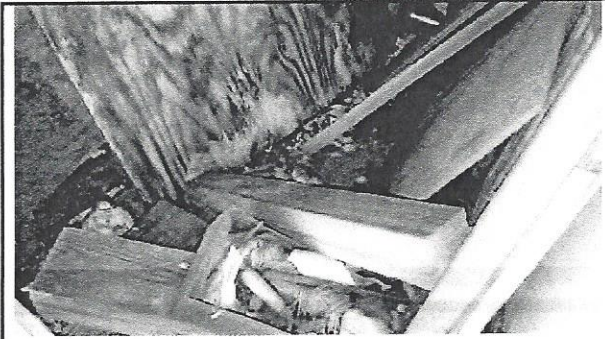
Picture 7 – Room Interior, excessive clutter and structural damage from ceiling collapse
