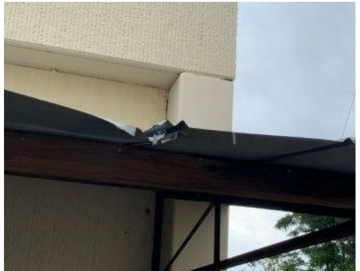
V-Crimp roof - Wind blown debris damage
