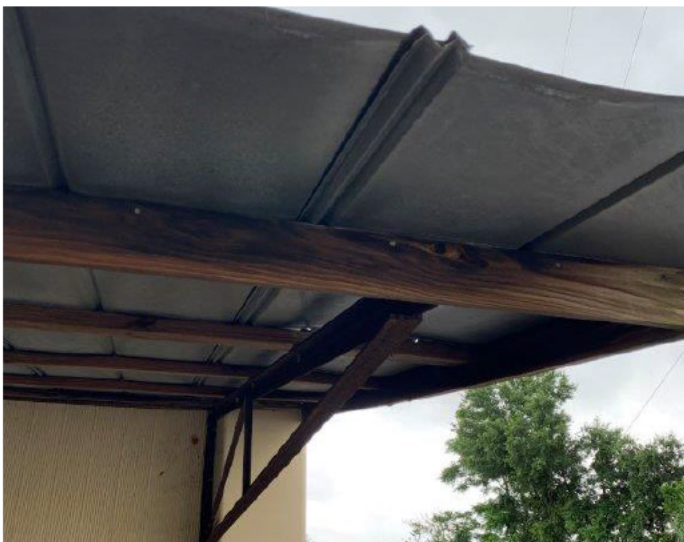
V-Crimp Roof - Fasteners pulled through and torn metal
