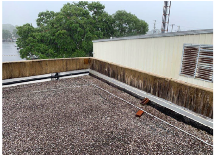
Roof Perimeter - Termination bar and coping flashing disconnected
