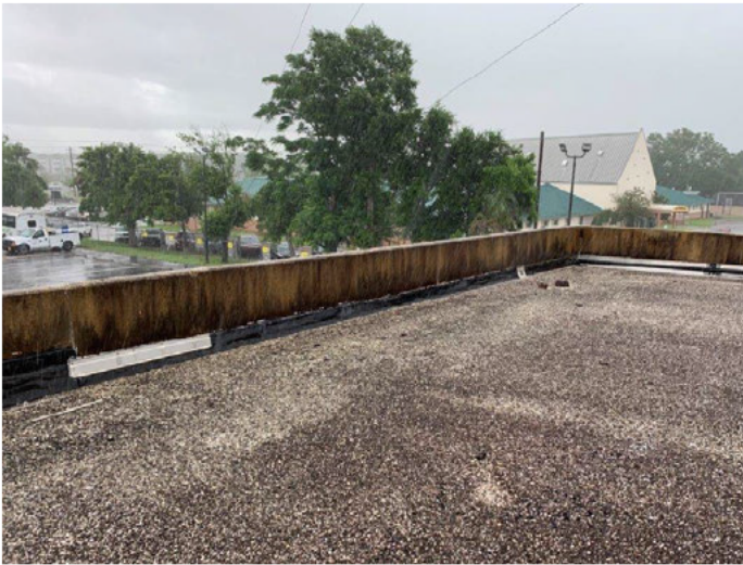
Roof Perimeter - Termination bar and coping flashing disconnected
