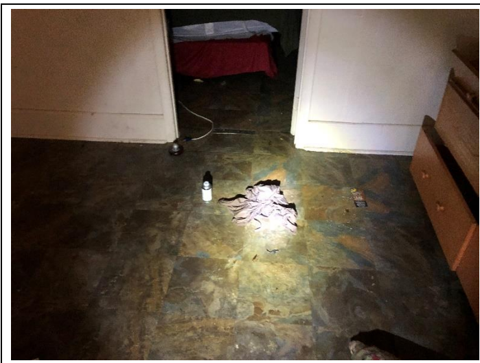
2. 1375 32nd St - Gray Vinyl Floor Tile & Black Mastic (Unit A Living Room Floor): HSA 21.
