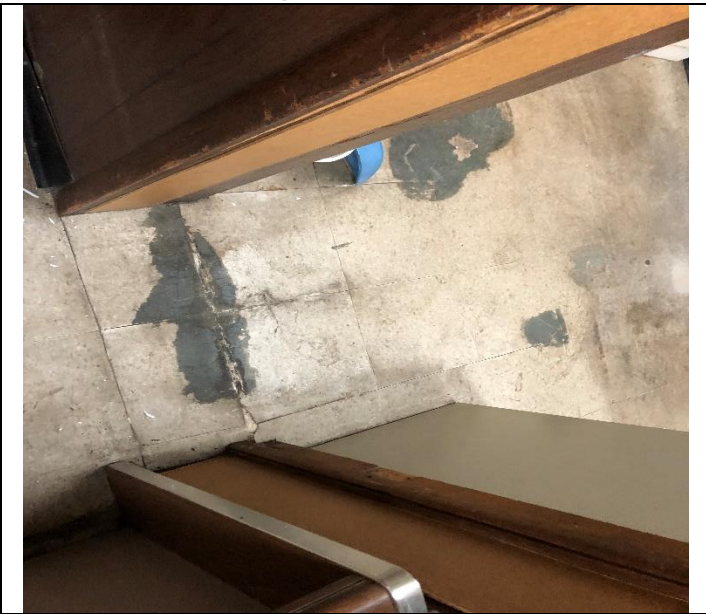
21. 3136-3146 US 1 - Black Mastic (Behind Office Wood Paneling): HSA 51.
