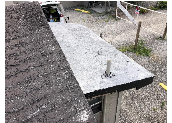
8. 1385 32nd St., Apts A & B - Black Tar & Silver Coating Material (Unit A & B Roof Overhang & Stacks): HSA 7.
