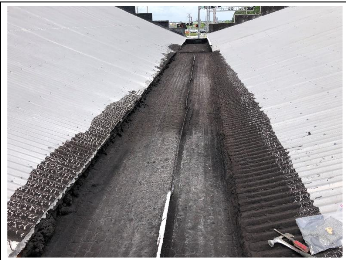
17. 3136-3146 US 1 - Black Flashing & Silver Coating Material (South Roof Seams at Metal and Gravel Roof): HSA 37.
