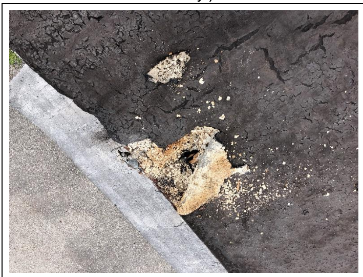
5. 1385 32nd St., Apts A & B - Black Tar (Center Roof Btwn. Pitches): HSA 3.
