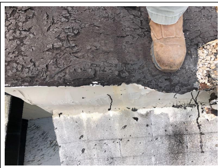
6. 1385 32nd St., Apts A & B - Black Tar (Roof Seams Under Eaves): HSA 4.
