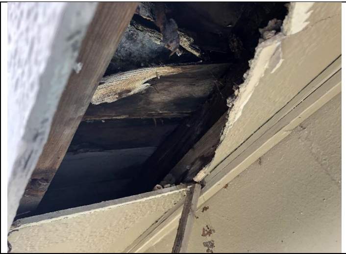
7. 1385 32nd St., Apts A & B - Black Tar & Silver Coating Material (Unit A Front Eaves): HSA 5.
