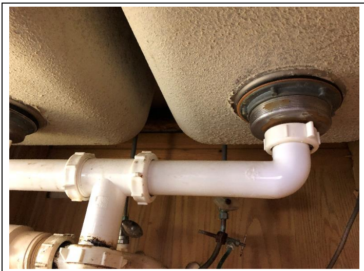
1. 1375 32nd St - White Sink Coating (Unit B): HSA 12.
