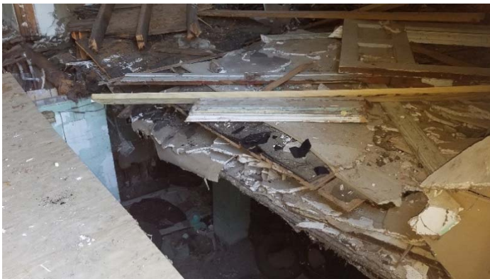
Photo 3 – Collapsed roof and ceiling systems.
