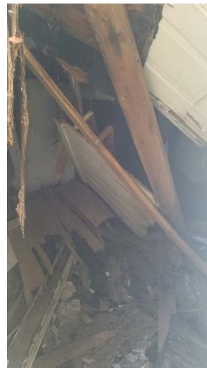
Photo 10 – Basement collapsed ceiling.
