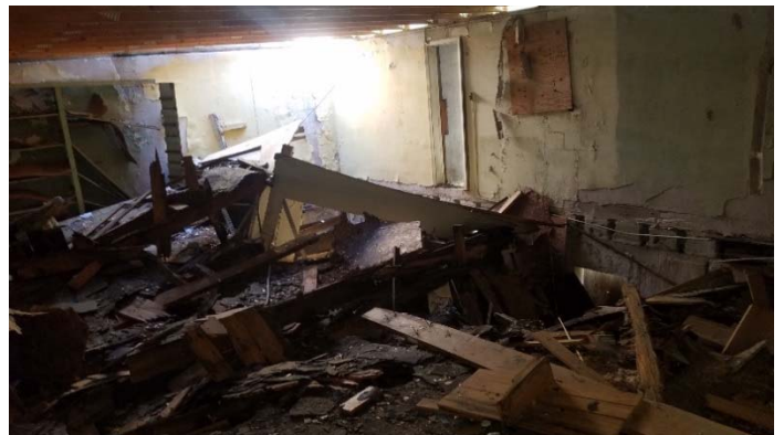
Photo 4 – Collapsed roof and ceiling systems.
