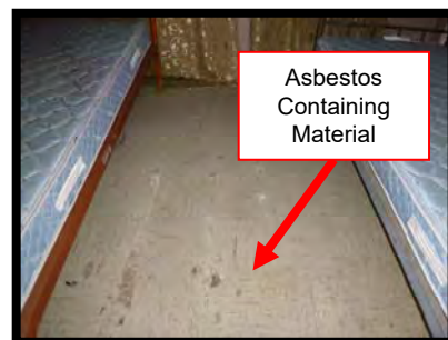
6: View of HA-01 – White Floor Tile.
