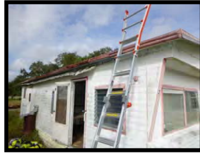
2: Trailer Unit B.
