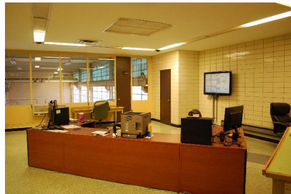
Figure 3.27 SCADA Control Room
