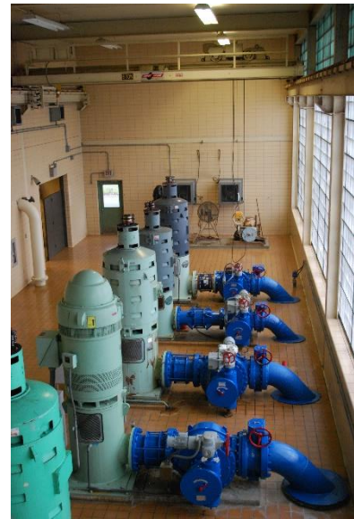
Figure 3.14 High Service Pumps
