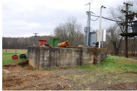
Figure 3.2 Well #1 Valve Vault
