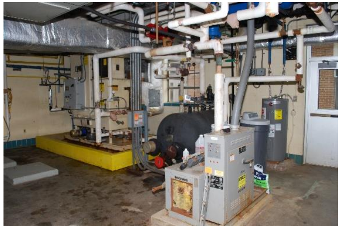
Figure 3.25 Mechanical Room with Kathabar Dehumidifier
