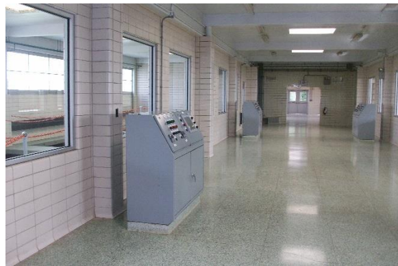
Figure 3.21 2nd Floor Filter Gallery
