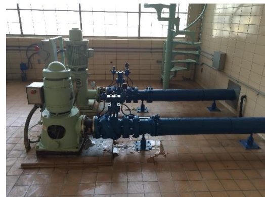
Figure 3.10 Backwash Reservoir Fill Pumps
