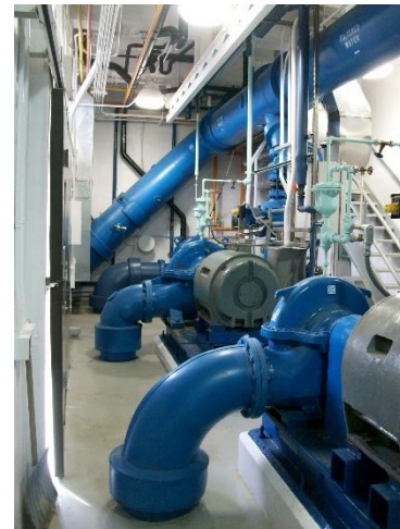
Figure 3.29 Northwest WTP High Service Pump Room
