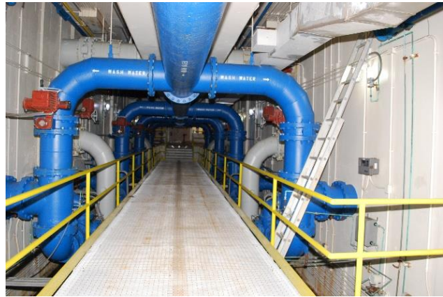
Figure 3.11 Filter Pipe Gallery
