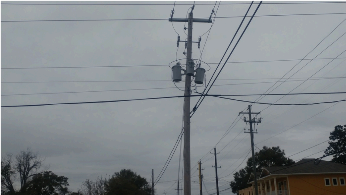
Photo 22: VIEW OF NORTH ADJOINING PROPERTY, POLE-MOUNTED TRANSFORMER.
