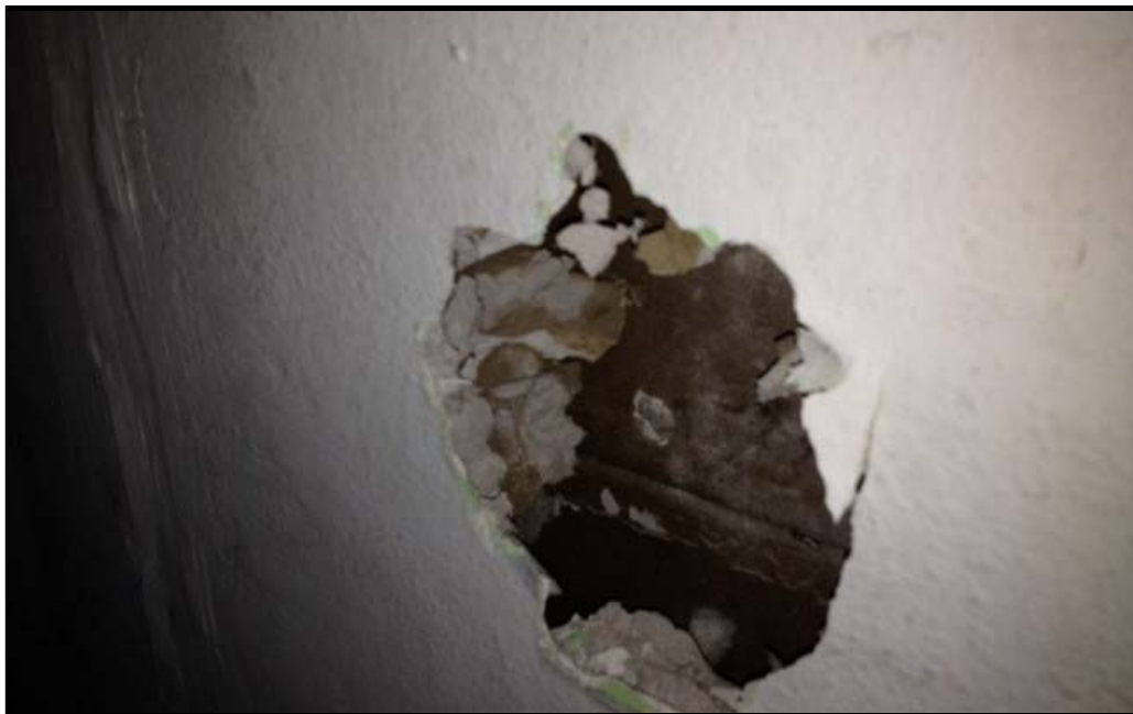
Photo 6: Drywall & Associated Joint Compound.
