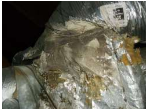
HOMOGENEOUS AREA 04 HVAC DUCT MASTIC (WHITE)
