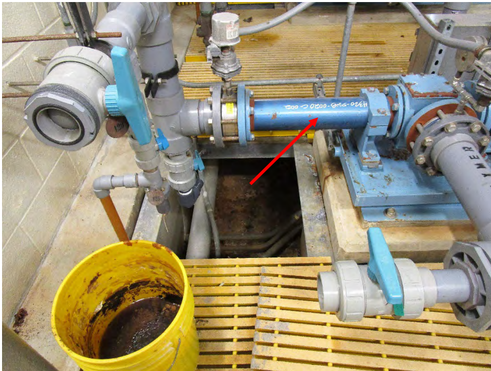
Photo A-36. Polymer Feed Pumps
