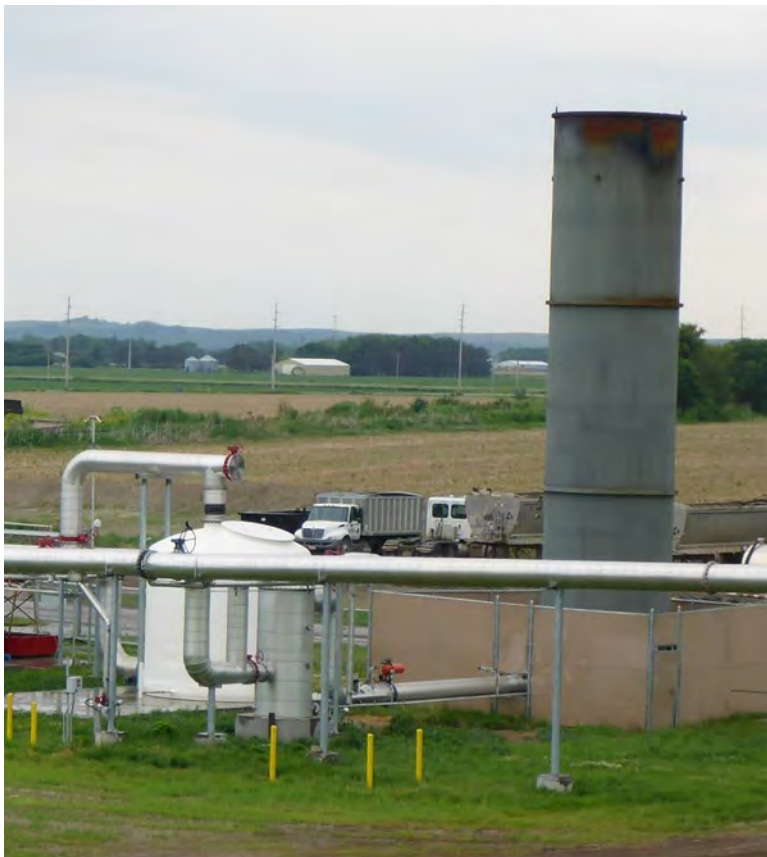
Figure 4. Enclosed Waste Gas Flare
