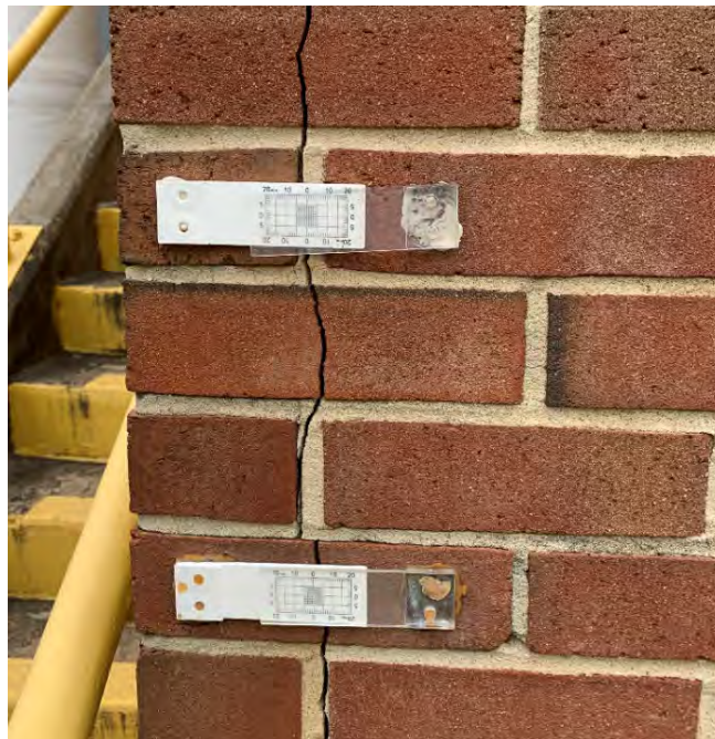
Figure 11. Structural Damage at the DAFT
