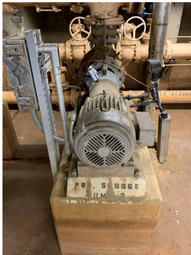
Figure 6. Primary Solids Pump
