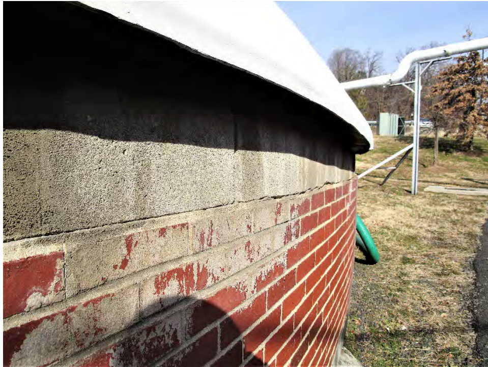
Photo A-17. Cement Bleeding
