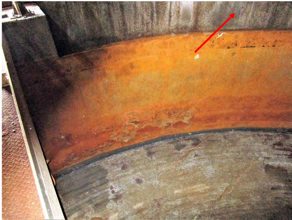
Photo A-7. Undetermined Peeling
