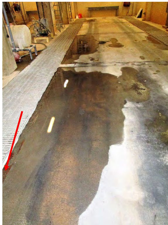
Photo A-38. Truck Scale Ponding, Edge Corrosion
