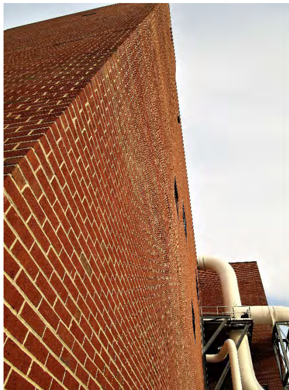
Photo A-43. Joint Damage
