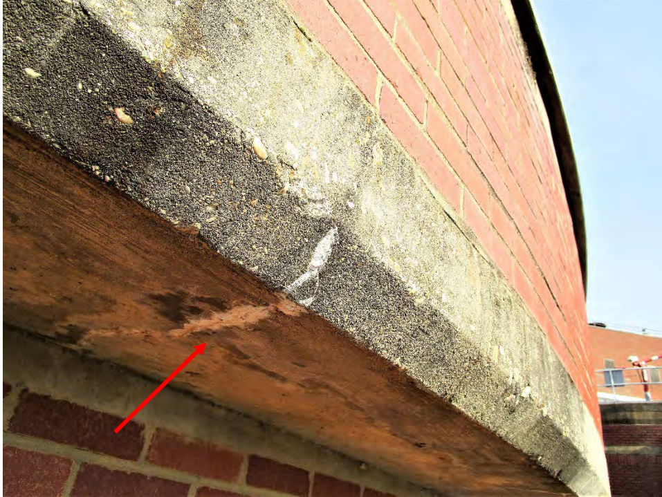
Photo A-15. Self Healed Dry Crack
