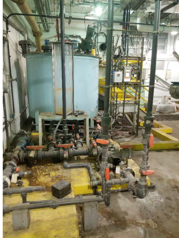
Figure 10. DAFT Polymer Mix Tank
