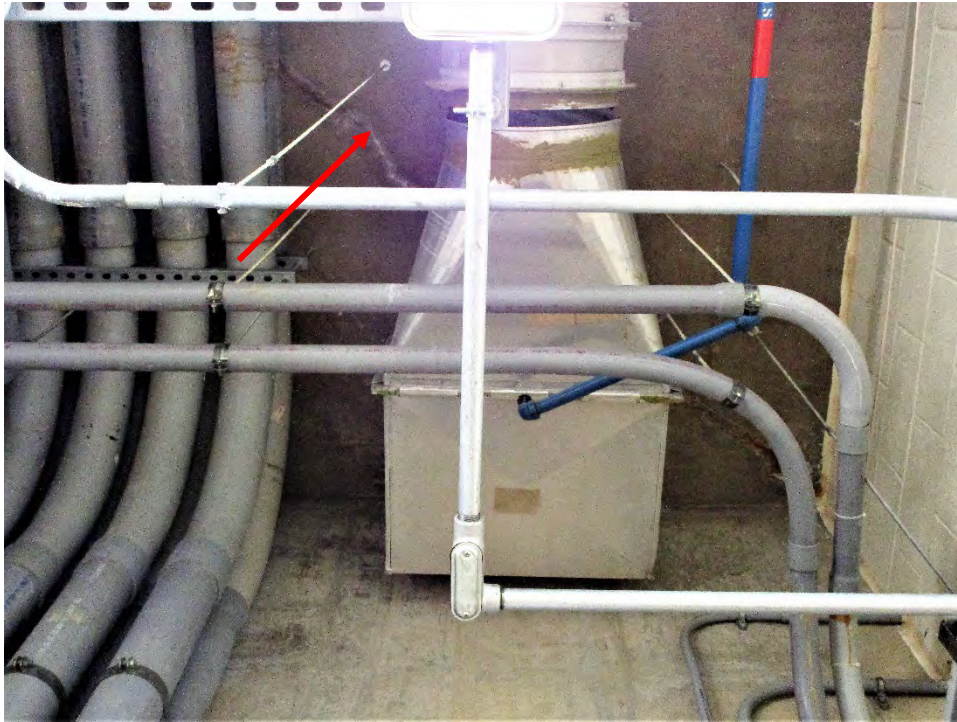
Photo A-35. MCC Ceiling Cracks
