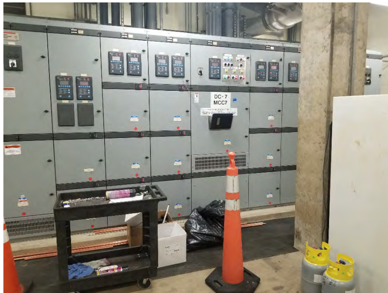
Figure 16. DC-7 Switchgear in the Dewatering Building
