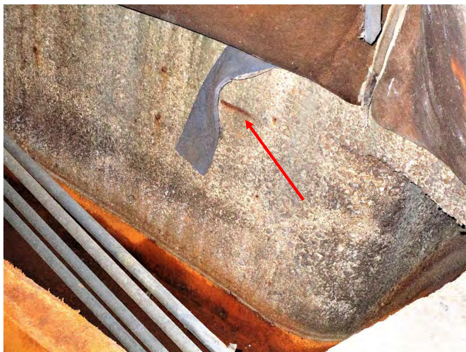
Photo A-2. Paste Loss Rebar
