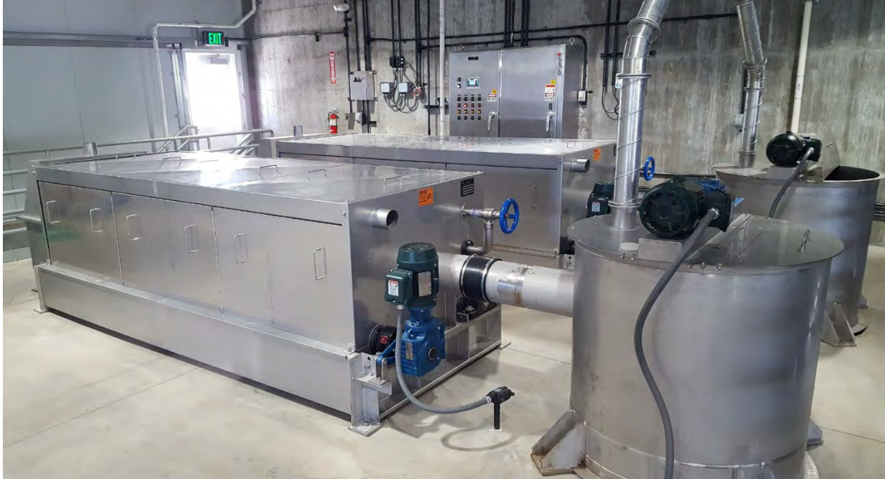
Figure 7. RDT and Floc Tank
