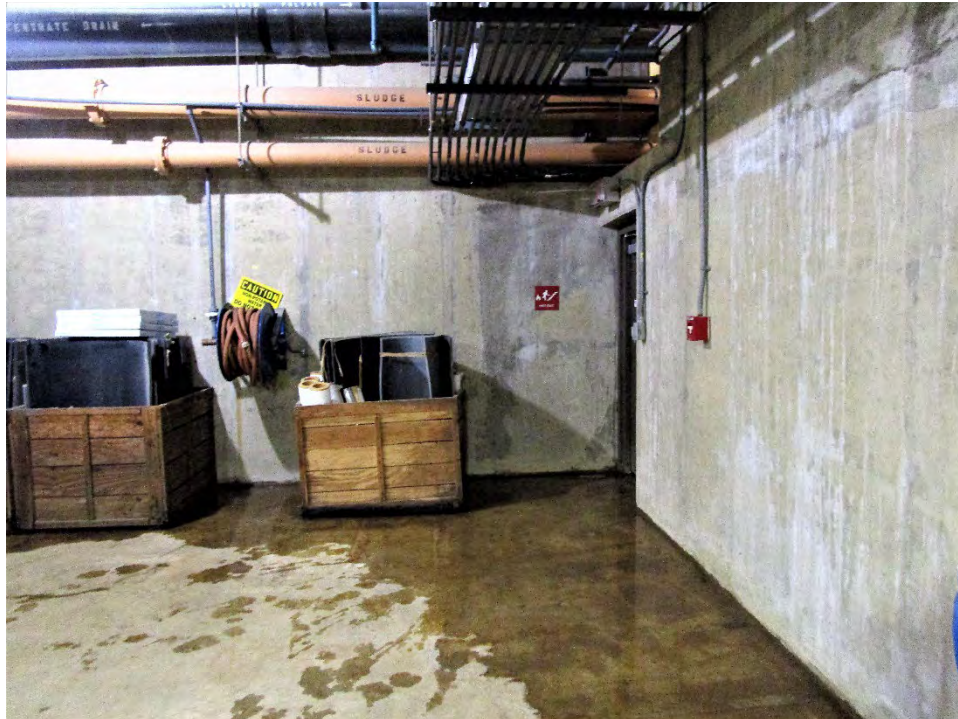
Photo A-32. Water in Link
