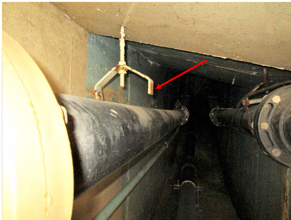
Photo A-24. Pipe Support Deficiency
