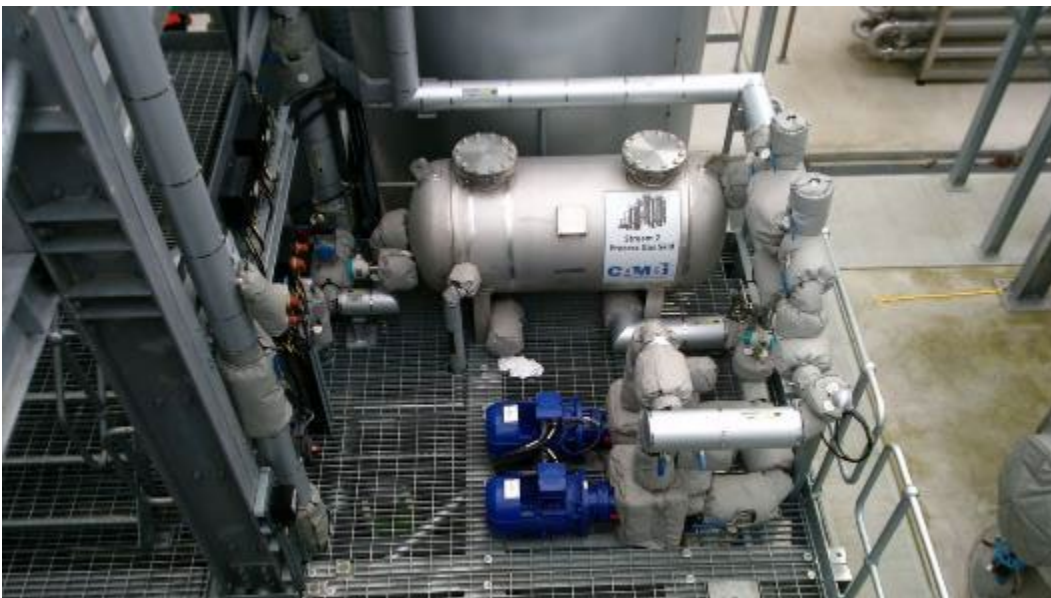
Figure 9-2. Process Gas Skid
