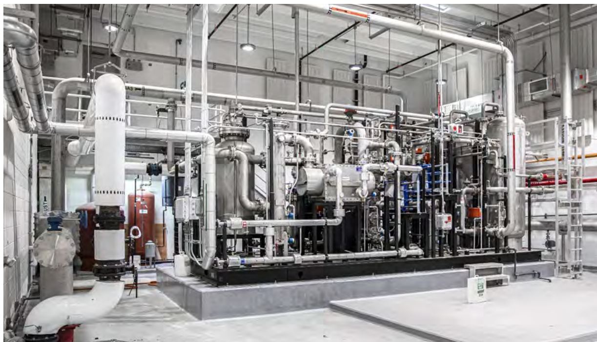
Figure 10. Typical Membrane Treatment Installation
