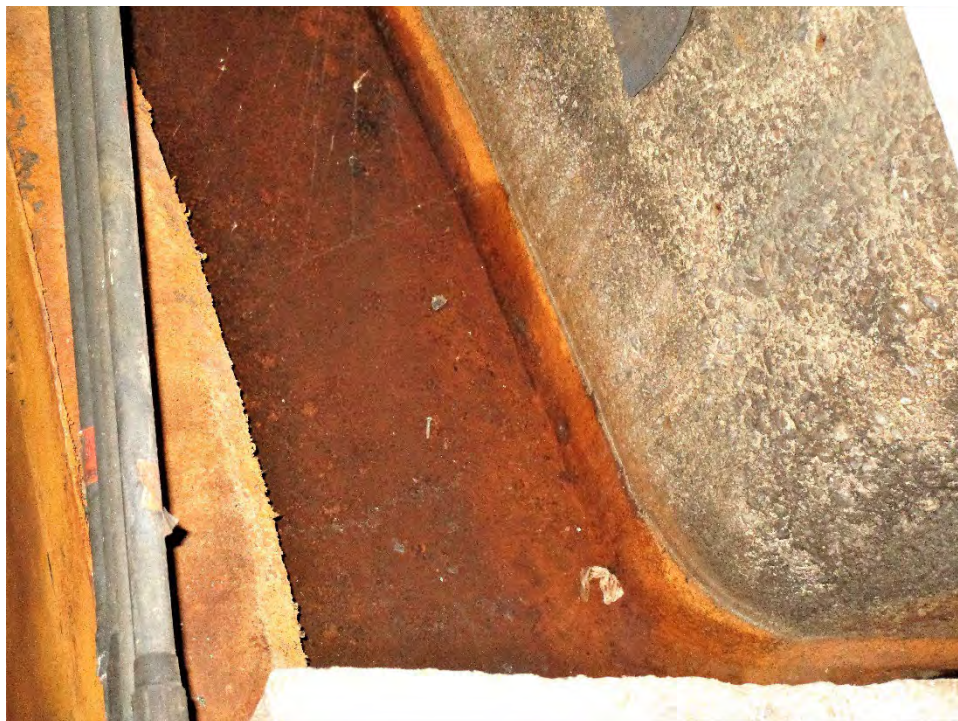
Photo A-3. Ferric Discoloration
