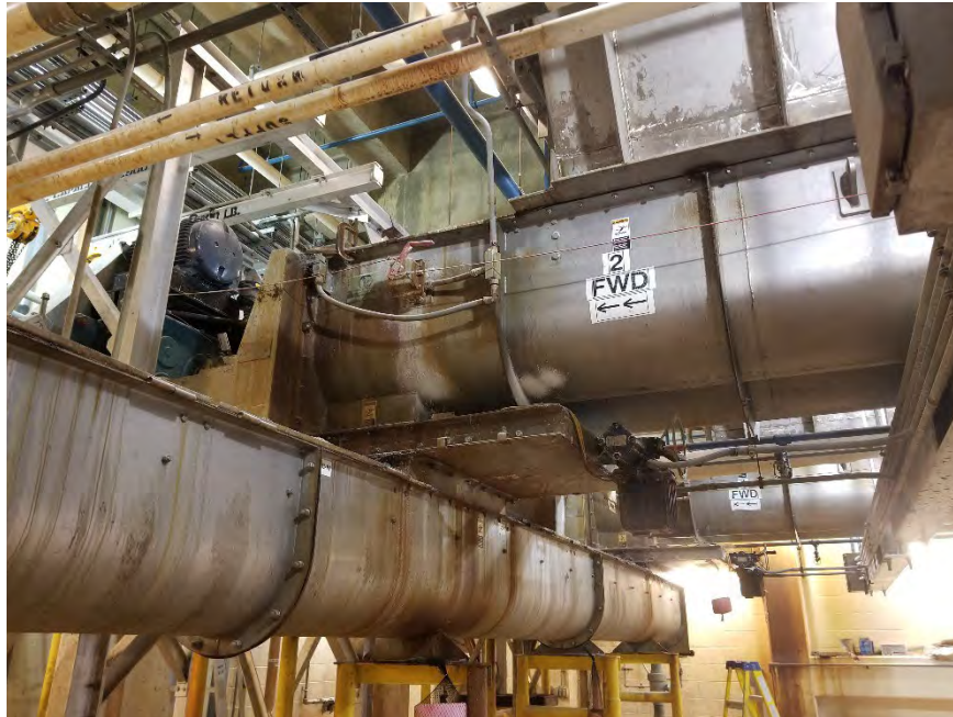
Figure 14. Second-floor Screw Conveyors
