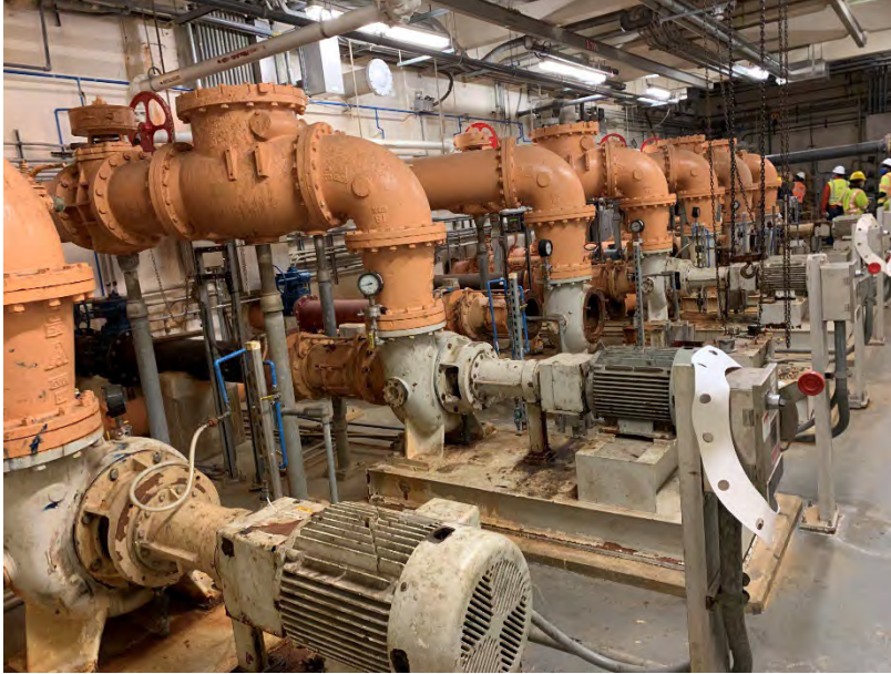
Figure 3. Side View of WAS Pumps
