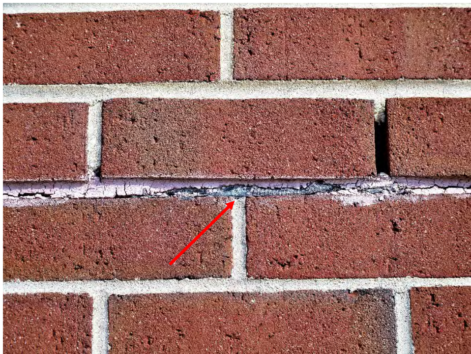
Photo A-47. Unusual Detailing
