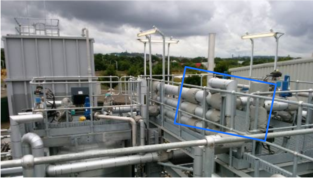
Figure 9-1. Process Gas Cooler
