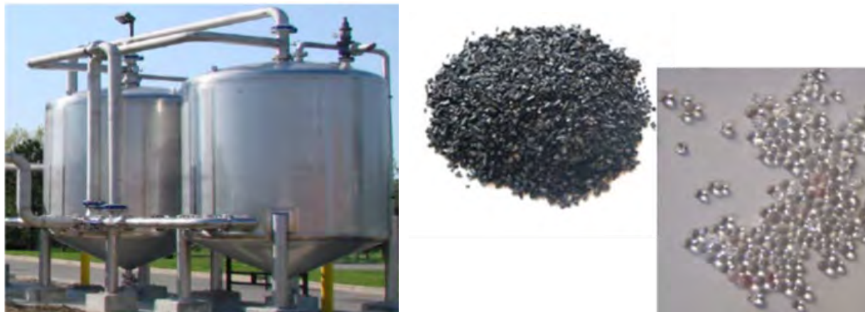
Figure 3. Siloxane Removal Equipment and Media
