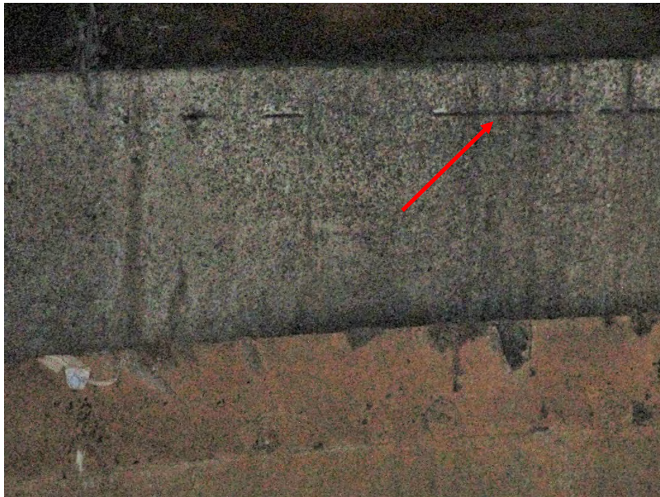
Photo A-6. Reinforcing Exposed
