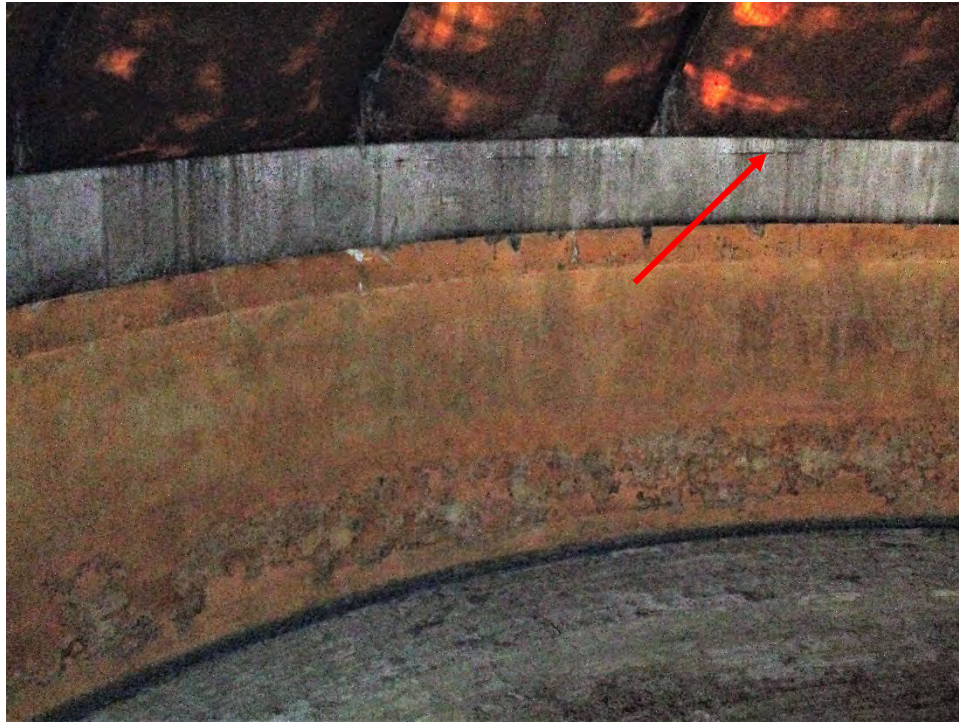
Photo A-5. Ferric Chloride Stain, Rebar Exposed
