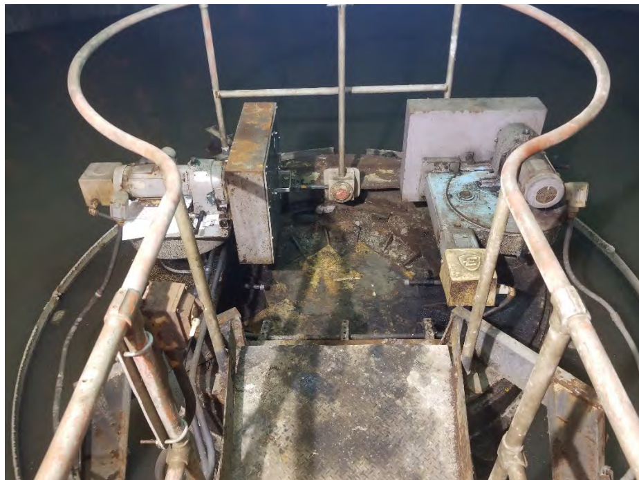
Figure 7. Gravity Thickener Center Platform
