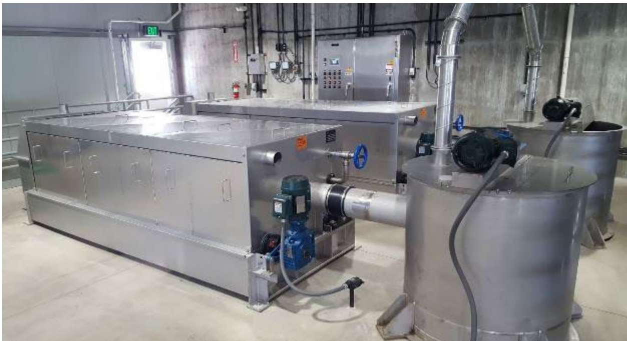
Figure 5-1. RDT and Flocc Tank
