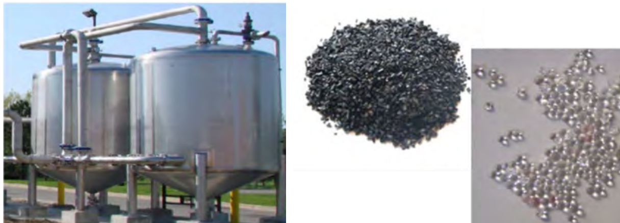
Figure 3. Siloxane Removal Equipment and Media
