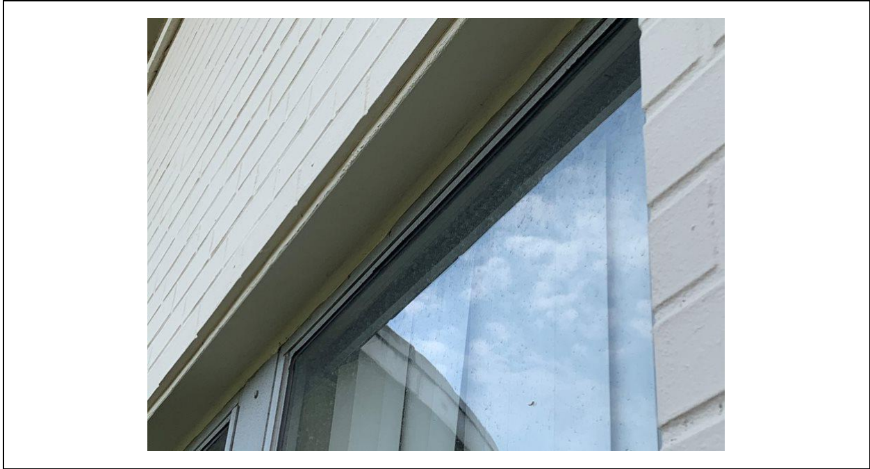
Lead-Containing Paint on the white metal window lintel at the building front entrance.
