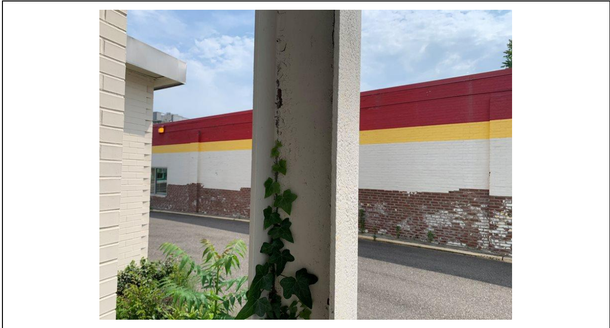
Lead-Containing Paint on the cream metal I-beam at the building rear and front entrance.
