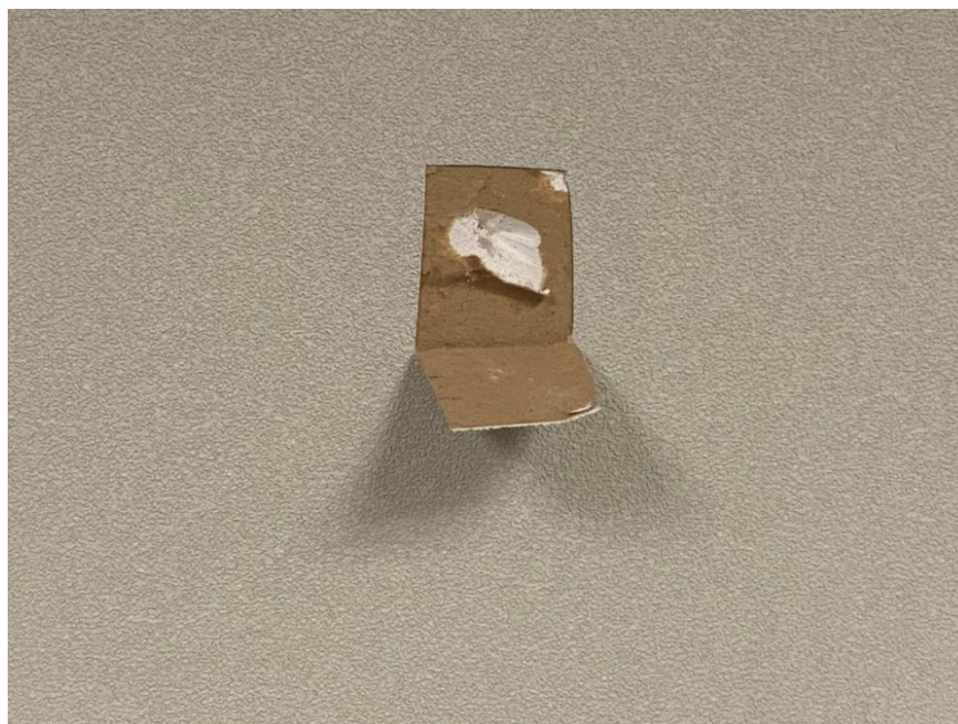
Homogeneous Material No. 17 – Non-ACM White Drywall with Associated White Joint Compound located in the Building Main Floor, 2 nd Floor and 3 rd Floor of the Subject Property
