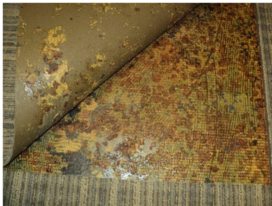
Homogeneous Material No. 16 – Non-ACM Brown/Tan/Black Floor Mastic located in the Building Main Floor, Main Customer Area of the Subject Property
