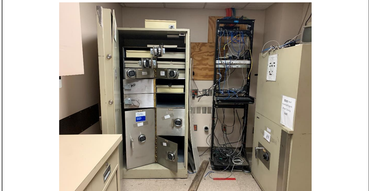
Wireless Control System components at the subject property building.
