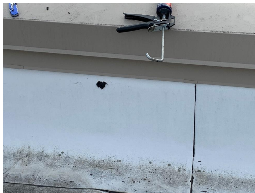
Homogeneous Material No. 2 – Non-ACM White/Black Curbing/Flashing located on the roof of the Subject Property
