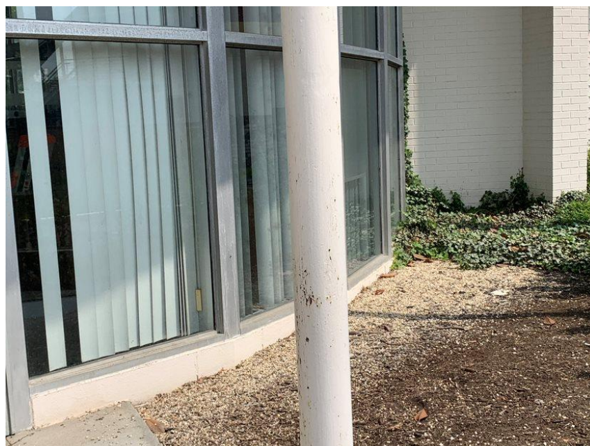
Lead-Containing Paint on the White metal column at the building rear and front entrance.
