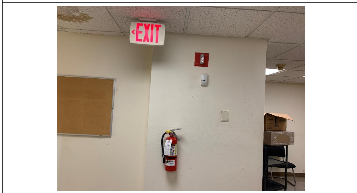
Typical Fire Extinguisher and Emergency Fire Strobe Lighting at the subject property building.
