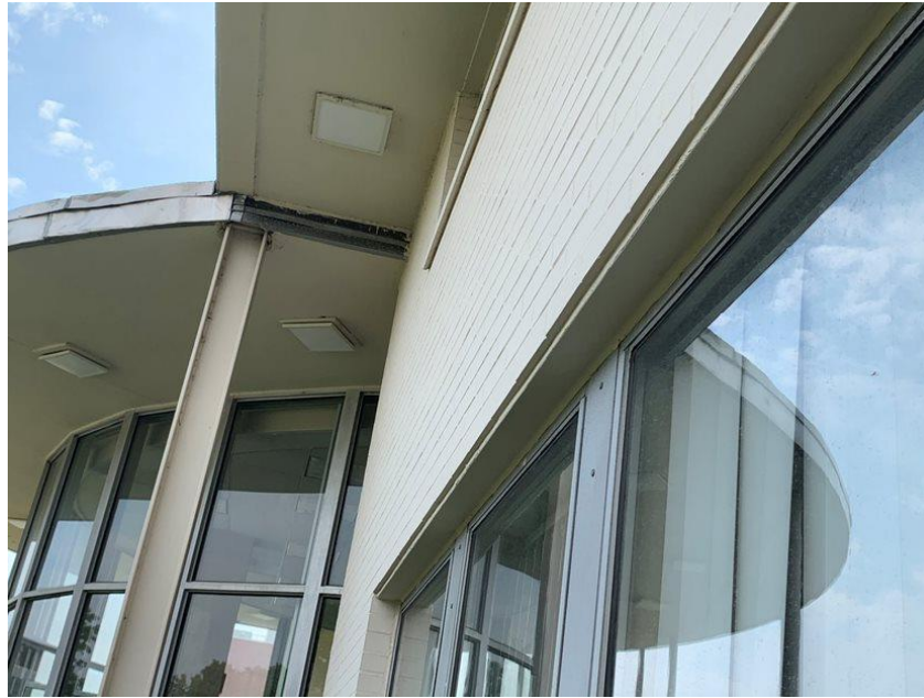
Lead-Containing Paint on the cream metal I-beam at the building front entrance.
