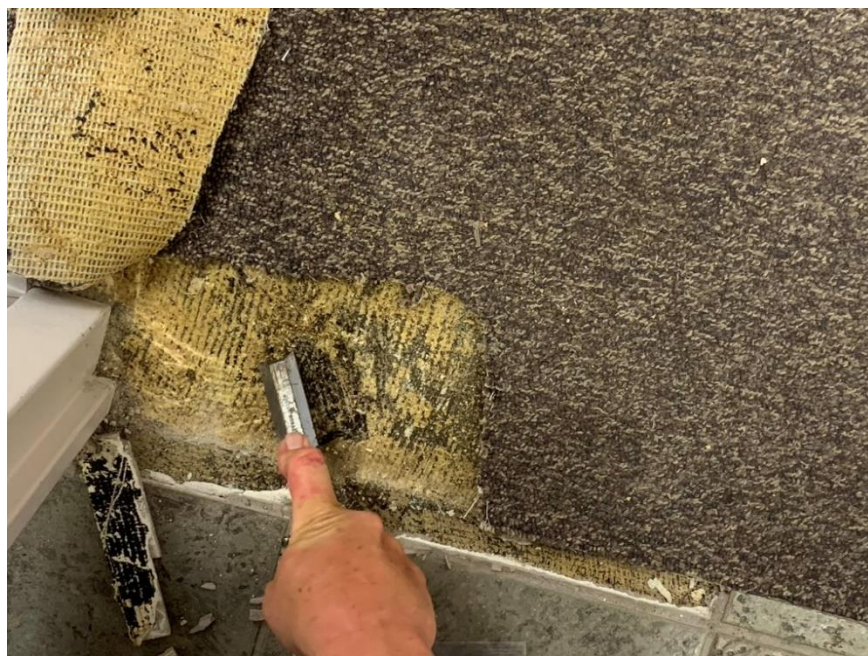
Homogeneous Material No. 21 – ACM Tan carpet glue with black mastic Located Throughout the offices on the Building 3 rd floor of the Subject Property
