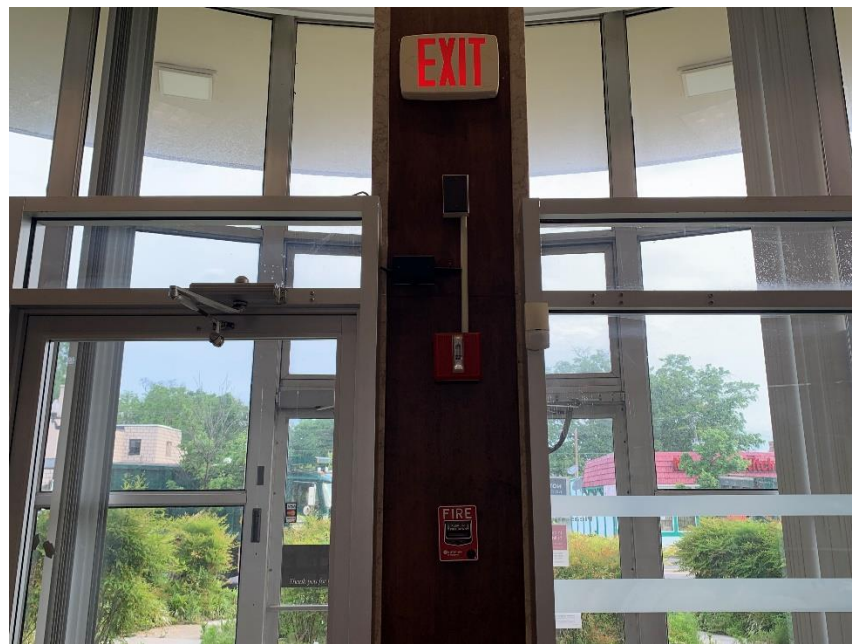
Typical Lighted Exit sign and Fire Emergency Pull-Down station at the subject property building.
