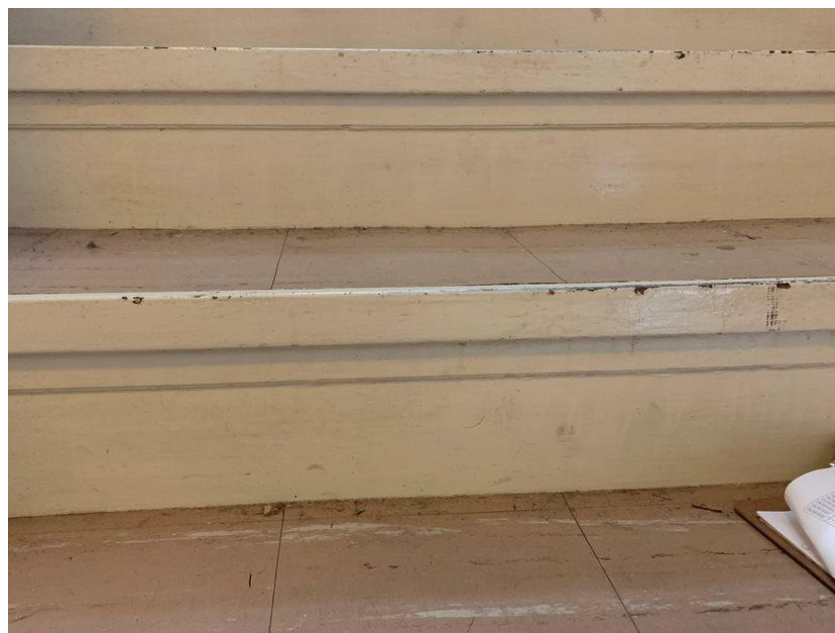
Lead-Containing Paint on the stairwell stair riser on the east side leading from the 1st floor to the 2nd floor.
