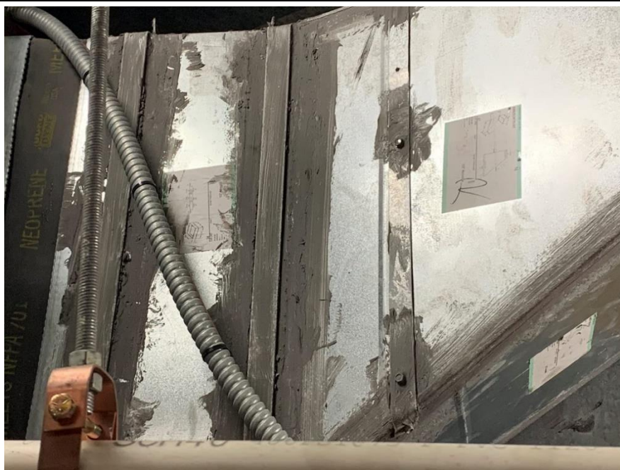
Homogeneous Material No. 8 – Non-ACM Gray HVAC Duct Seam Mastic located in the Building Basement, HVAC Room Number 1 and 2 of the Subject property
