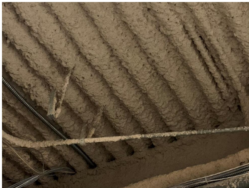
Homogeneous Material No. 5 – Non-ACM Gray Spray-on Fire Proofing located in the Building Basement Corridor, Electrical Room and Boiler Room of the Subject Property
