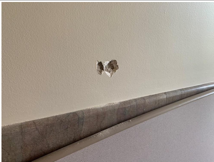
Homogeneous Material No. 11 – Non-ACM Plaster Gray Base White Skim Coat on Wall located in Building Main Floor, Corridor near Elevator of the Subject Property
