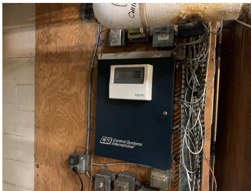
Fire Control Panel at the subject property building.
