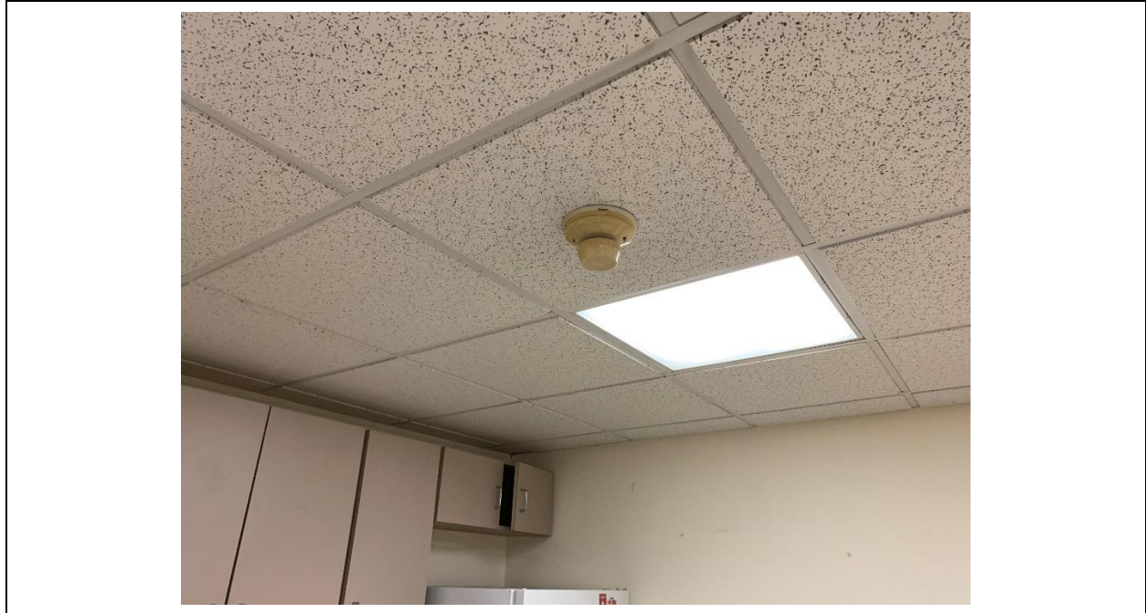
Typical Ceiling-Mounted Smoke Detector at the subject property building.
