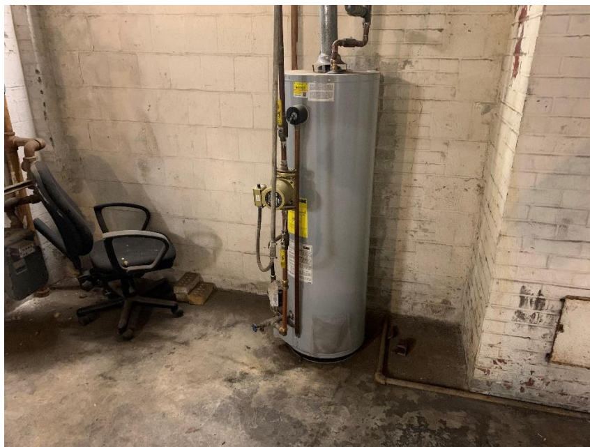
Domestic water heater (boiler) in the basement of the subject property building.
