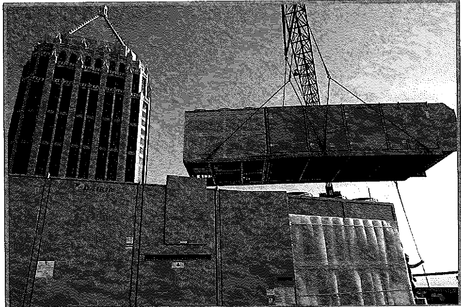
Bracken Building Low Roof HVAC
