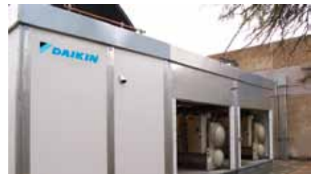
MCP with Dual Chillers Inside
