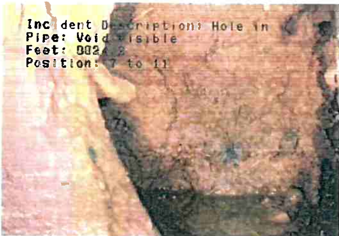
HVV - Hole in Pipe: Void Visible @ 24.2 ft.
