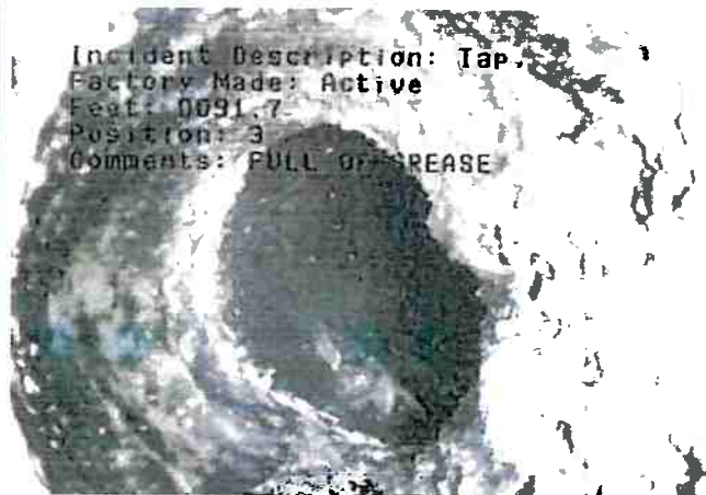
TFA - Tap, Factory Made: Active @ 91.7 ft. FULL OF GREASE
