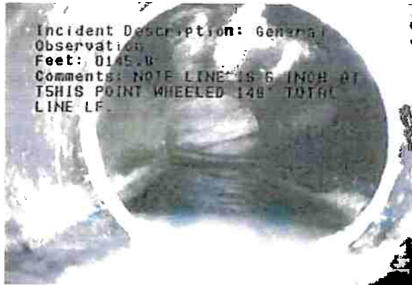
MGO - General Observation @ 145.0 ft. NOTE LINE IS 6 INCH AT THIS POINT WHEELED 148' TOTAL LINE LF.
