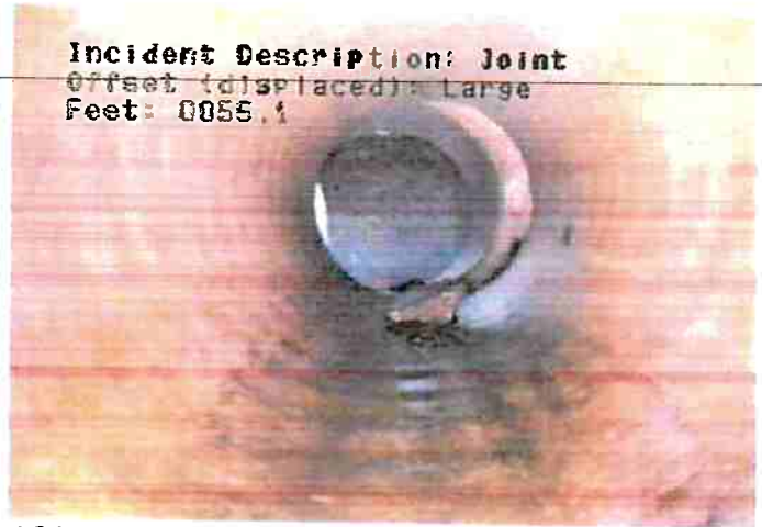
JOL - Joint Offset (displaced): Large @ 55.1 ft.
