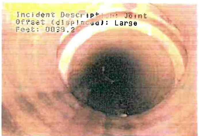
JOL - Joint Offset (displaced): Large @ 39.2 ft.
