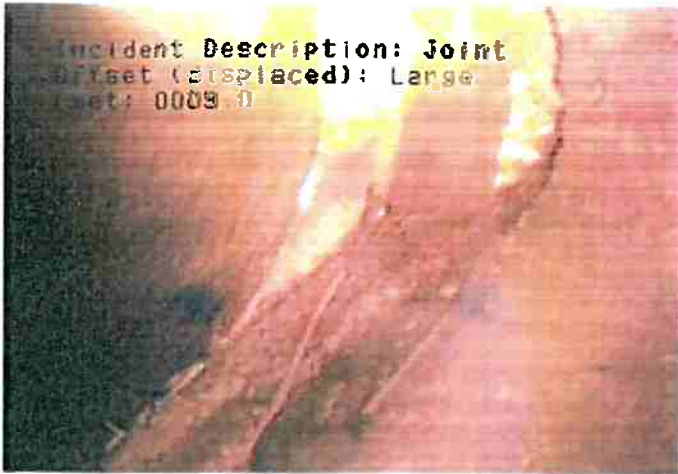
JOL - Joint Offset (displaced): Large @ 9.0 ft.
