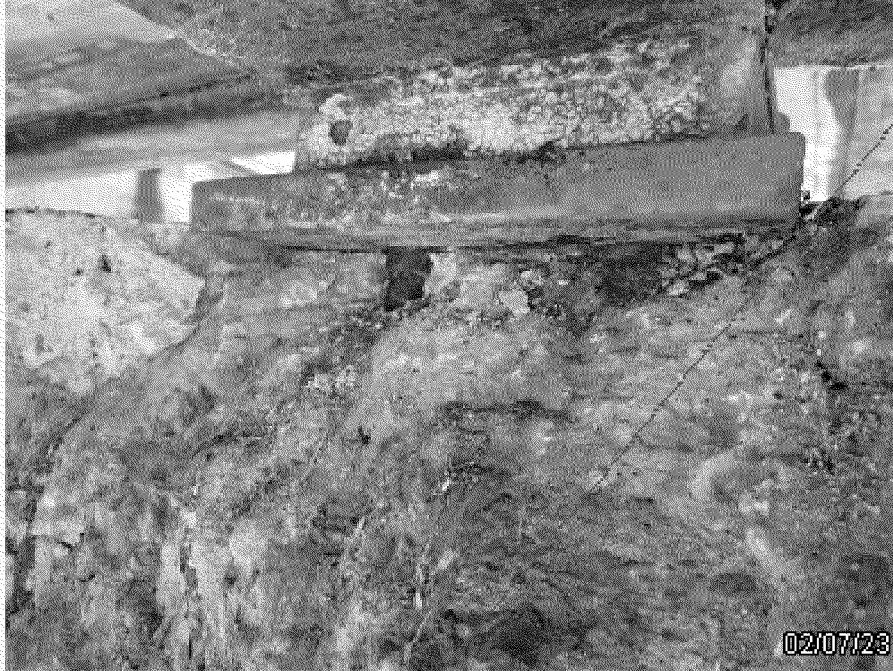
Photo 5: Loss of bearing at Bearing 19-3 at Bent 19
