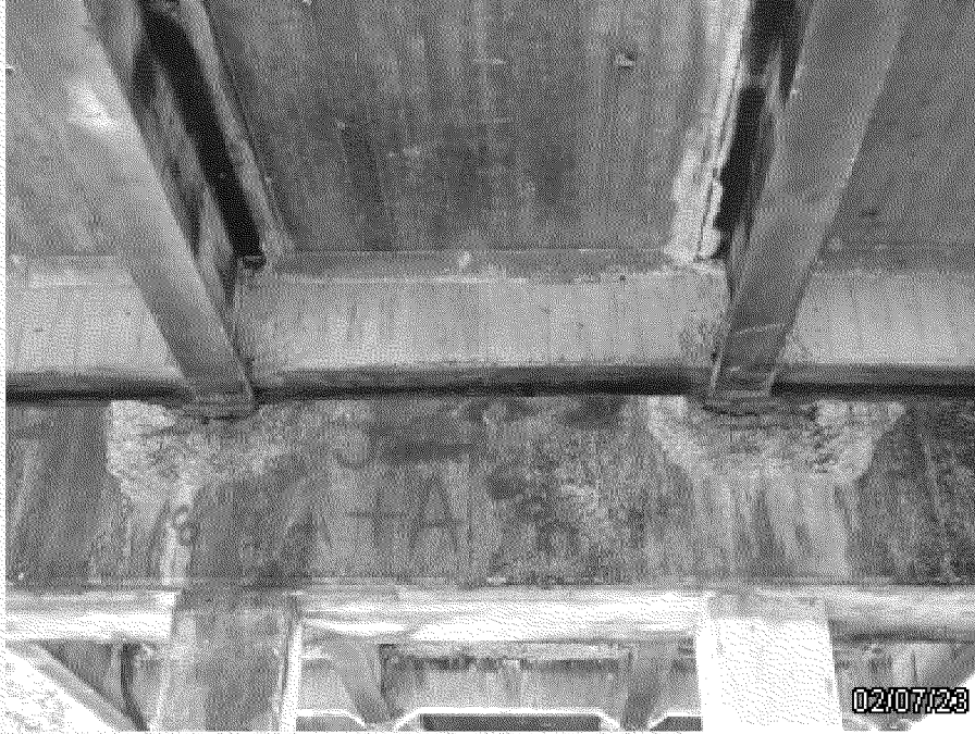
Photo 1: Spalls in Bent Cap 19 causing loss of bearing at near end of Beams 19-2 and 19-3
