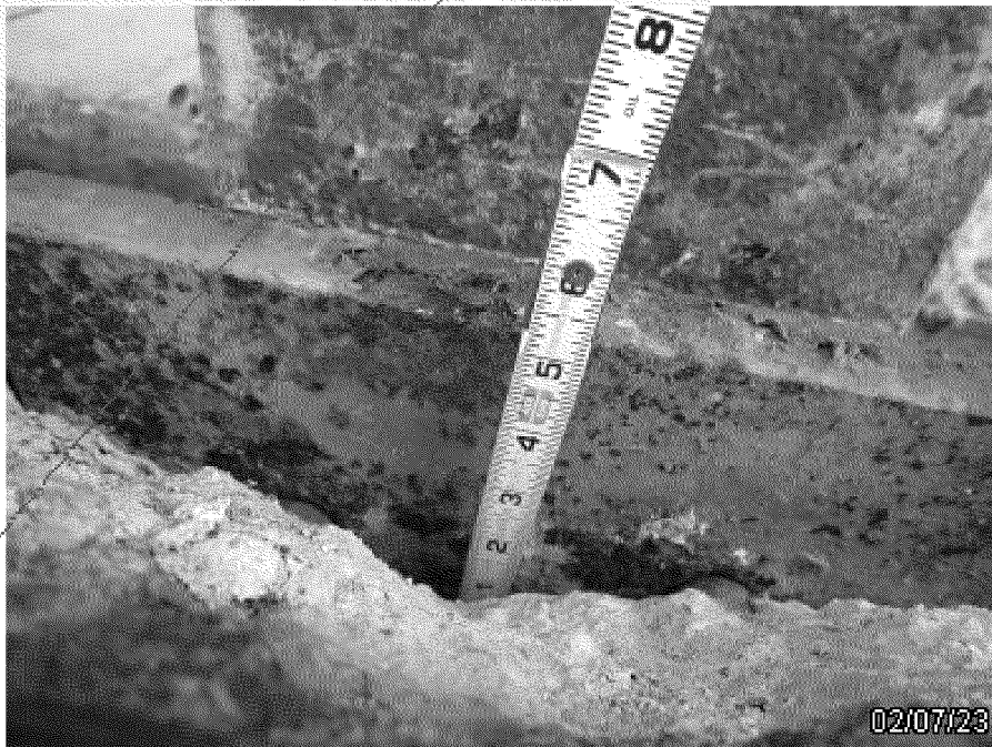
Photo 2: Loss of bearing at Bearing 19-2 at Bent 19
