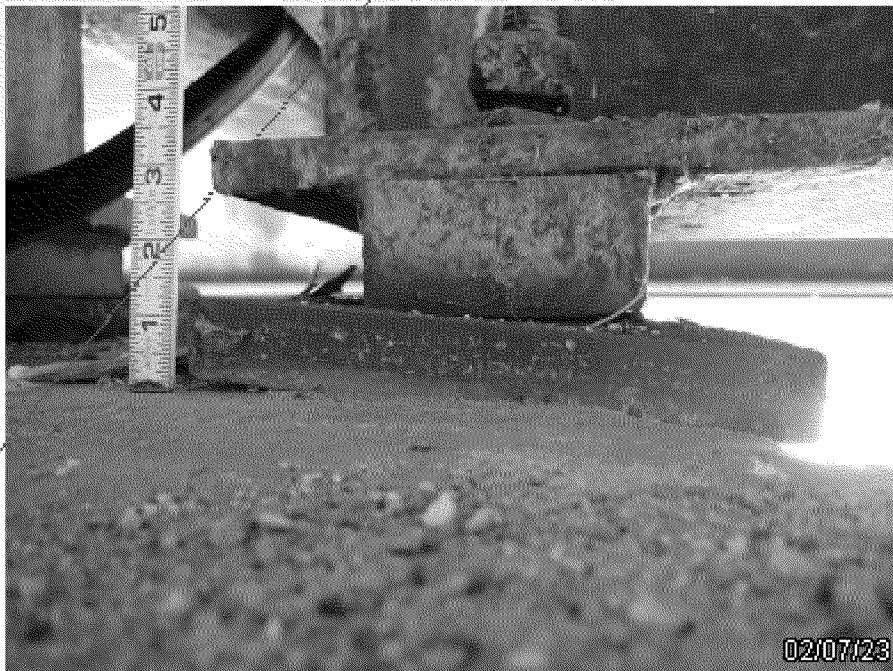
Photo 6: Bearing 19-2 tilting towards the far side causing a gap along near side
