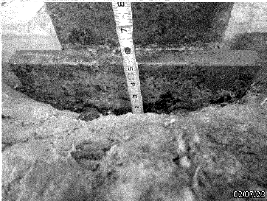
Photo 4: Loss of bearing at Bearing 19-3 at Bent 19
