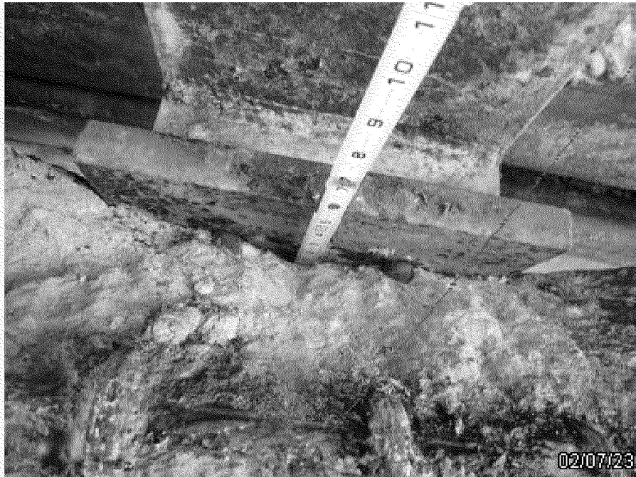
Photo 3: Loss of bearing at Bearing 19-2 at Bent 19
