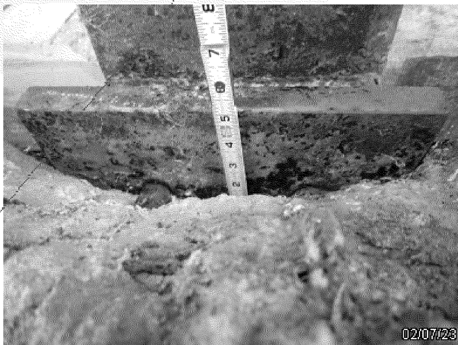
Photo 4: Loss of bearing at Bearing 19-3 at Bent 19
