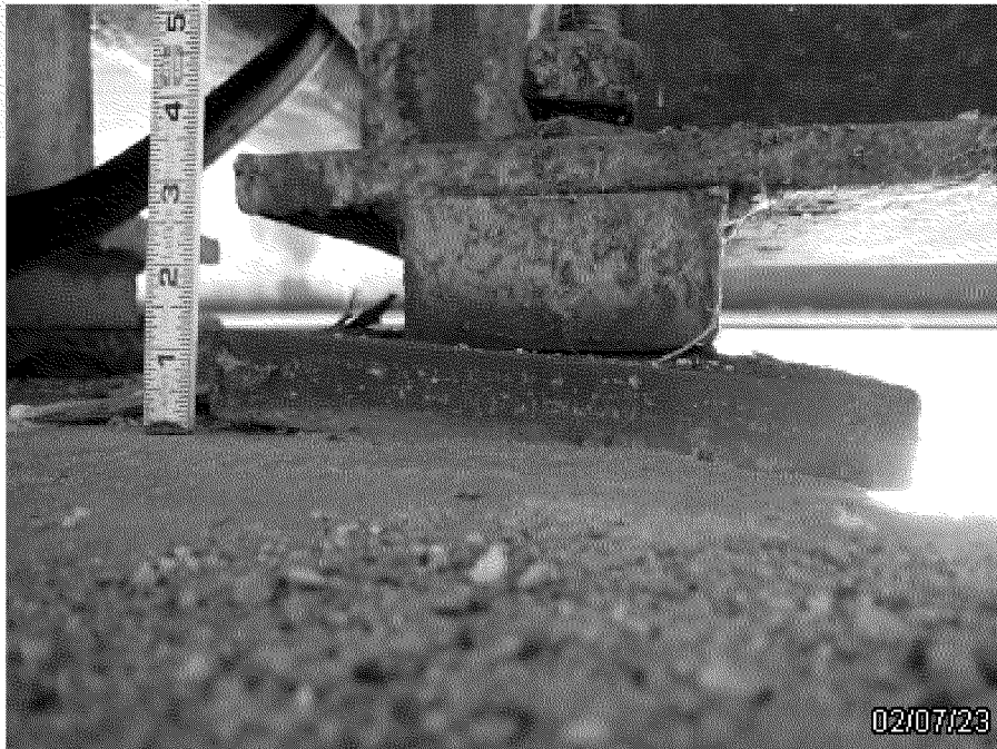
Photo 6: Bearing 19-2 tilting towards the far side causing a gap along near side
