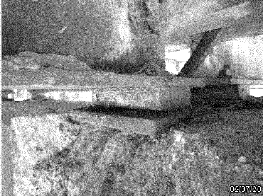
Photo 7: Bearing 19-3 tilting towards the far side causing a gap along near side
