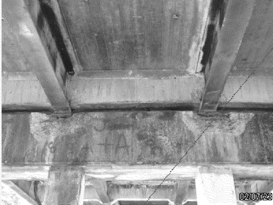
Photo 1: Spalls in Bent Cap 19 causing loss of bearing at near end of Beams 19-2 and 19-3
