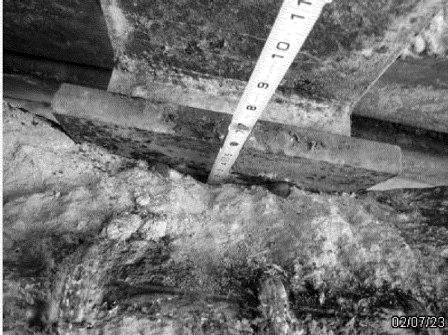
Photo 3: Loss of bearing at Bearing 19-2 at Bent 19
