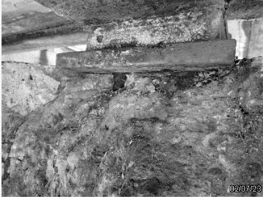
Photo 5: Loss of bearing at Bearing 19-3 at Bent 19
