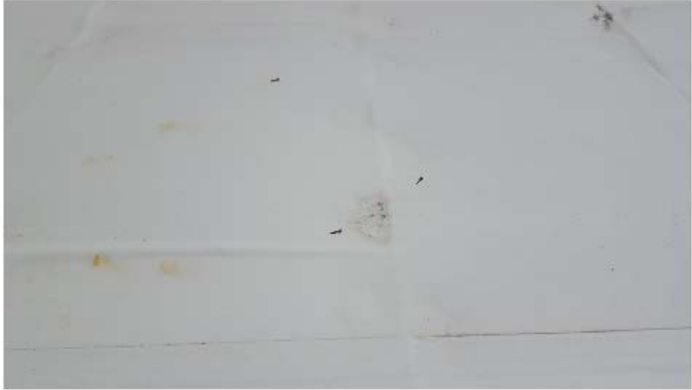
Loose screws/debris on roof
