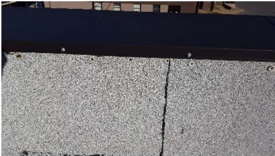
Exposed nails at wall flashing
