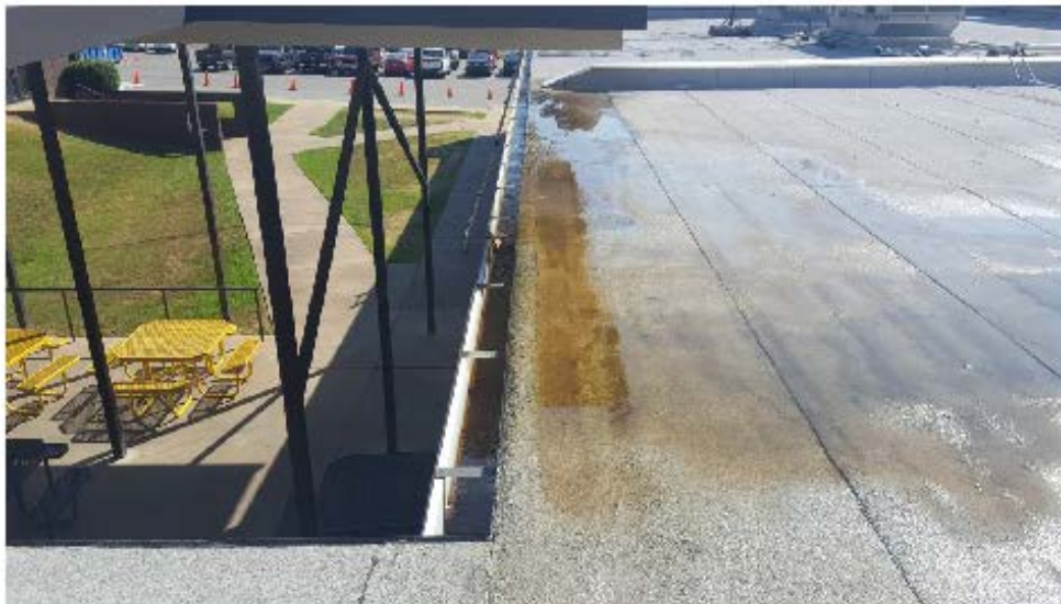
Ponding water resulting from leaking pipe
