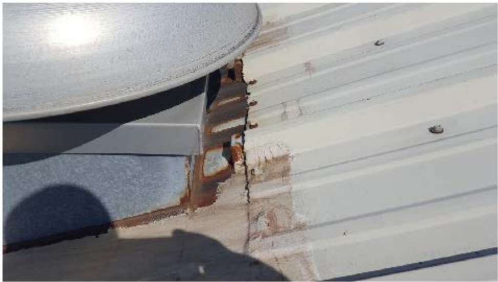
Rusted curb flange; rusted fasteners
