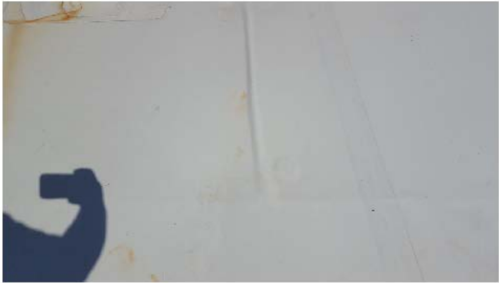
Ridging in membrane caused by loose insulation
