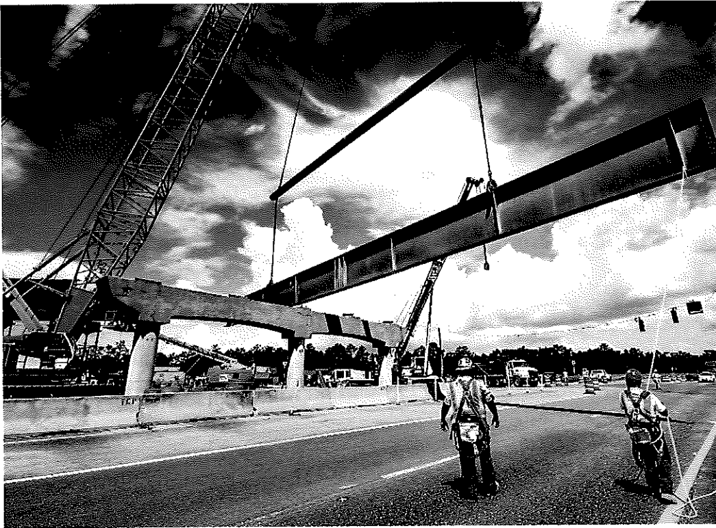
CEI services were provided for a new flyover bridge at the intersection of SR 123 and SR 85 to relieve traffic congestion in Okaloosa County. The project won the Outstanding Project Award by FICE/FDOT.
