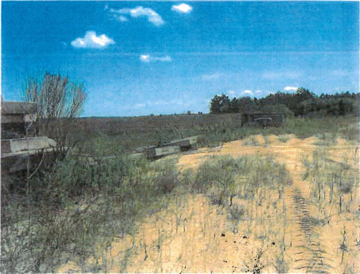
Photo #4 (C-72) Concrete Material
