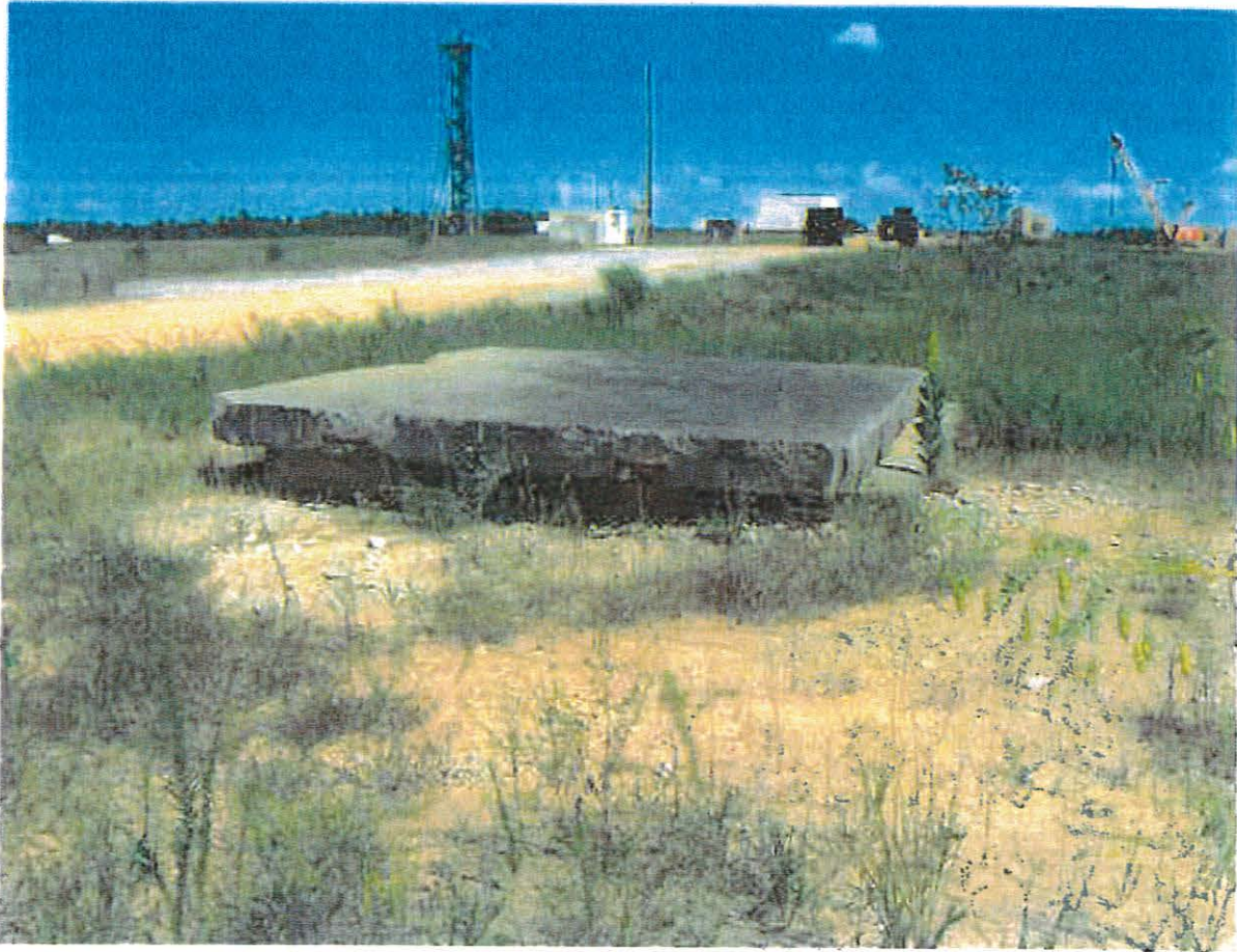
Photo #2 (C-74) Concrete Material
