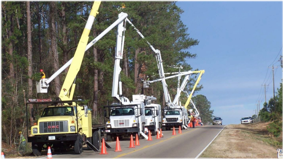
Hazard Tree Removal (Leaner)
