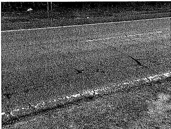
Alligator cracking on roadway
